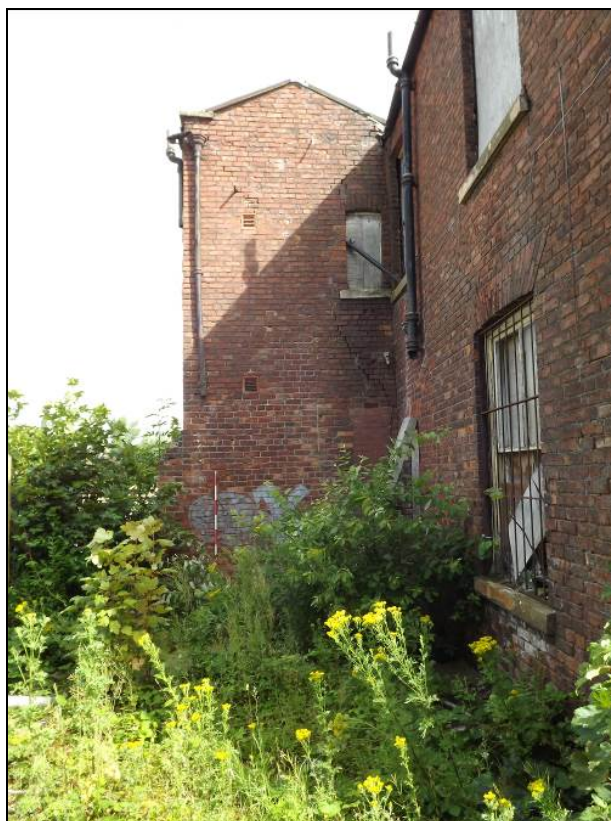
Plate 26: South facing elevation of addition showing blocked ground floor window and first floor window
