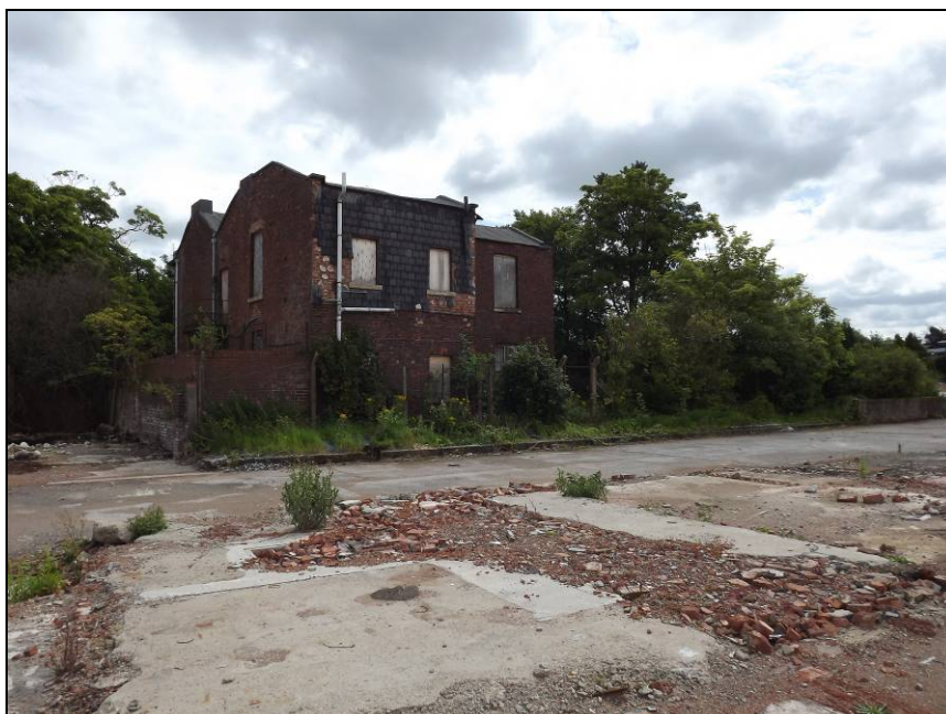
Plate 2: View looking east showing the north and west elevations of Bramhall House
