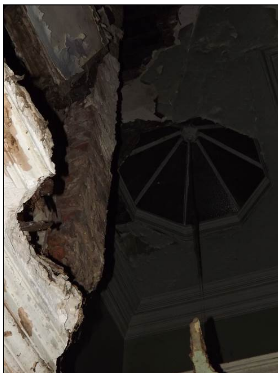
Plate 34: View of a hexagonal roof light which would have lit the first floor landing
