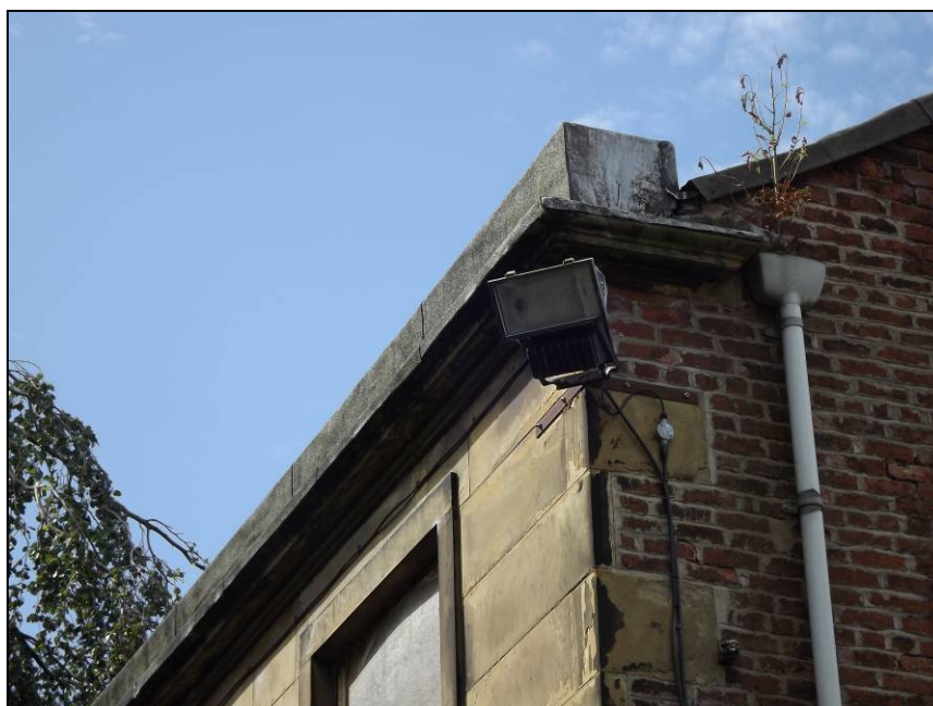
Plate 10: Detail of cornice and line of stone blocks along the top of the east elevation
