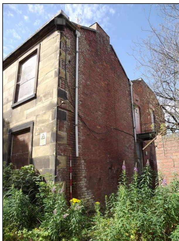
Plate 16: Detail of ashlar quoins of the east elevation and the brickwork of the north elevation
