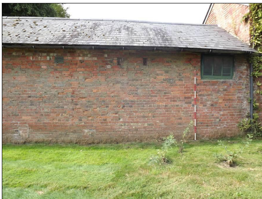
Plate 23: North elevation, west end, showing single window which lights the Tack Room (Scale = 2m)
