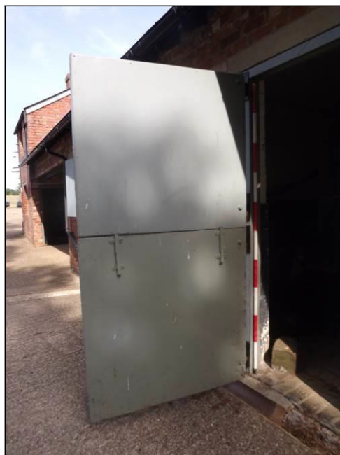
Plate 15: Detail of the internal side of one of the doors showing the metal sheeting
