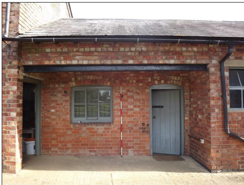
Plate 10: South elevation showing set back doorway and window for the Tack Room (Scale = 2m)
