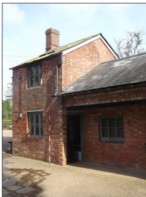
Plate 5: Detail of two-storey section with scarring for a former flue visible above the roof of the lower section
