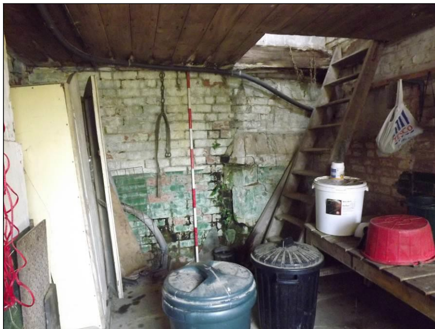
Plate 26: North wall of ground floor Store showing wooden staircase and projecting section of earlier garden wall
