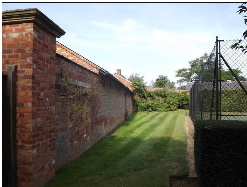
Plate 19: View looking west along the north elevation of the Loosebox Range, with the tennis court to right of photograph
