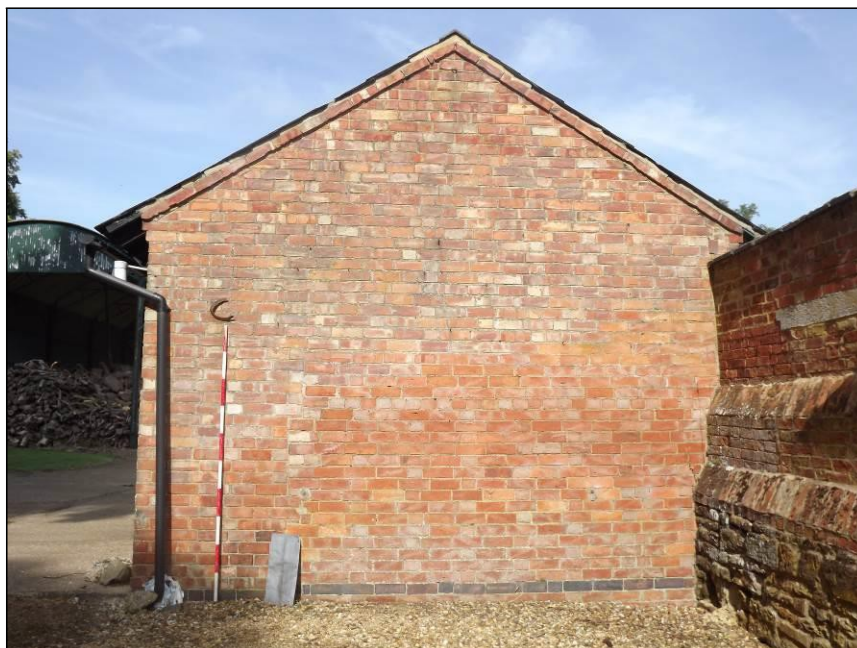
Plate 16: East elevation showing the band of blue brick near ground level (Scale = 2m)
