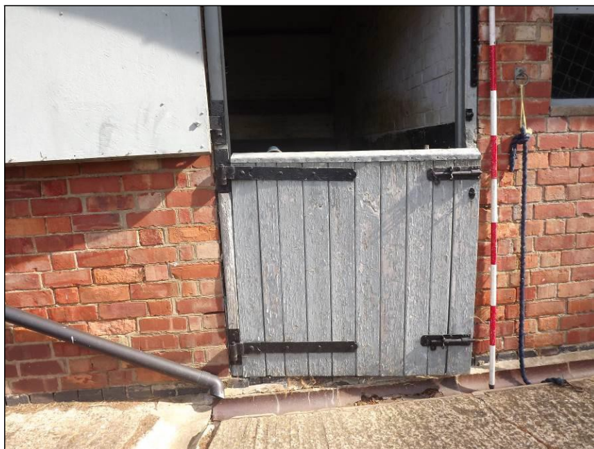
Plate 14: Detail of one of the loose box doors showing the external hinges and bolts, south elevation
