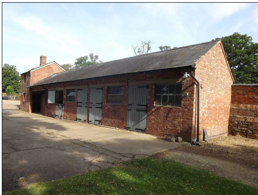
Plate 12: South elevation showing the doorways and windows of the four loose boxes
