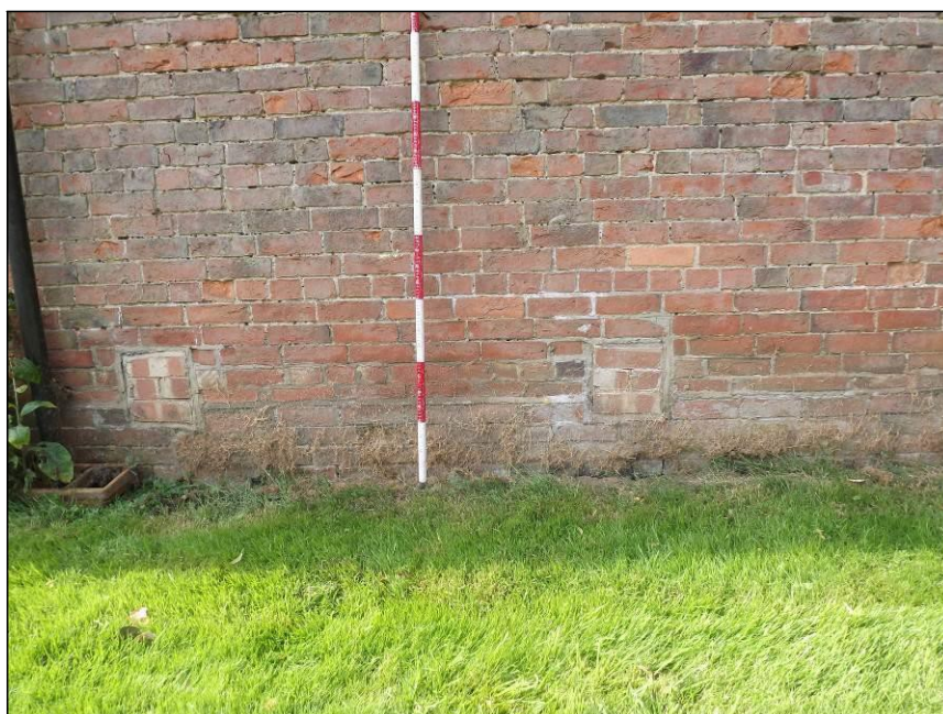
Plate 21: Detail of English Garden Wall Bond brickwork and possible former ventilation holes, north elevation
