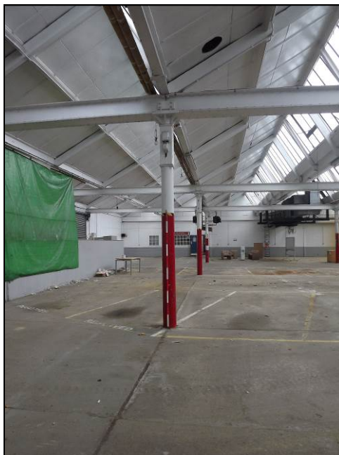
Plate 33: View looking north-west showing the round columns and I-beams of the roof structure, main former factory floor
