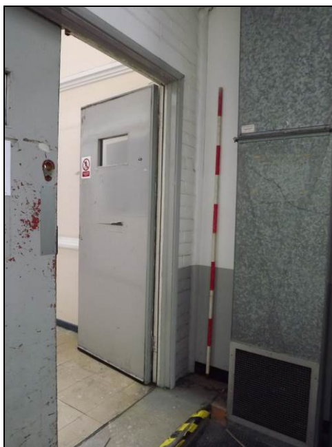
Plate 40: Double doorway at north end of the north-west wall of main former factory floor with column incorporated into the wall (Scale = 2m)
