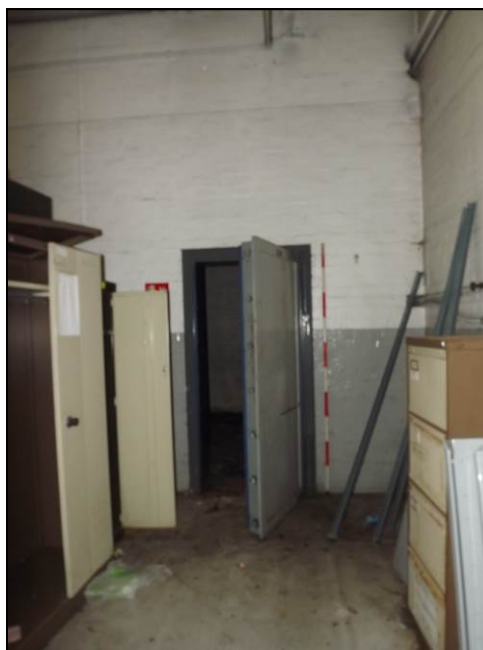
Plate 49: Small room at north-east end of c.1930 addition, possibly a former strong room (Scale = 2m)
