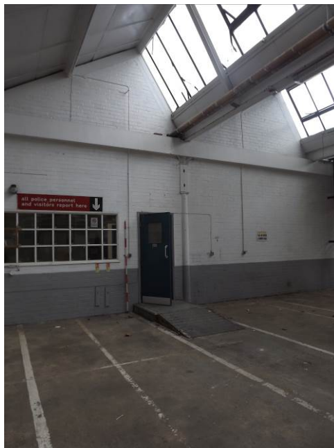
Plate 39: North-west wall (south end) of main former factory floor showing the possible inserted wall, window and doorway
