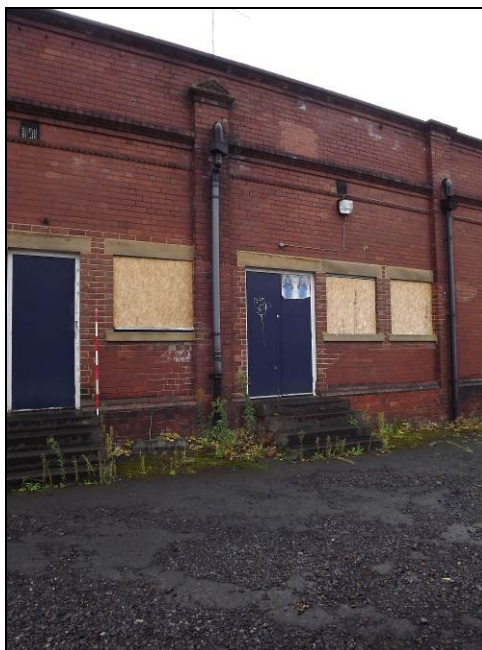
Plate 11: North-west elevation showing architectural detailing in the form of horizontal banding and vertical columns
