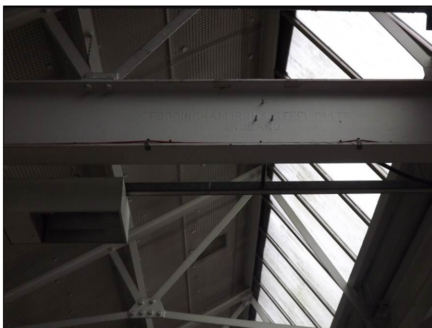
Plate 48: Detail of steel maker's mark 'Frodingham Iron and Steel Co Ltd', roof structure in c.1930 addition
