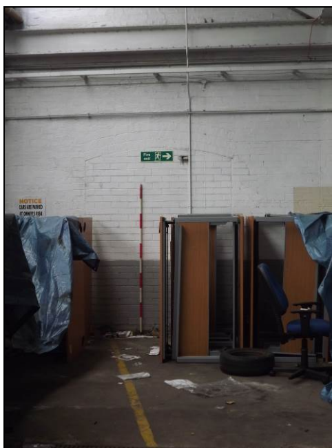
Plate 36: Original doorway in south-east wall of main former factory floor (Scale = 2m)
