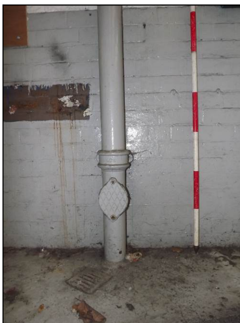
Plate 53: Detail of possible access hatch, downpipe on north-west wall of north-west of c.1930 addition
