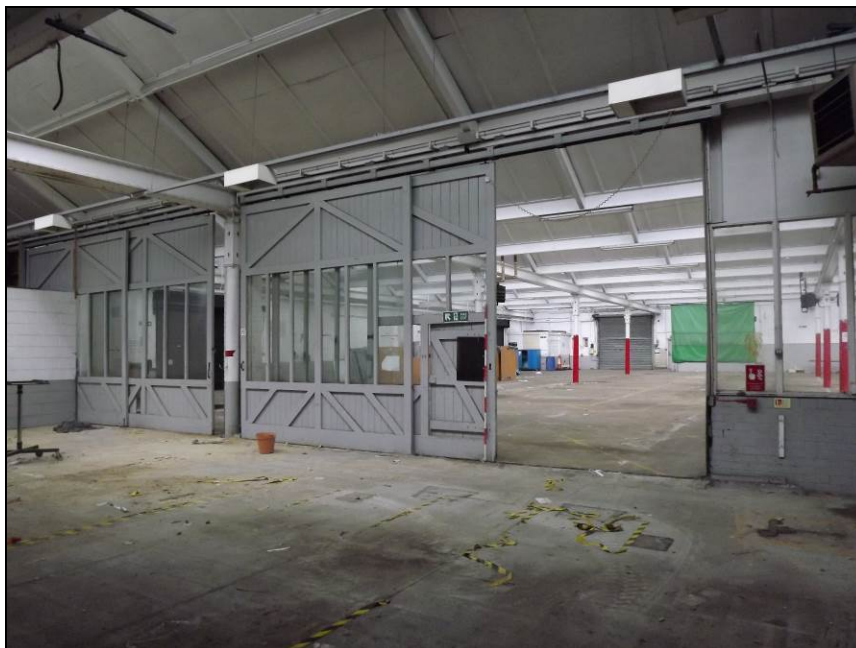
Plate 43: Northern side of sliding doors, located in the north-east wall of the main former factory floor (Scale = 2m)
