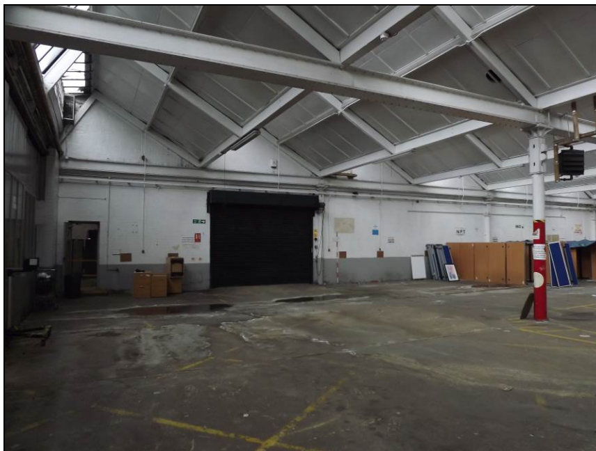
Plate 37: South-east wall of main former factory floor showing inserted doorways and incorporated columns
