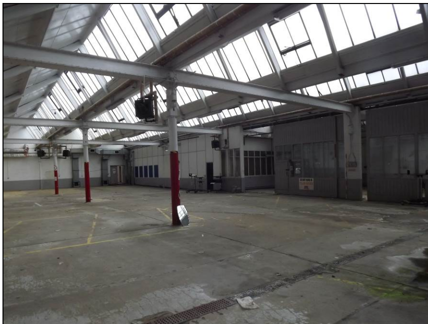
Plate 41: North-east wall of main former factory floor showing inserted sliding doors and stud walls
