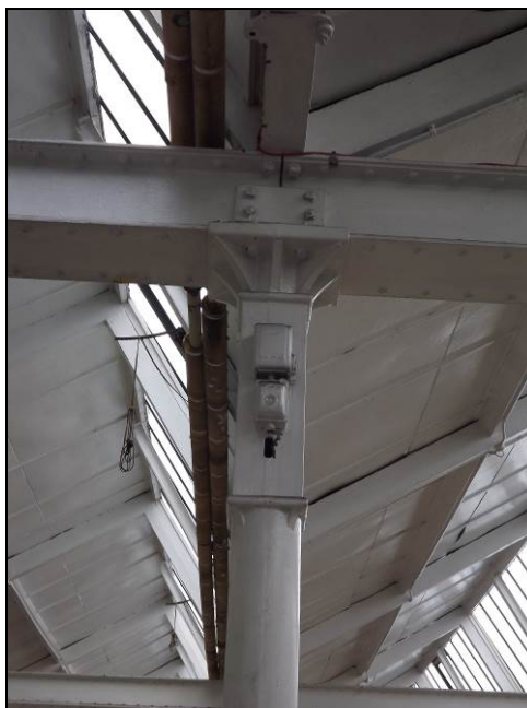
Plate 35: Detail of top of column showing joints between I-beams and electric fittings
