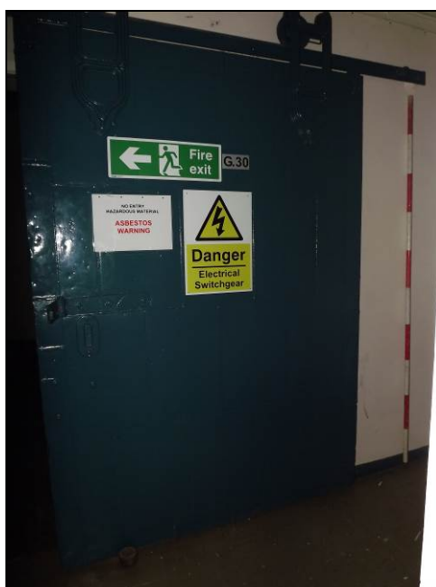
Plate 56: Room G30 (Electrical Switchgear)
