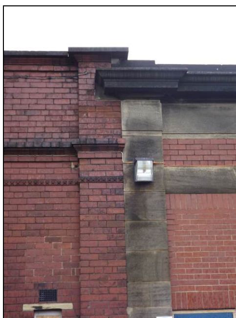
Plate 26: Construction break between original factory (left) and c.1930 addition (right), south-west elevation
