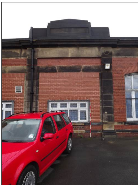
Plate 23: South-west elevation, c.1930 addition, showing the shadow of the company name 'ARTHUR AND COMPLY LTD'
