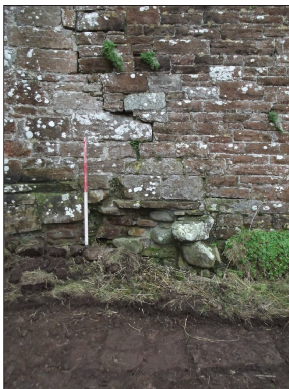
Plate 6: Curtain wall in the vicinity of the exposed stone slabs, facing north
