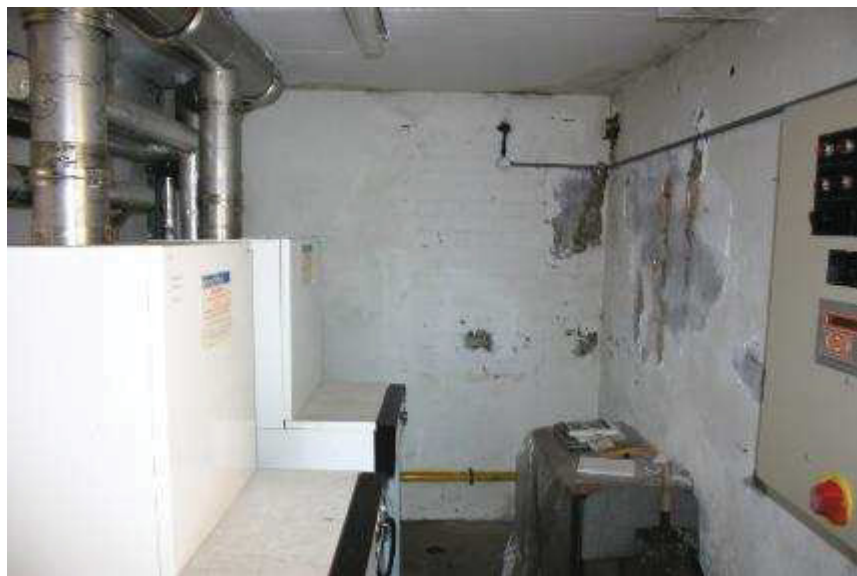
Plate 26: R 29, Boiler Room
