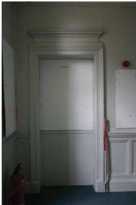
Plate 55: R 32, blocked doorway
