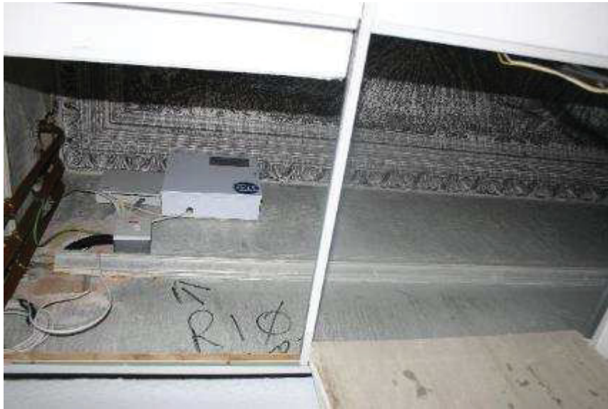
Plate 84: R 97, damaged coving/frieze above false ceiling
