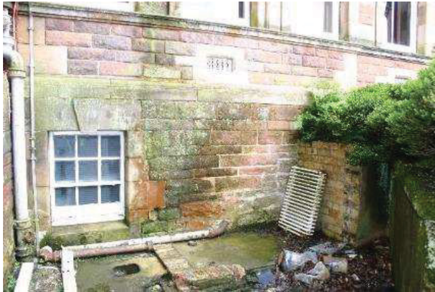
Plate 13: Lichen infestation Main Building
