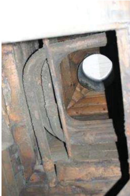
Plate 176: R 347, detail of water pipes in skylight lit service shaft
