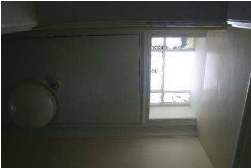
Plate 130: R 209, blocked skylight
