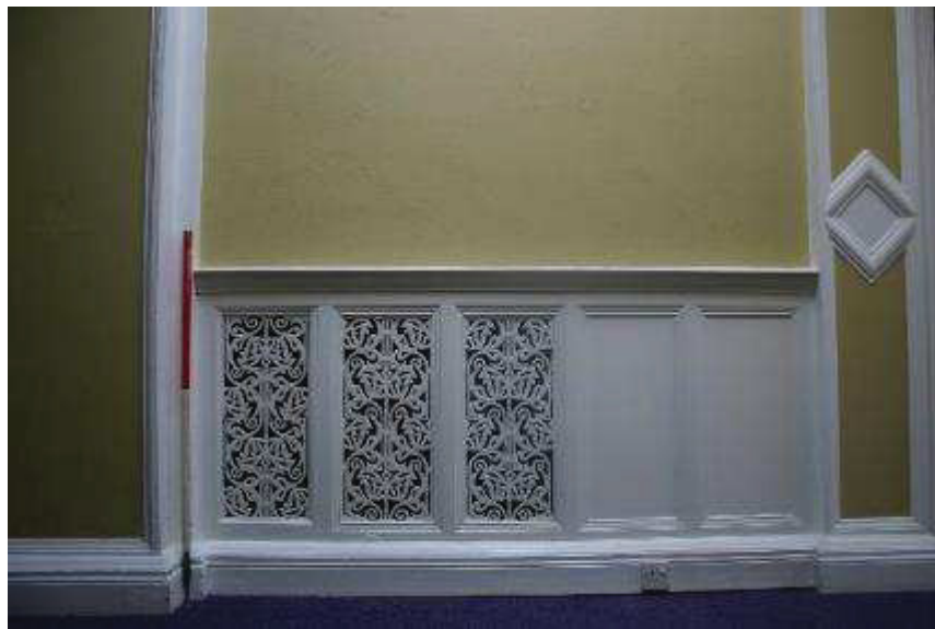
Plate 80: R 95, detail radiator air vent
