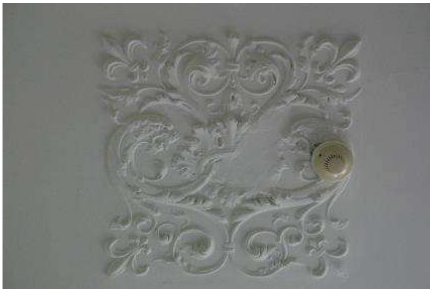
Plate 143: R 242, detail of damage to stucco decoration
