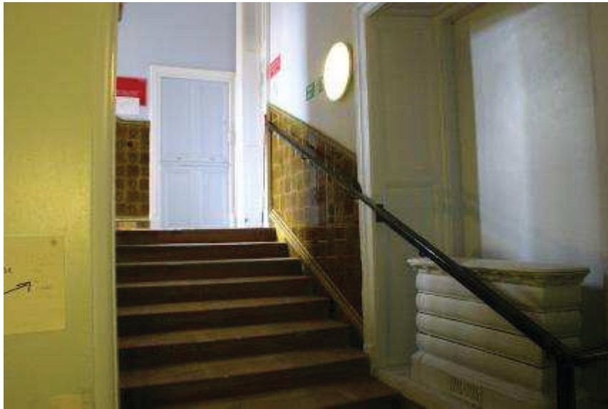
Plate 142: R 240, general view, with Victorian encased radiator
