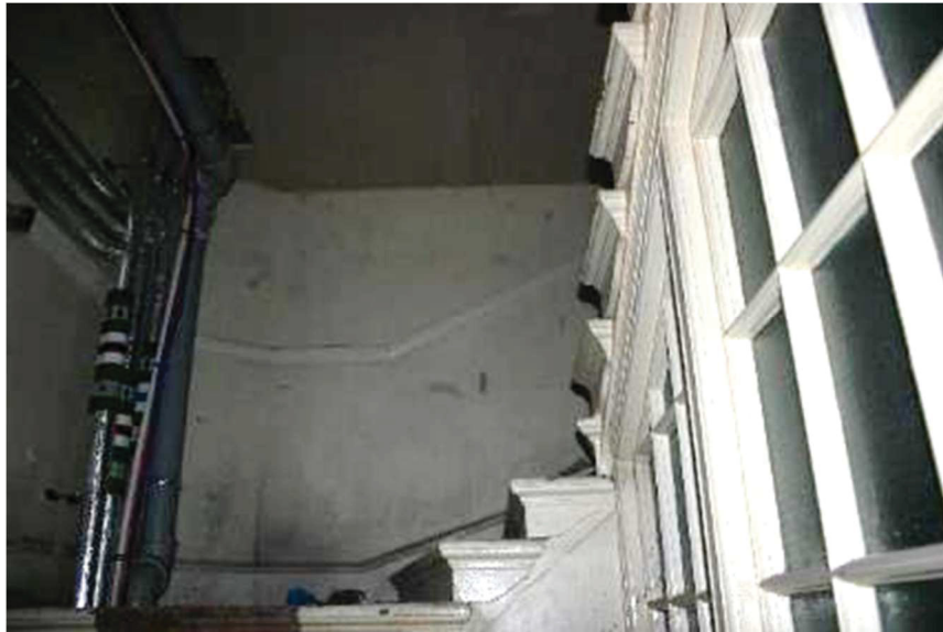
Plate 63: R 54, blocked staircase
