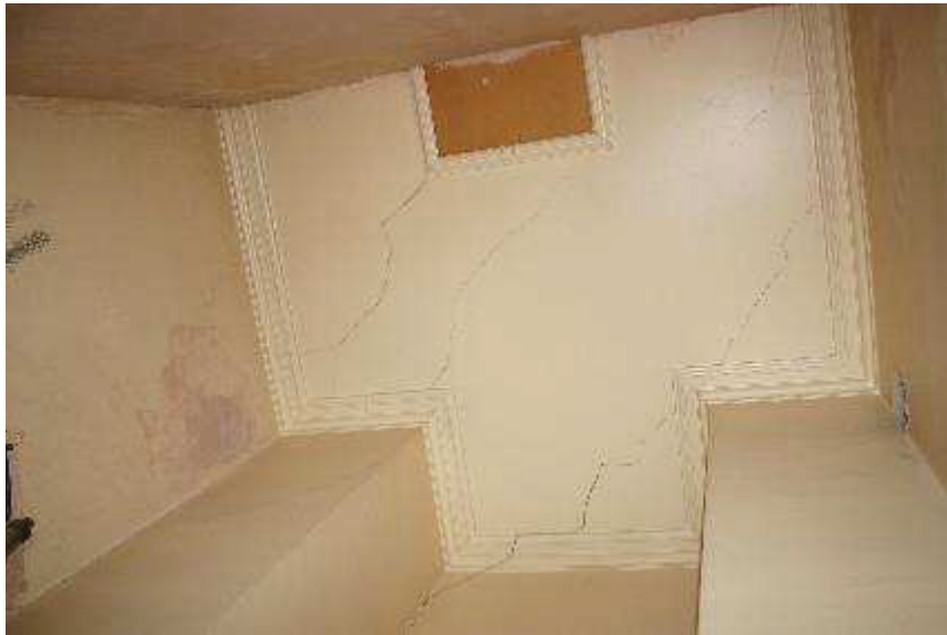
Plate 170: R 319, ceiling and blocked skylight
