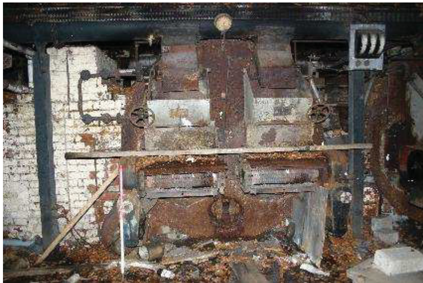
Plate 183: Engineers Pavilion, detail of boiler with coal hopper feeds
