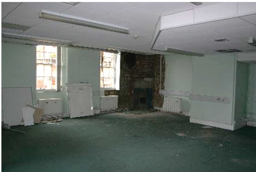
Plate 171: R 320, water damage in corner
