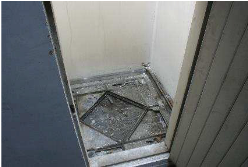
Plate 166: R 300, damaged skylight
