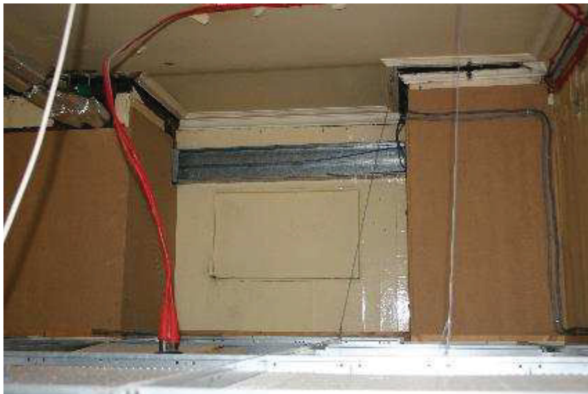
Plate 155: R269c, ceiling with blocked over door light
