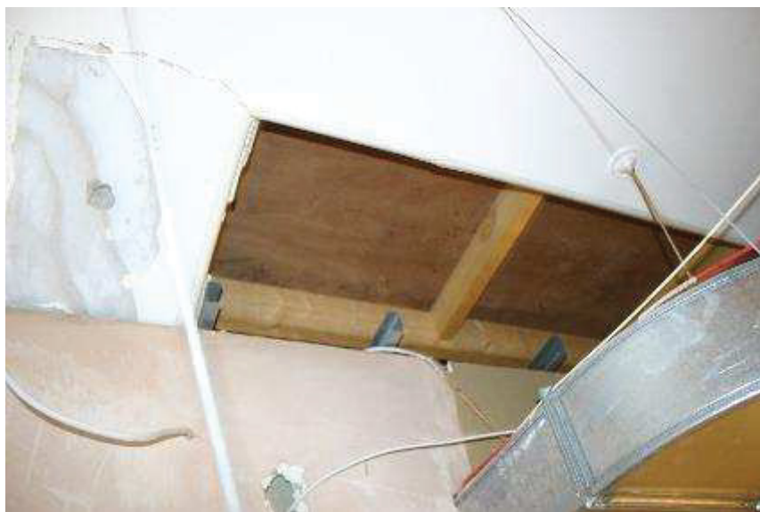
Plate 83: R 97, disabled toilet, blocked skylight
