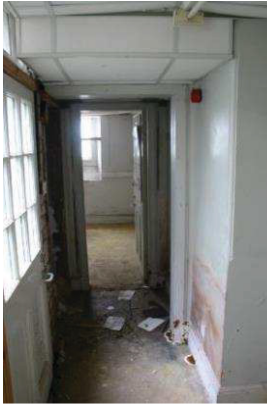
Plate 44: dry rot/fungus infestation in R 71
