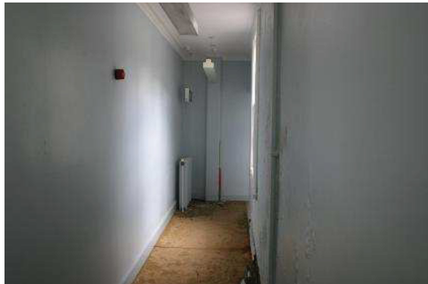
Plate 24: hallway 27, some water damage visible on the right
