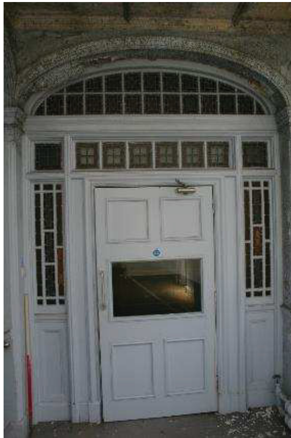
Plate 29: doorway with stained glass, heavy mould infestation R 36
