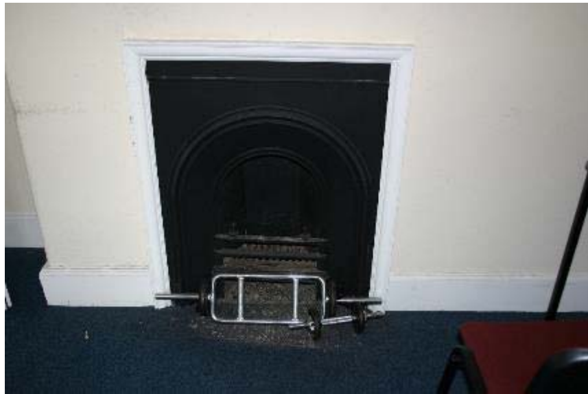
Plate 15: Cast iron fireplace R 4.
