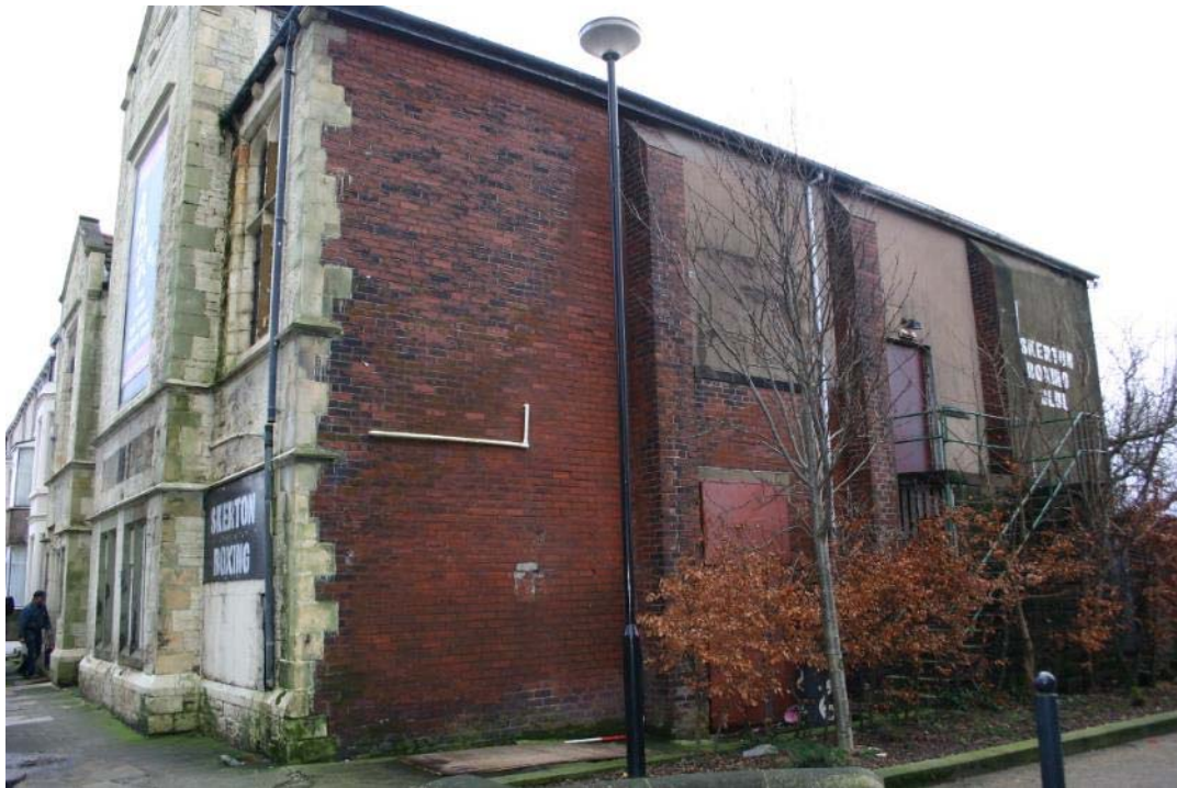
Plate 3: West Elevation, with modern fire escape
