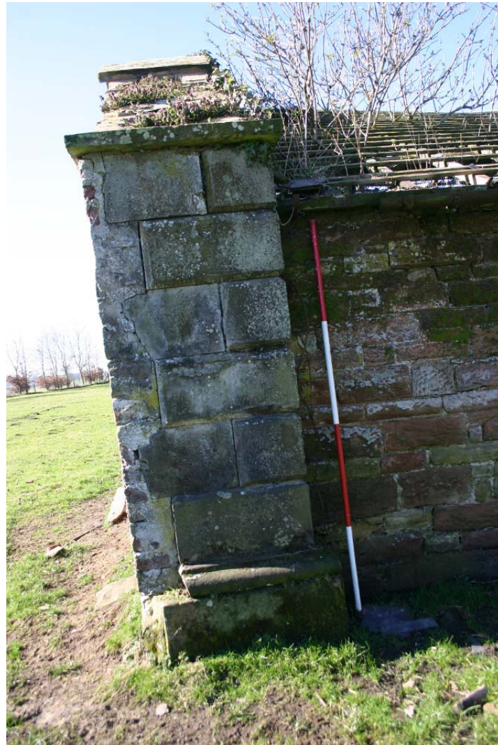
Plate 22: East corner of structure 2, brick walling set in front of sandstone ashlar masonry
