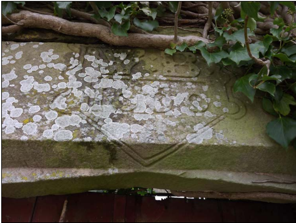
Plate 18: Initials and date 'W B 1660', on the lintel reused above a doorway in the south-west elevation of Crofton Hall Range, Photo: F.Wooler 2011
