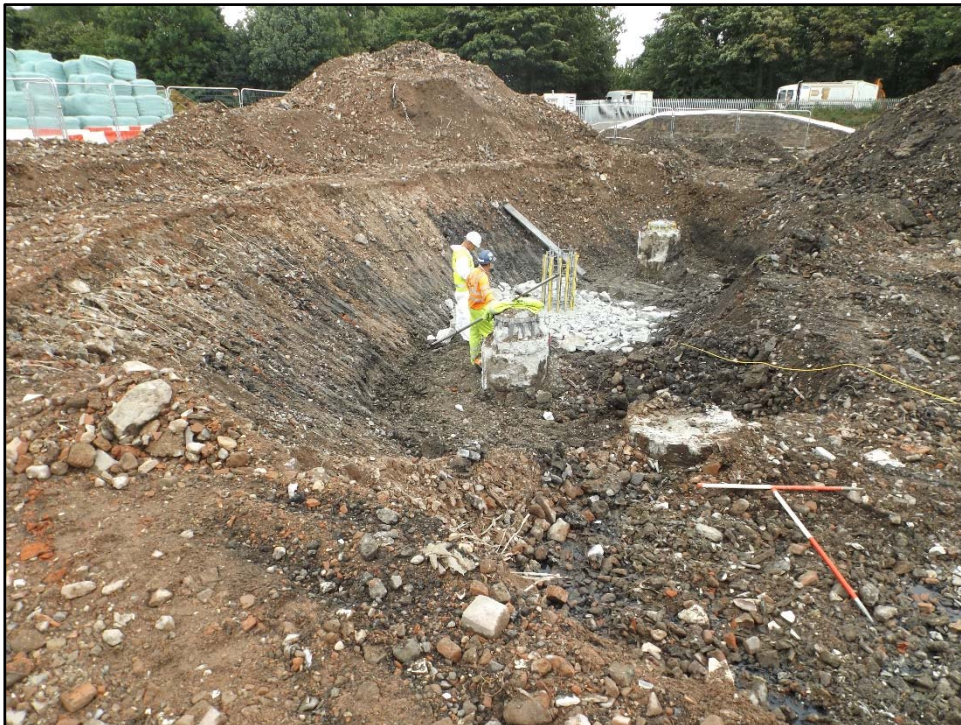
Plate 2: Excavations of Trench 2 showing made ground and the installation of pilings within the trench.
