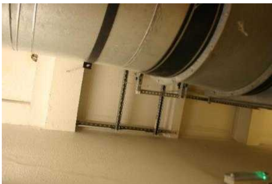
Plate 11: Lift Tower, fourth storey, remains of coving
