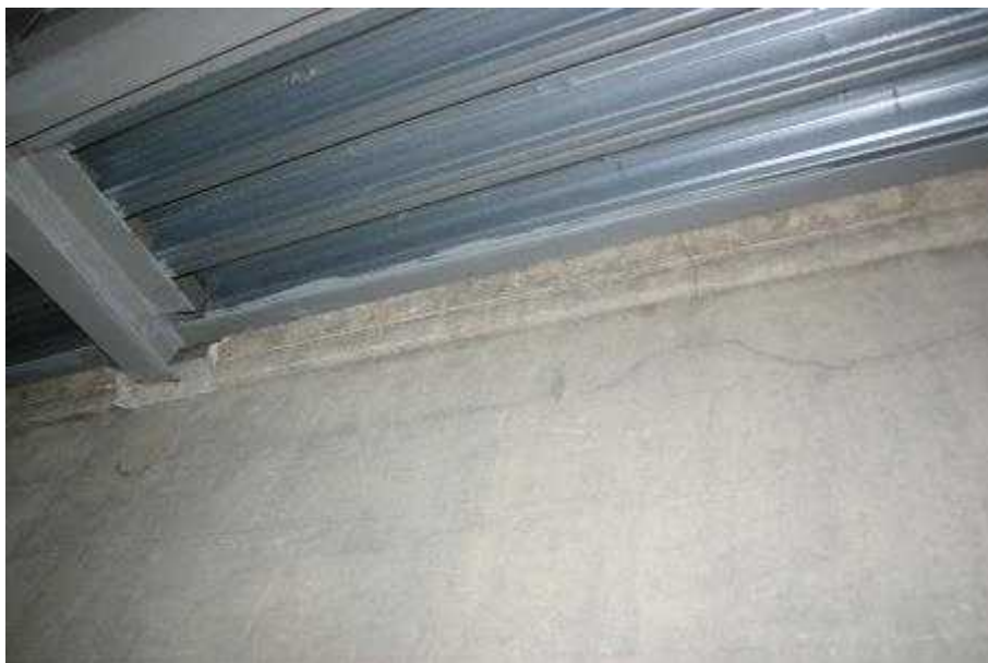
Plate 26: Unit 7, Coving at angled north elevation
