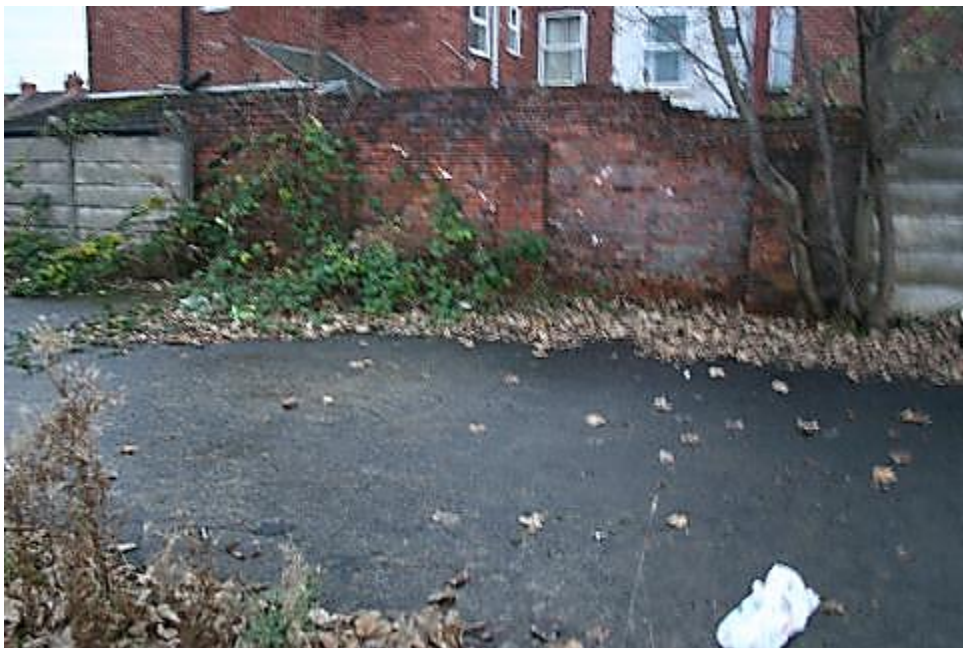
Plate 10: Part of brick wall at southern end of site, towards Taylor Street
