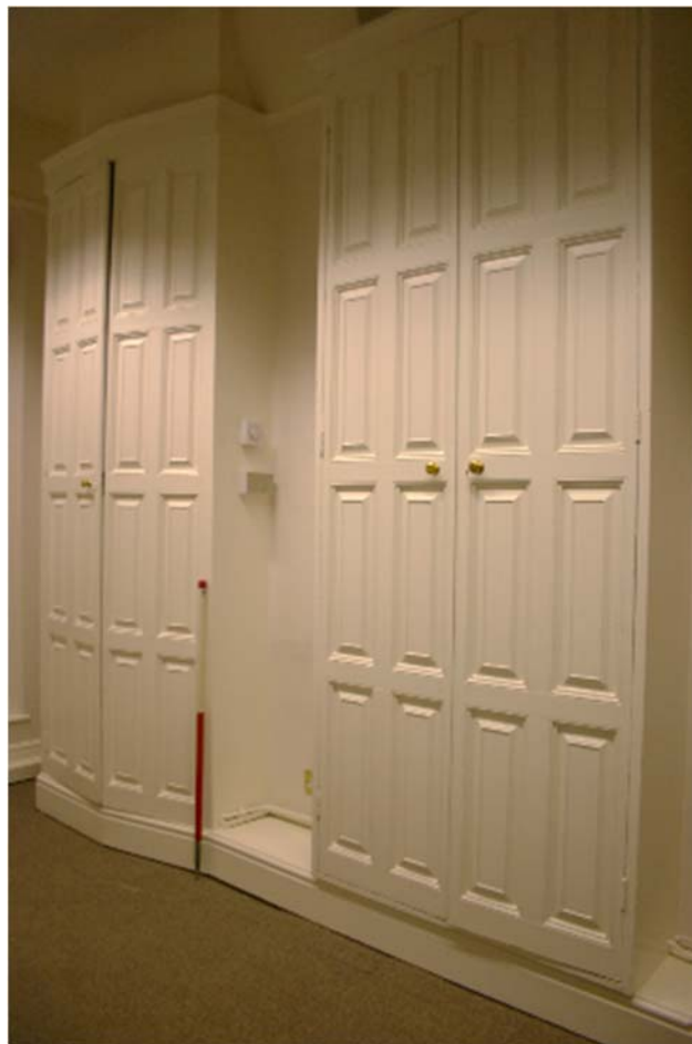
Plate 18: No 20 west room, ground floor, built in timber cupboards, possibly associated with use as surgery
