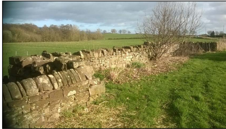
Plate 3: View of recessed areas in south-western boundary wall
