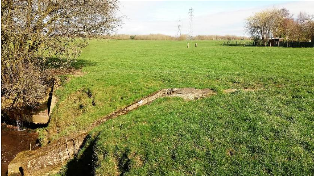
Plate 5: View looking north-east showing the two concrete culverts present in the south-western part of the site
