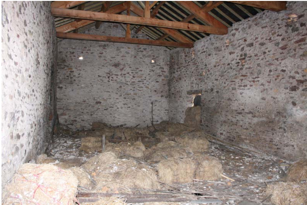
Plate 20: Interior view of barn main building prior to development, by Graham K Norman Architect
