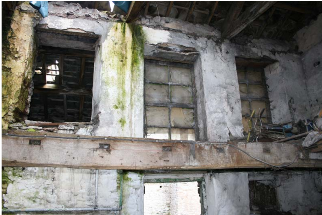
Plate 22: Interior north elevation of garage building prior to development, by Graham K Norman Architect
