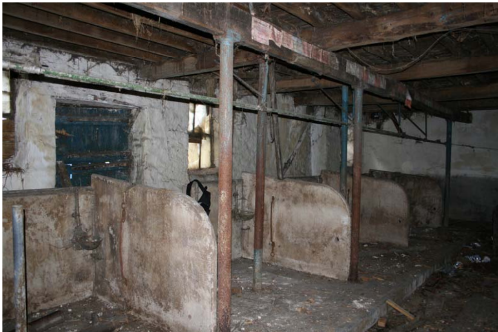
Plate 21: Interior view of building prior to development, by Graham K Norman Architect
