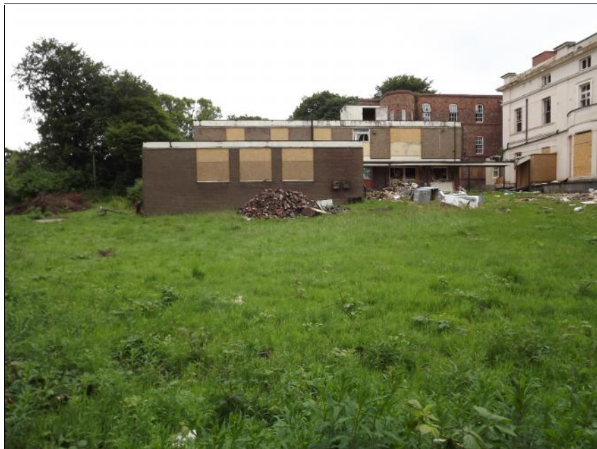
Plate 5: View looking south showing the north elevation of the former Nursery Building (No.8 on Figure 2)
