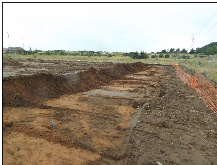
Plate 1: Water monitoring post in bund area, facing south-west
