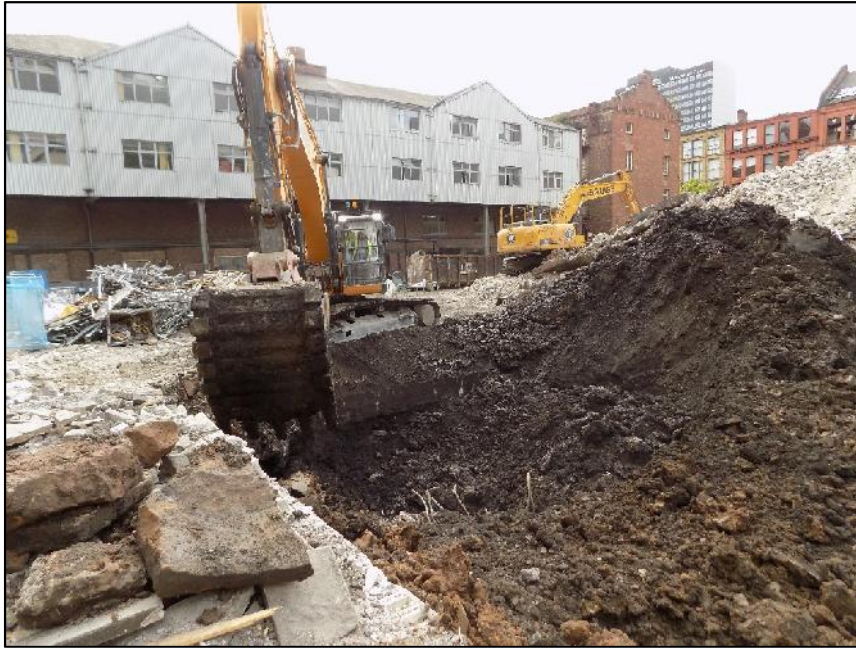
Plate 3: View looking west showing the excavation of Block C, with one of the concrete beams visible behind the excavator bucket (June 2017)
