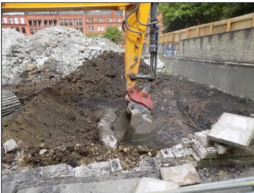
Plate 2: View looking north-west showing one of the 1960s horizontal concrete and steel beams being removed, Block C (June 2017)
