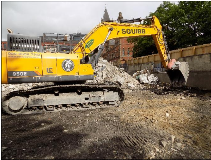
Plate 1: View looking north showing the area of excavation on 1 st June 2017, south-east end of Block C
