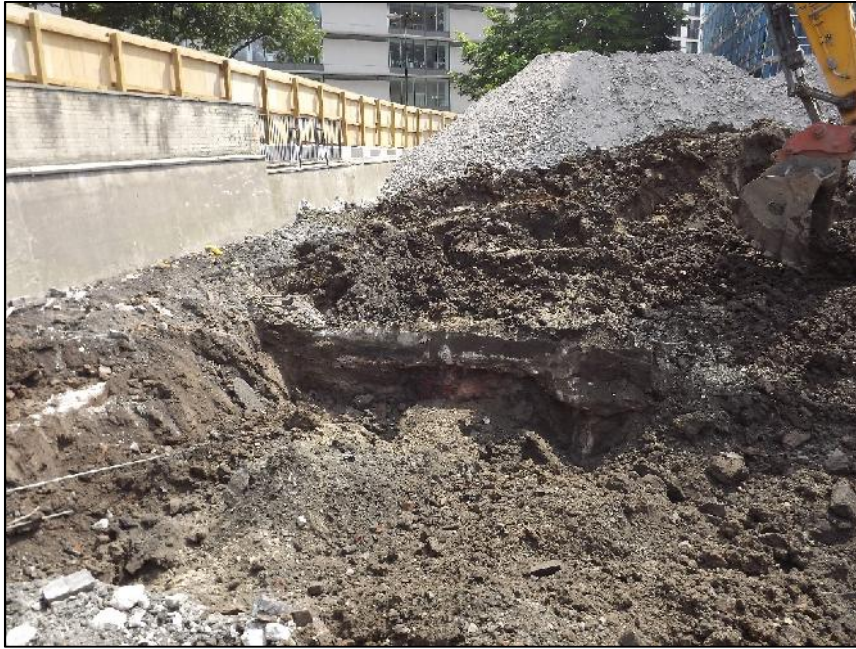
Plate 9: View looking south-east showing section of brick wall directly below one of the horizontal concrete beams, Block C (June 2017)
