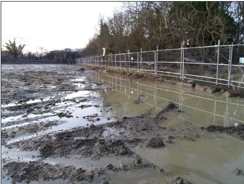
Plate 2; PHASE 1 - general shot of northern end of Site, facing northwest with no scale
