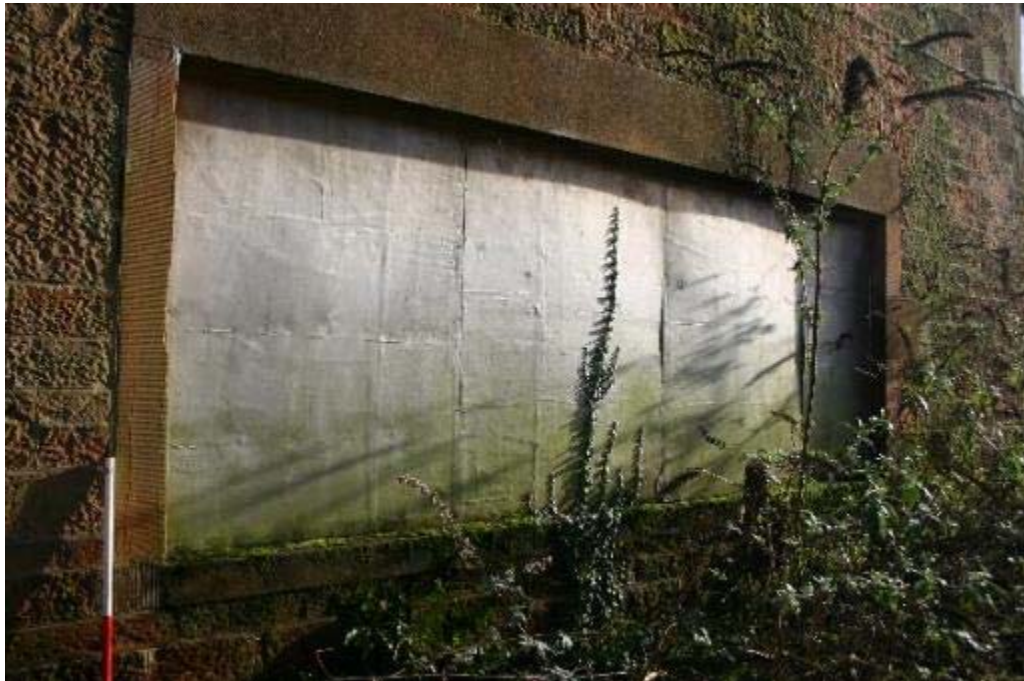
Plate 15: West facing elevation, boarded up large window front at No 25
