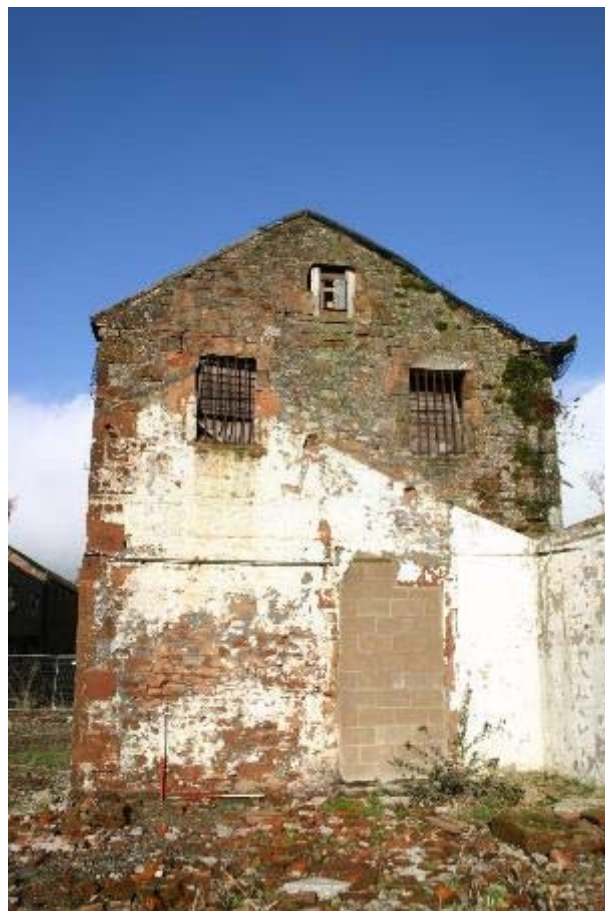
Plate 23: South facing elevation of No 25 with roof scarring
