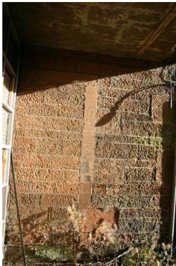
Plate 13: West facing elevation, blocked off opening at northern section at overbridged driveway
