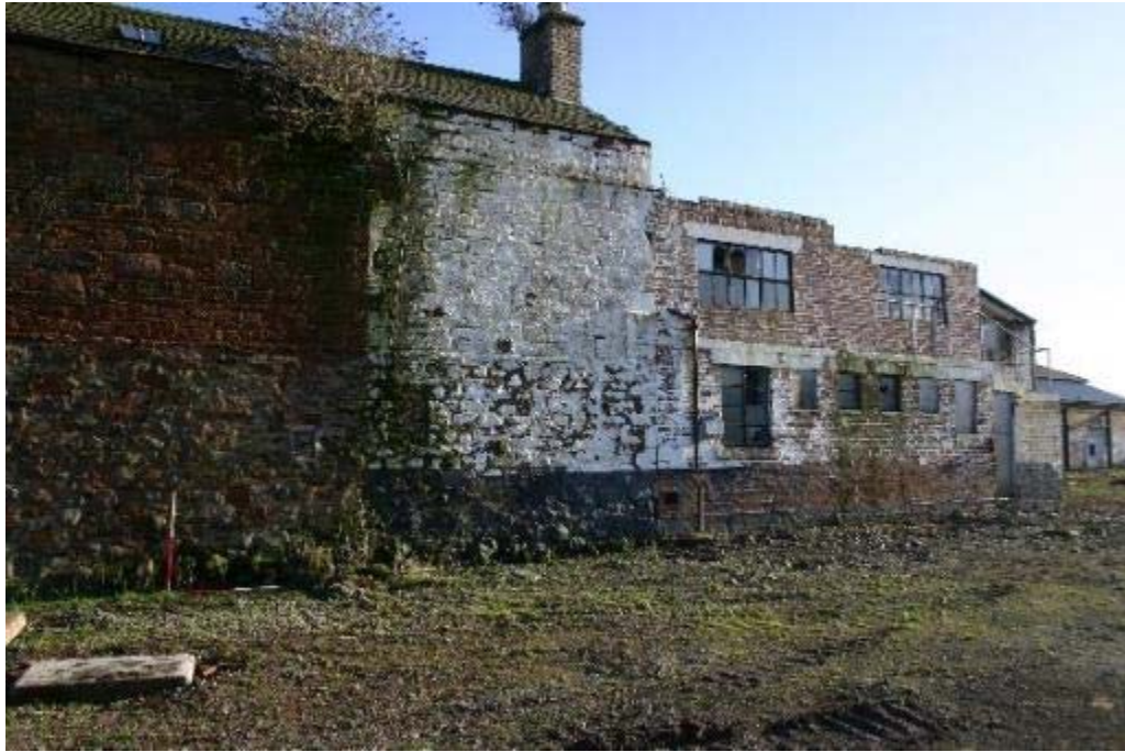
Plate 10: West facing elevation, southern central section and southern modern addition of No 23
