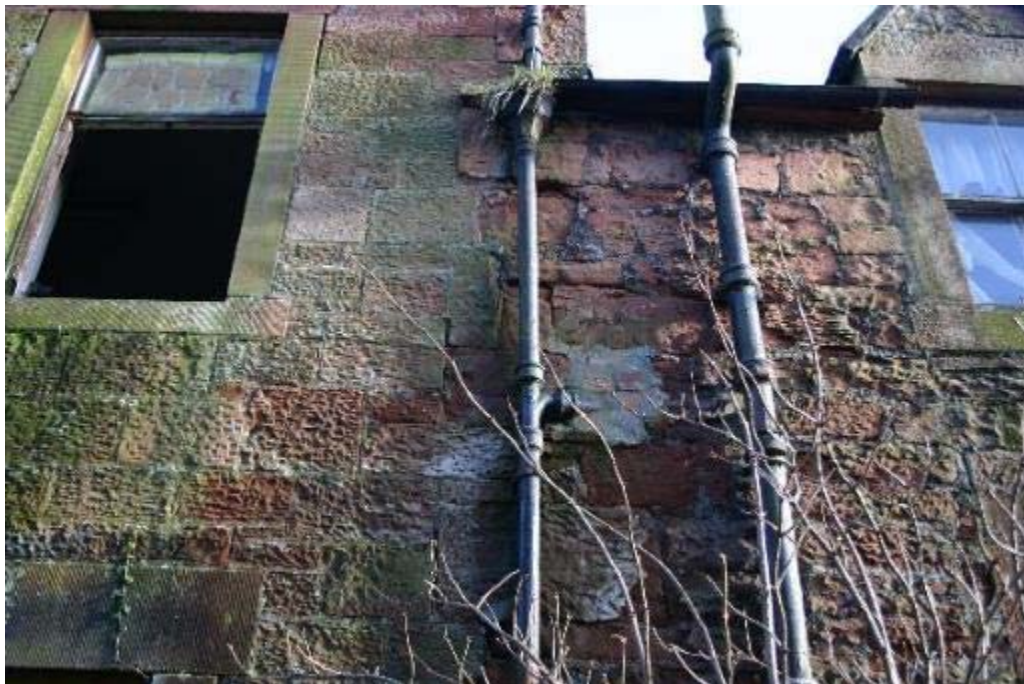
Plate 16: West facing elevation, transition from 1920's building to mid to late 19 th century building of No 25
