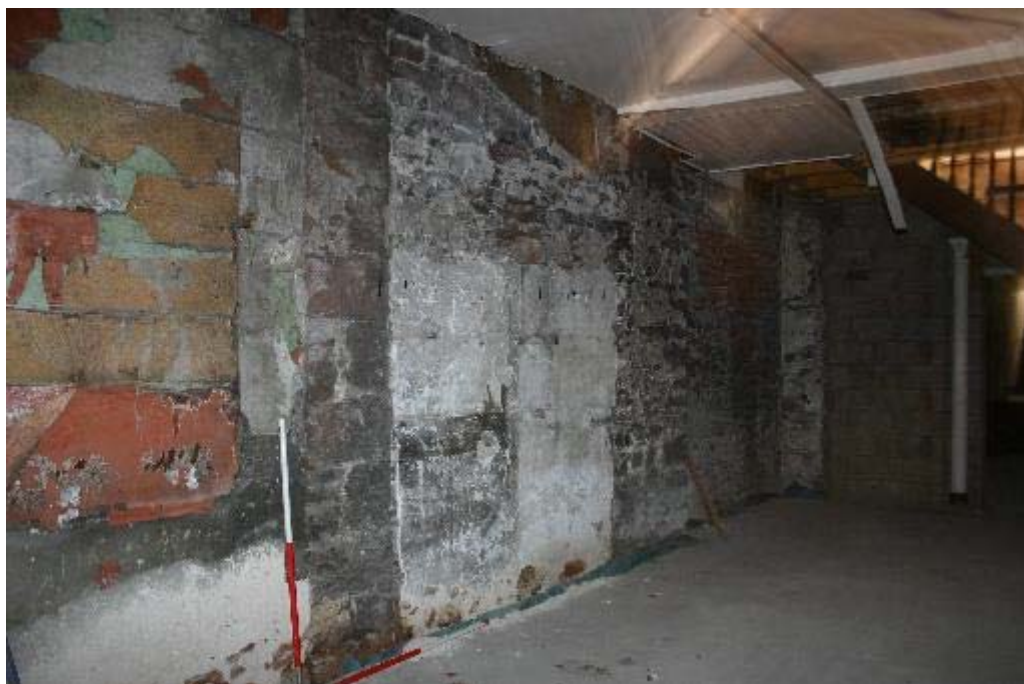
Plate 46: No 25, GF 2 east elevation with blocked openings towards the current police station
