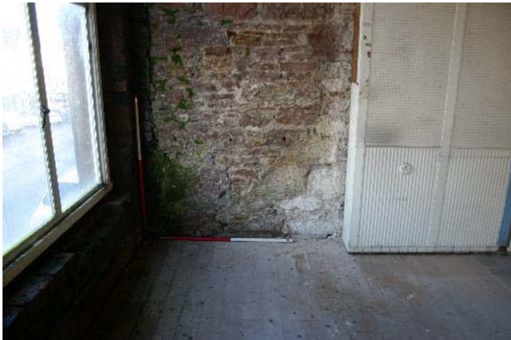
Plate 71: No 25, FF5 roof scarring at the east elevation
