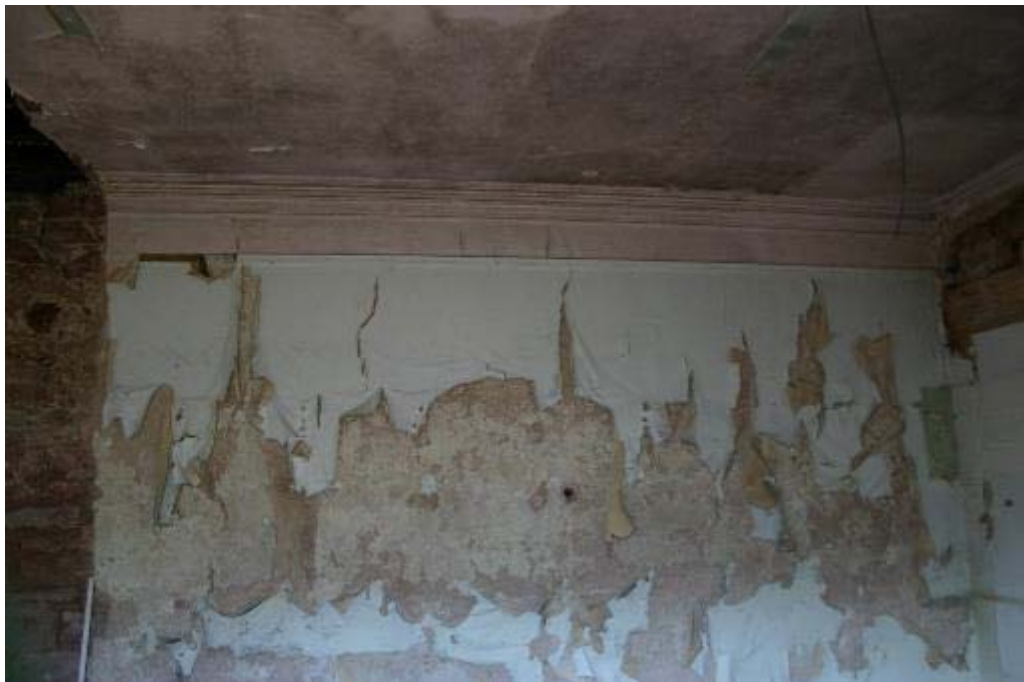
Plate 67: No 23, FF4 remnants of the decorative coving and picture rail
