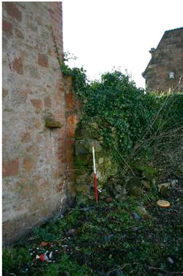
Plate 82: Remains of stone boundary wall to the south of the small yard
