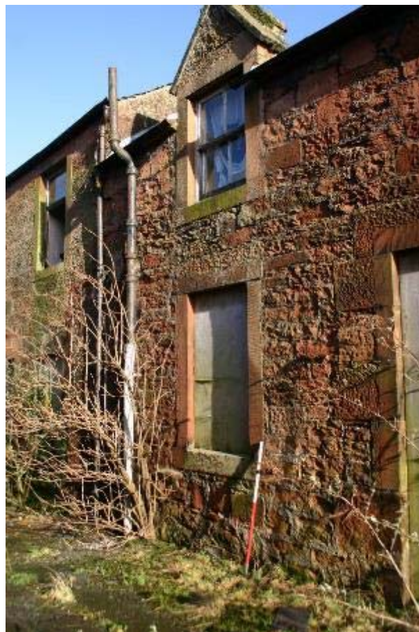
Plate 17: West facing elevation, half dormer window of mid to late 19 th century possibly residential building of No 25
