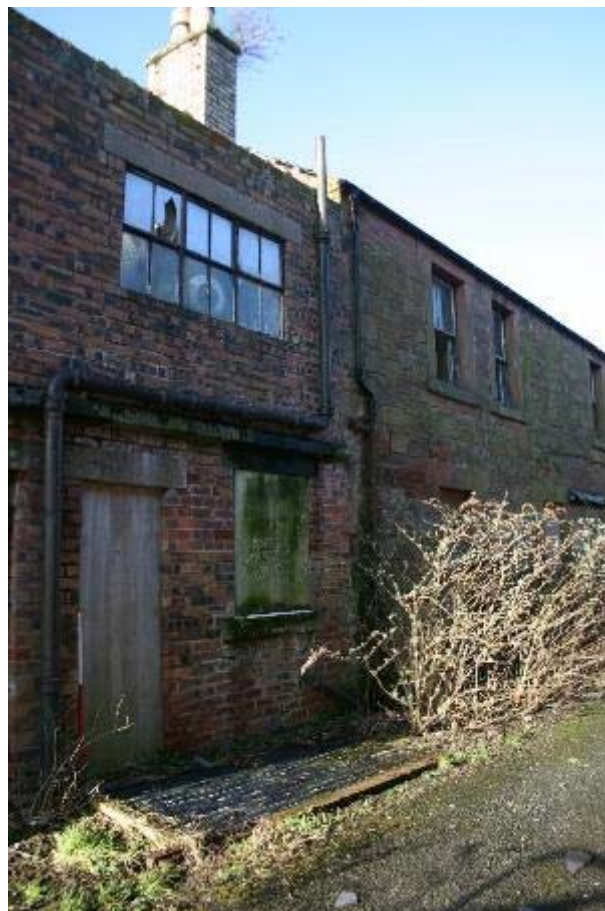
Plate 25: East facing elevation, transition from modern brick structure to mid to late 19th century structure at No 23
