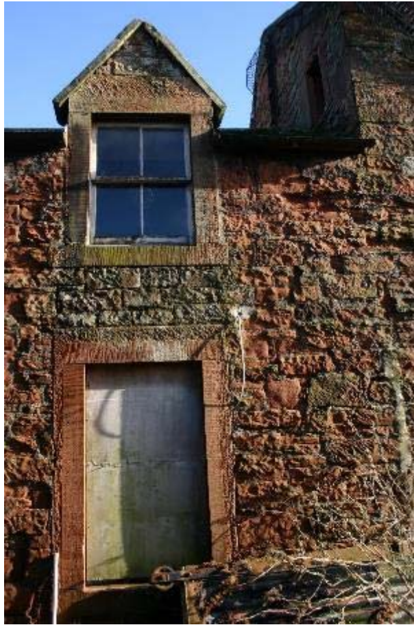
Plate 19: West facing elevation, no visible break in fabric between the residential like building and the larger industrial style building
