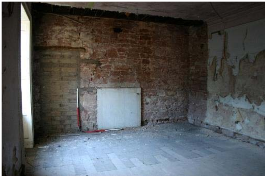
Plate 65: No 23, FF4 view to the south with blocked off doorway and fireplace
