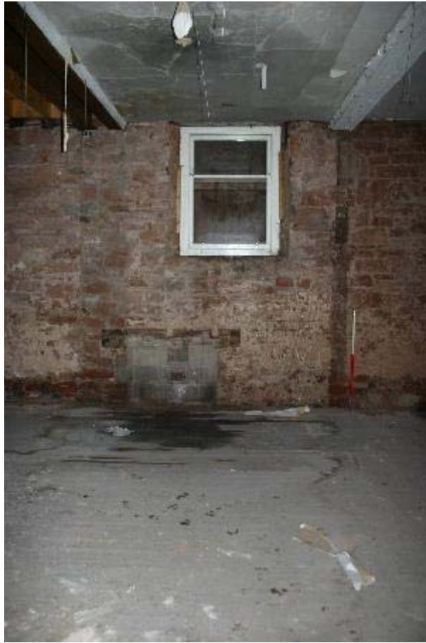
Plate 55: No 23, GF5 blocked up opening and boarded up staircase window at west elevation
