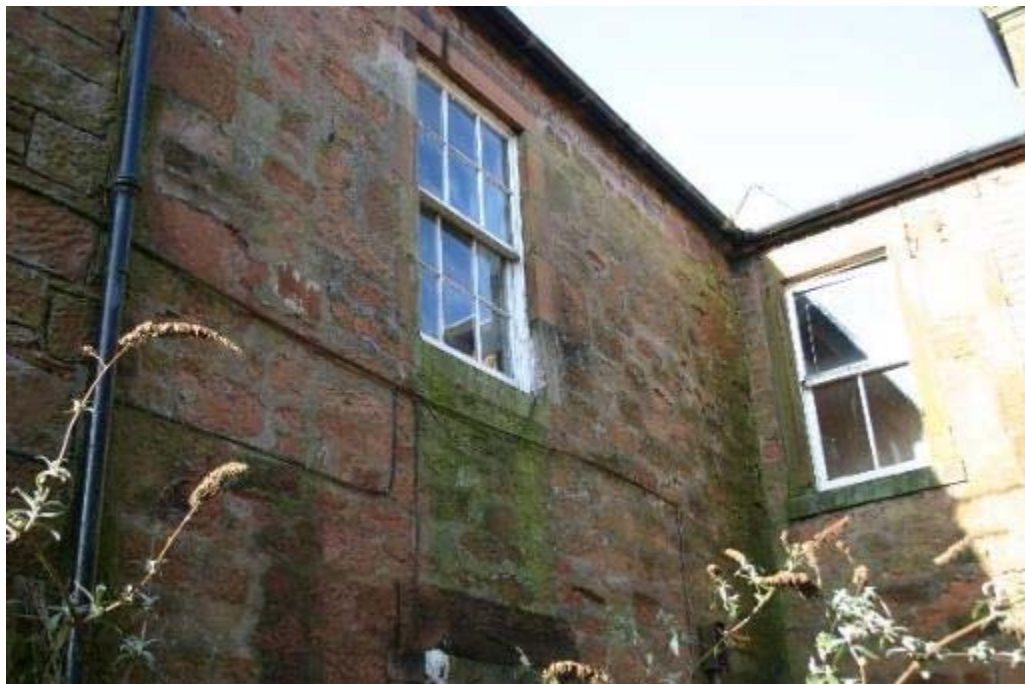
Plate 28: East elevation, visible break in fabric at the level of the drainage pipe
