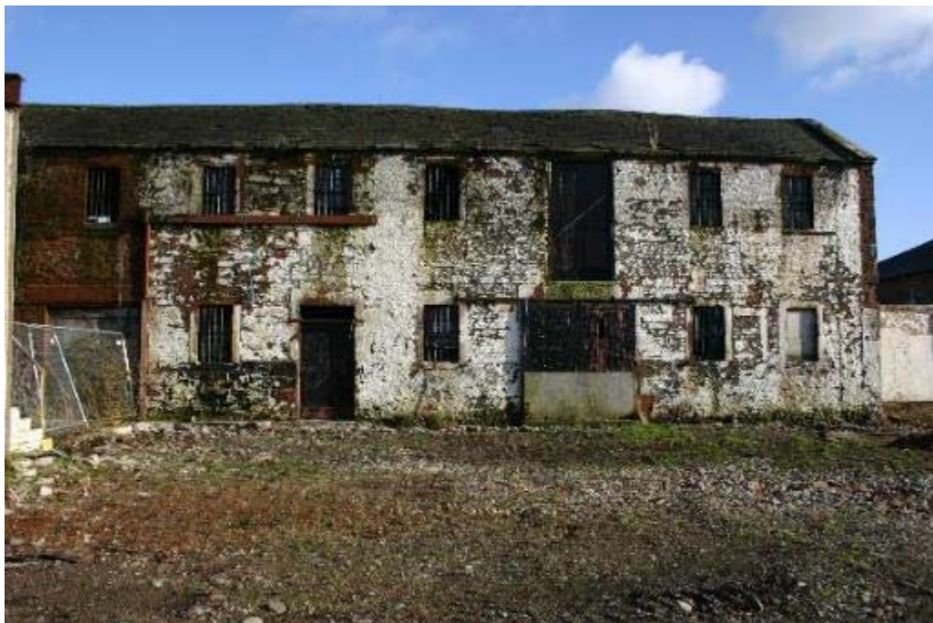
Plate 21: West facing elevation, painted section of the possibly industrial building of No 25
