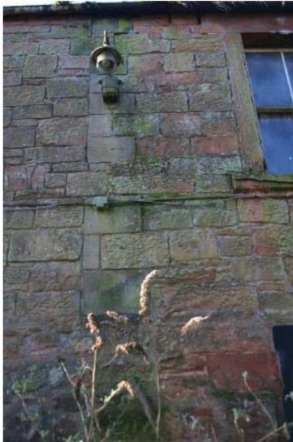
Plate 26: East elevation, visible break in fabric and modernised historic lamp at No 23
