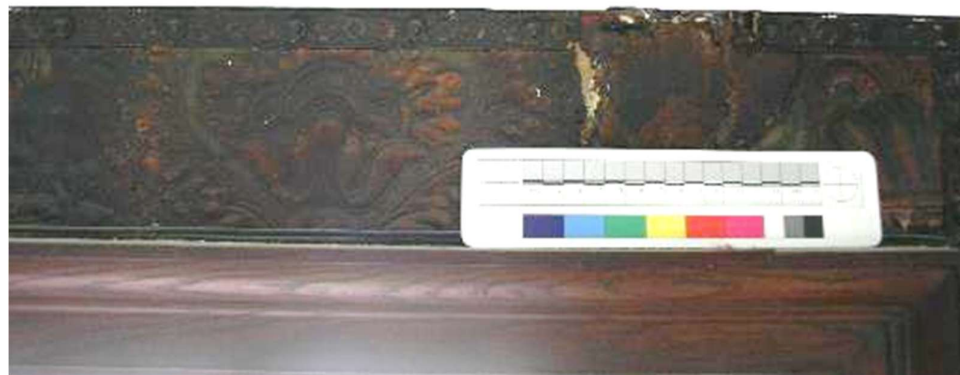
Plate 18: Easternmost section of wallpaper, covered up damage
