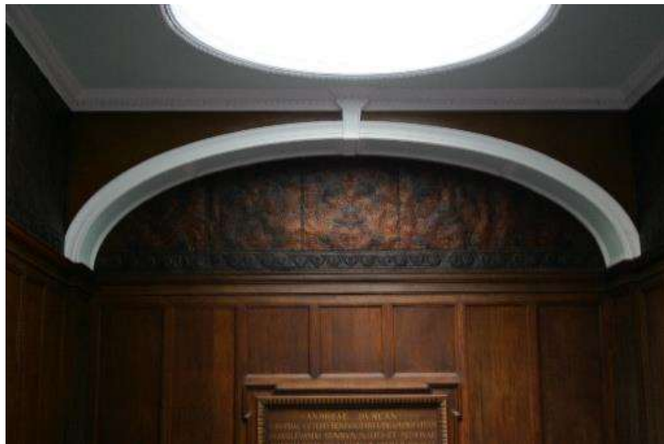
Plate 4: Visibly bubbled section above the staircase
