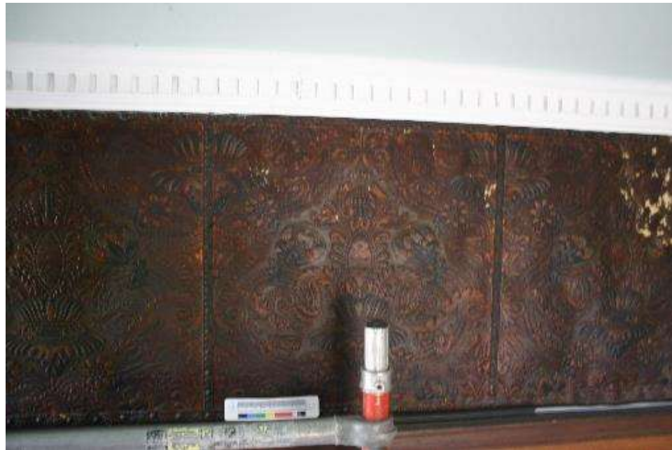
Plate 17: Easternmost section of wallpaper, damage in corner
