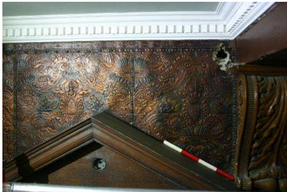
Plate 10: Northern section of wallpaper on lower level, damage from hole at corner
