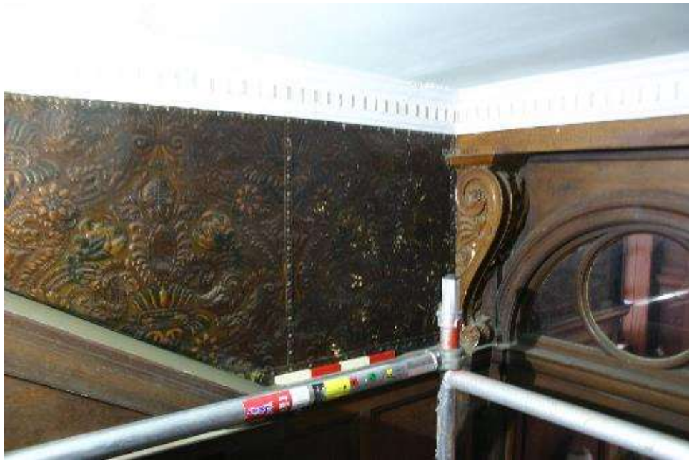
Plate 8: south section of wallpaper on lower level, visible damage in corner
