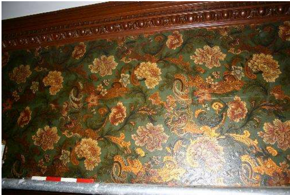
Plate 3: Detailed view of a section of wallpaper at the eastern section of the north elevation
