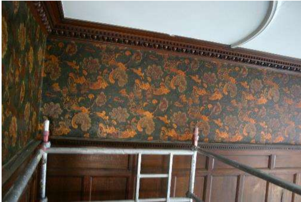
Plate 2: General view of the current condition of the wallpaper at the east elevation
