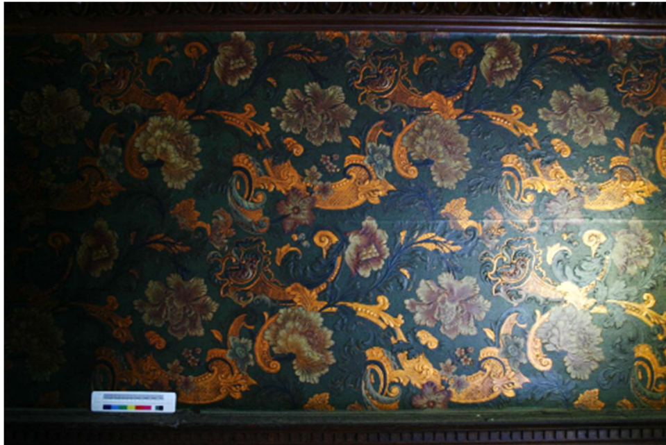
Plate 4: Detailed view of the wallpaper at the western section of the north elevation
