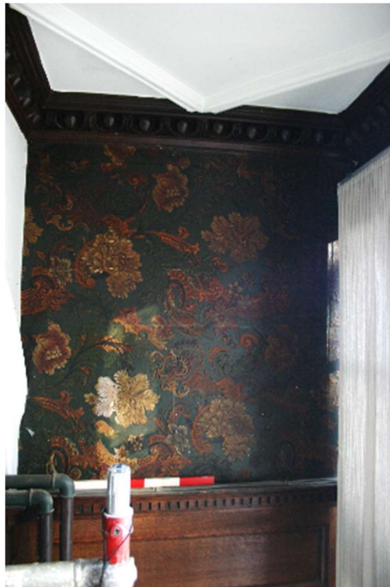
Plate 5: Detailed view of the wallpaper at the southern end of the east elevation, with noticeable clear area
