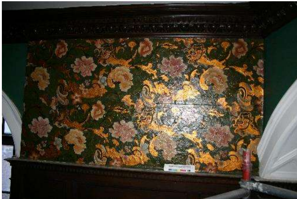
Plate 6: Noticeable different looking, previously restored section of wallpaper at the south elevation
