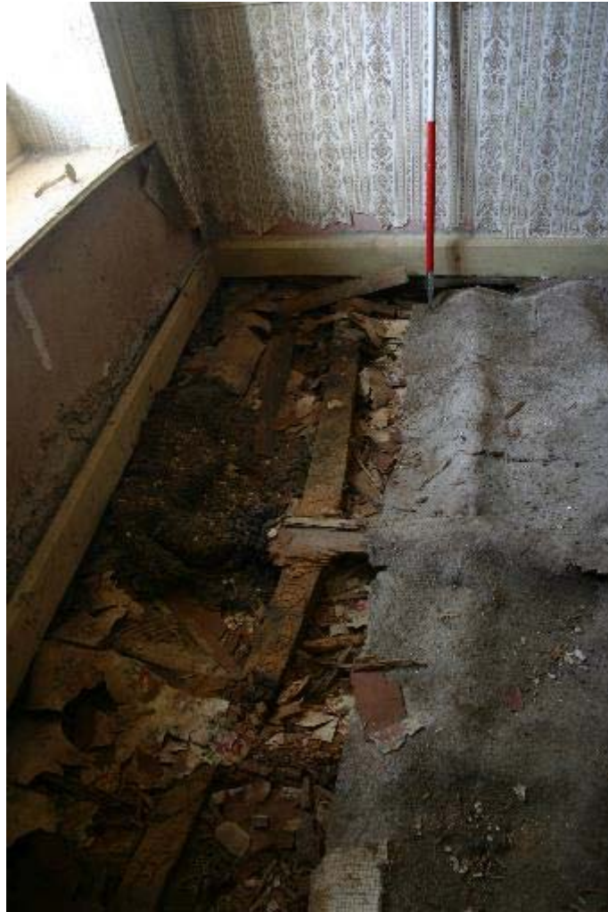
Plate 14: GF-3, current condition of the flooring
