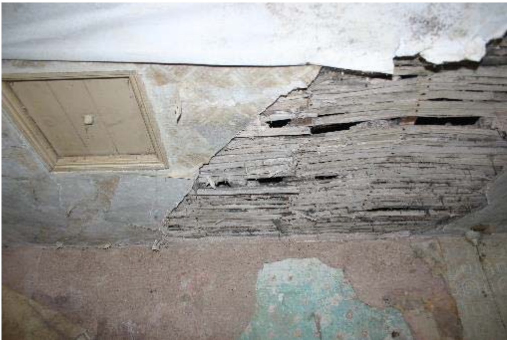
Plate 37: FF-4 damage to ceiling and wall
