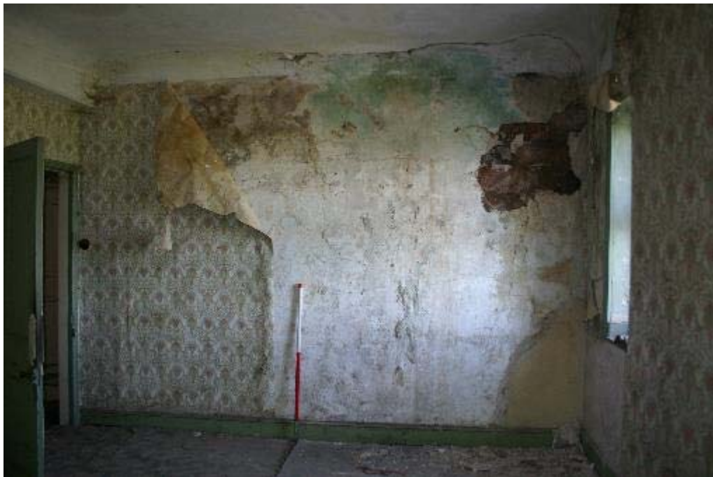
Plate 34: FF-3 damage to wall
