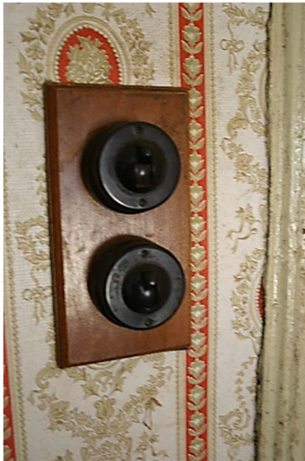
Plate 11: GF-2, Bakerlite light switches
