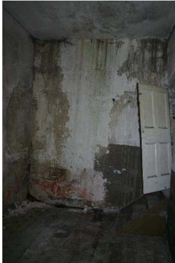
Plate 40: FF-6 damage to wall and flooring
