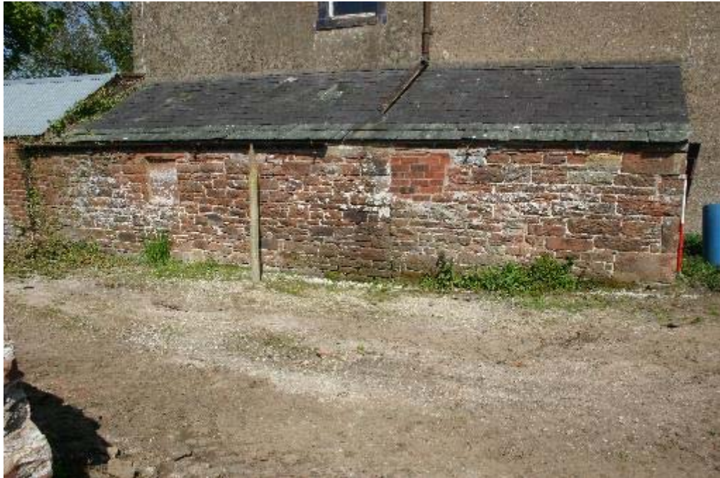
Plate 45: Break in fabric to the north of the red brick repair
