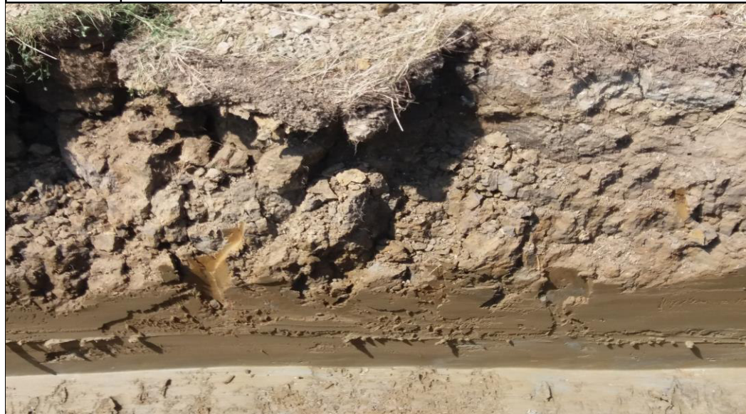
Picture Taken: 12/07/2018 Plate No. 12 Title: Eastern side of cable trench 4.3 within Area A, facing E.
