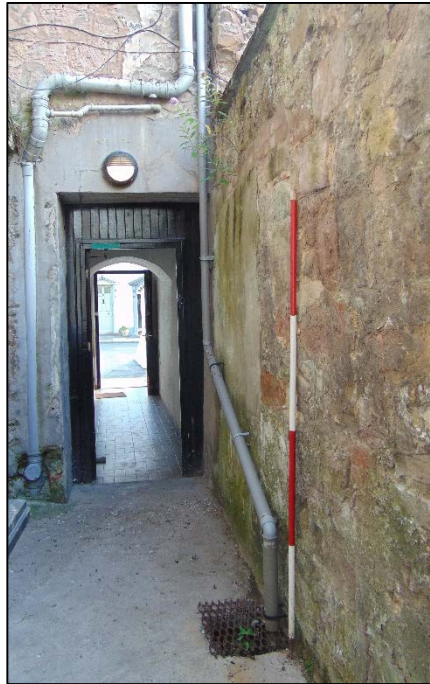
Plate 13: Blocked former opening towards south-eastern extent of wall, north-east facing elevation, facing south-east
