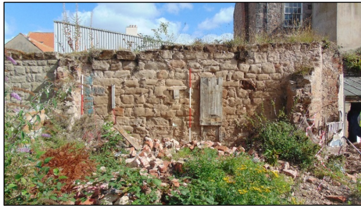
Plate 2: Remains of former abutting walls (left and right) and timber fixtures on south-west elevation of western part of wall
