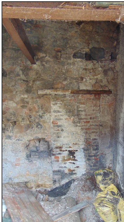
Plate 12: Former doorway noted within outbuilding in south-west elevation of eastern part of wall
