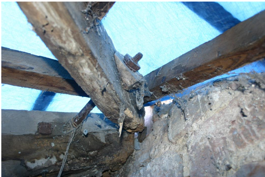
Plate 2: Upper end of principal (c) with hip-rafter (d) fastened to it with a 20th century rod
