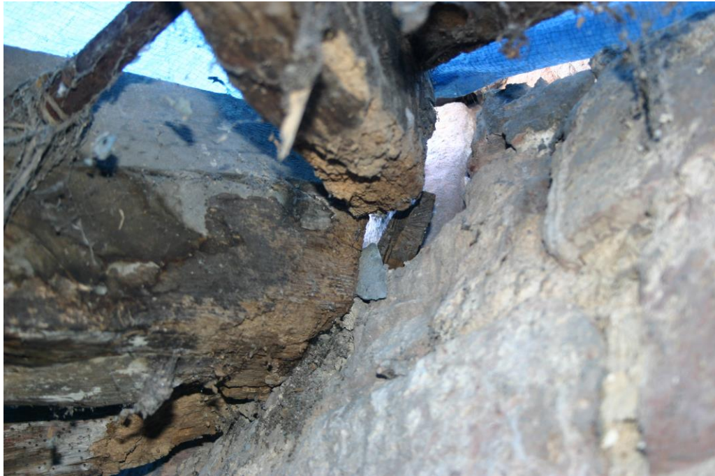
Plate 3: The upper end of roof is not attached to the elevation
