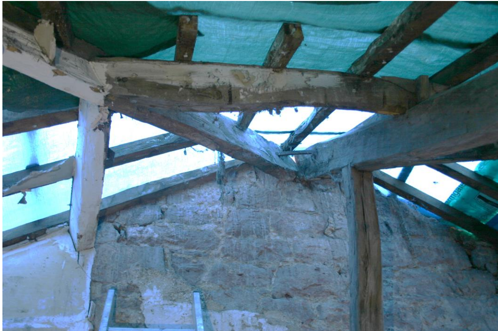
Plate 5: Dowel holes in purlin (f)
