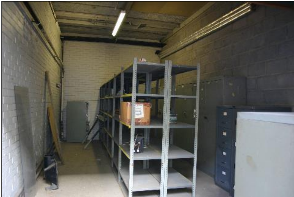
Plate 37: GF26 storage room, looking north, with recent breeze block partition wall to GF15
