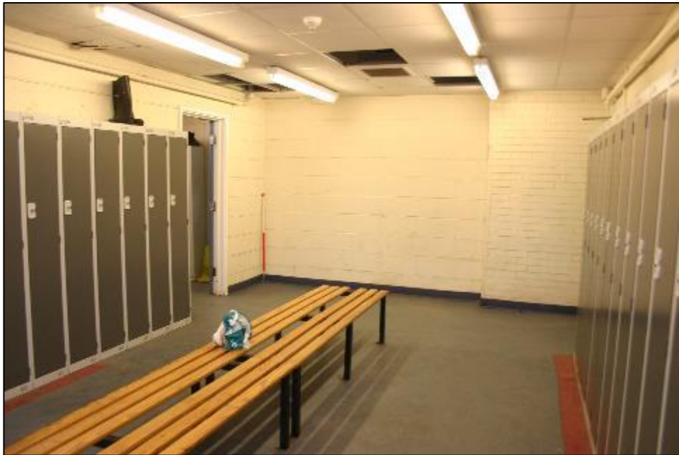
Plate 17: GF12 looking north, noticeable: large opening blocked up with concrete breeze blocks
