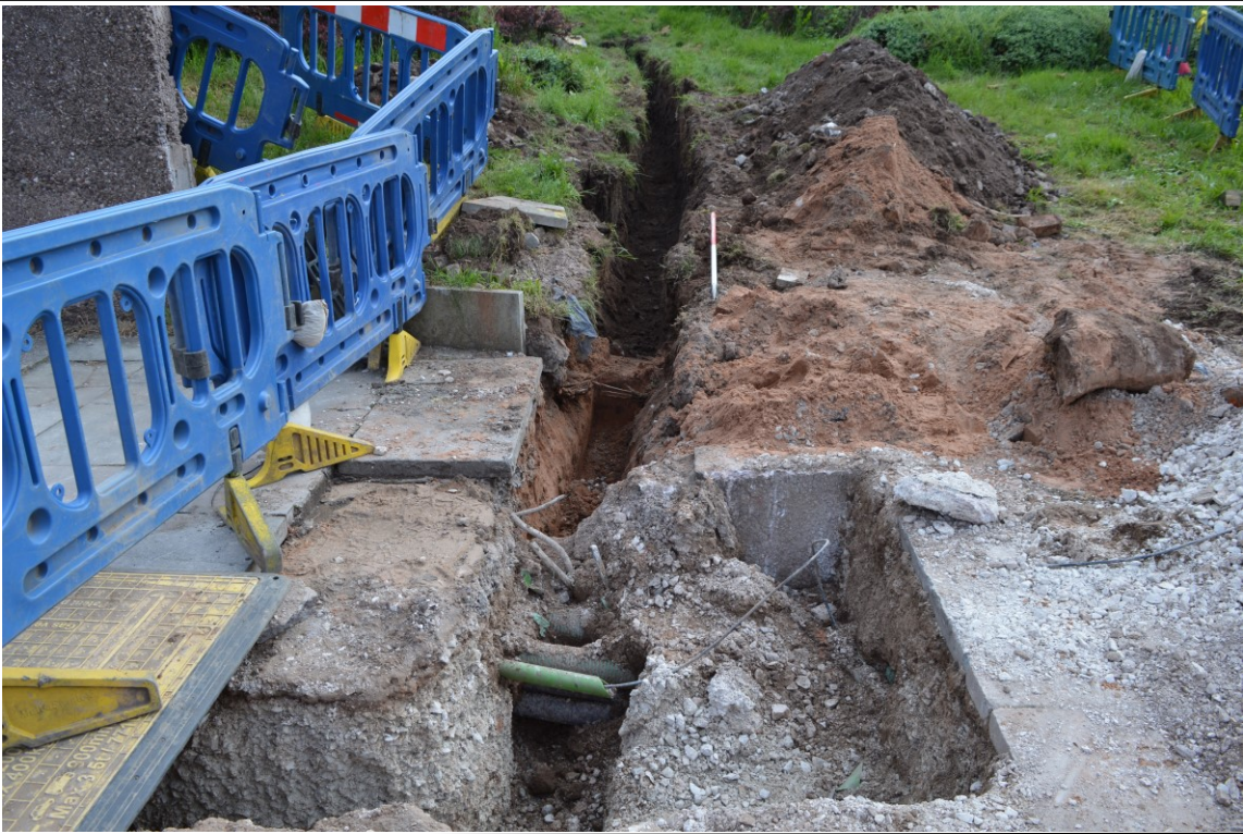
Picture Taken: Plate No. 35 Title: Excavation for gas diversion through open green, looking east with 1m scale
