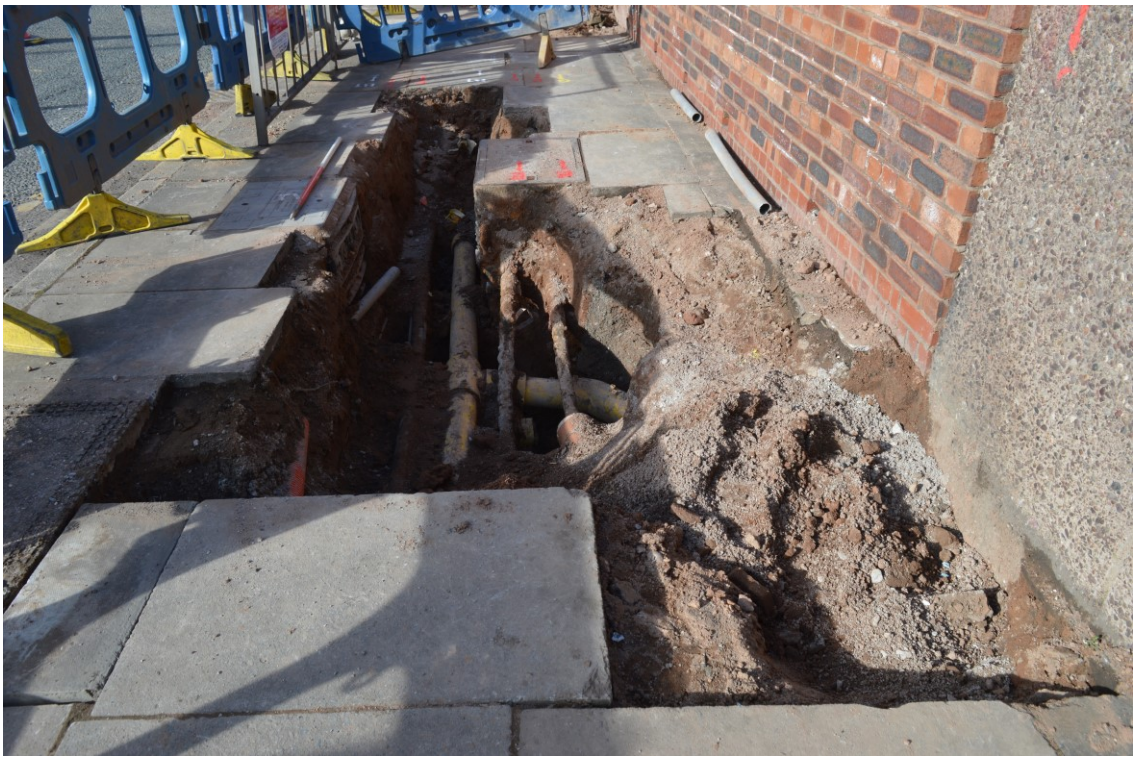
Picture Taken: Plate No. 41 Title: Excavation for gas diversion within footpath bounding St. Martin's Way, looking north with 1m scale
