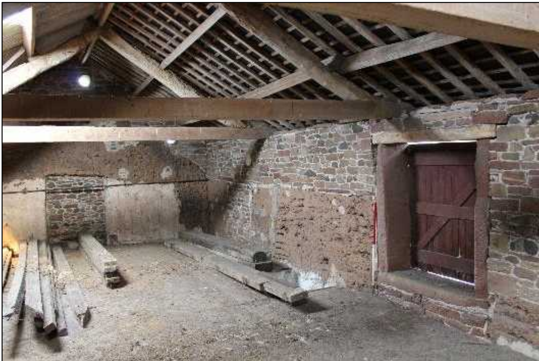
Plate 88: Building F, loft space, north elevation (Feature 111) and northern extent of eastern elevation
