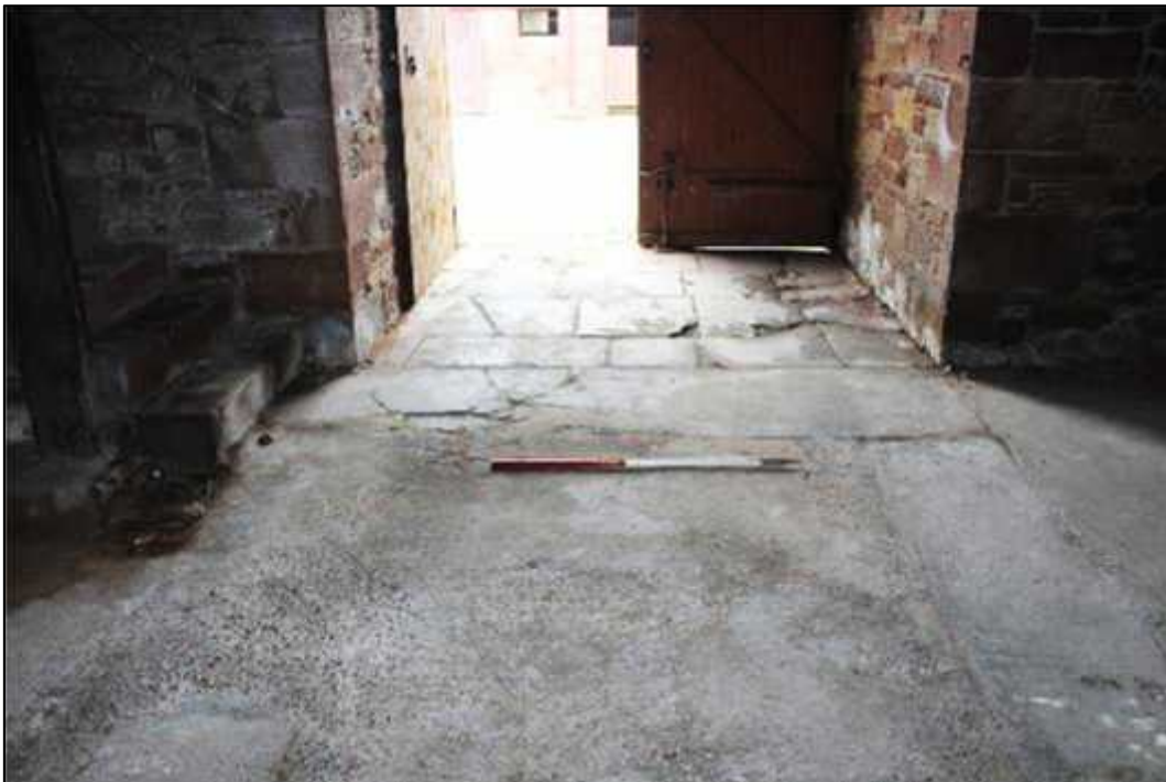
Plate 20: Interior of Building B, southern extent, showing flagged flooring at canopy entrance (Feature 110)
