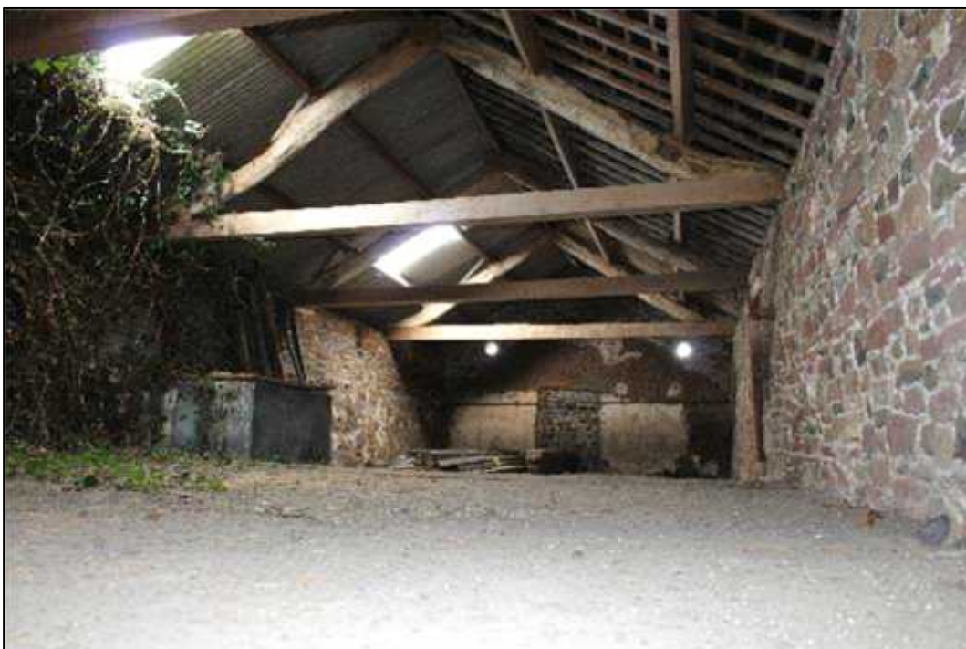
Plate 90: Building F, loft space, north elevation and northern extents of western and eastern elevations
