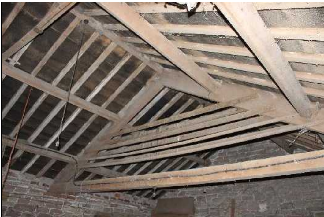
Plate 36: Building B: central section, interior of loft space above cart entranceways, roof structure
