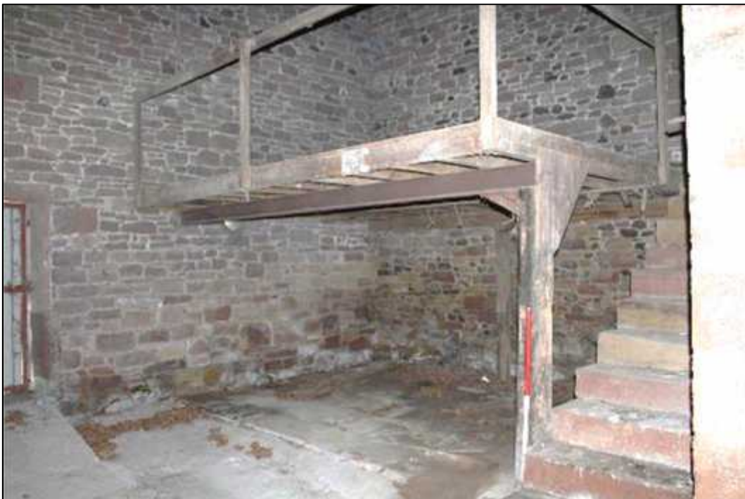
Plate 22: Interior of Building B, northern extent, showing inserted floor above south bay (Feature 117)
