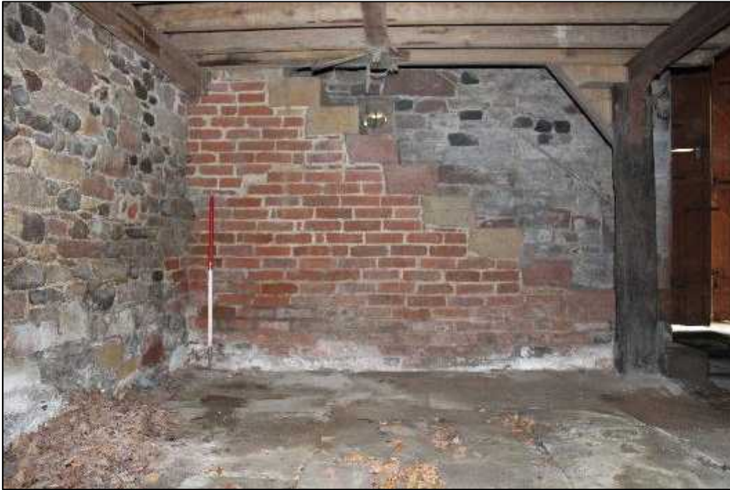
Plate 23: Interior of Building B, northern extent, showing stairway in south bay (Feature 104)
