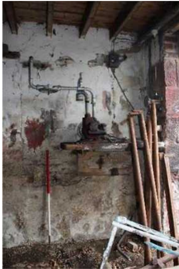
Plate 33: Building B: central section, interior of southern cart entranceway, south elevation with machinery (Feature 106)
