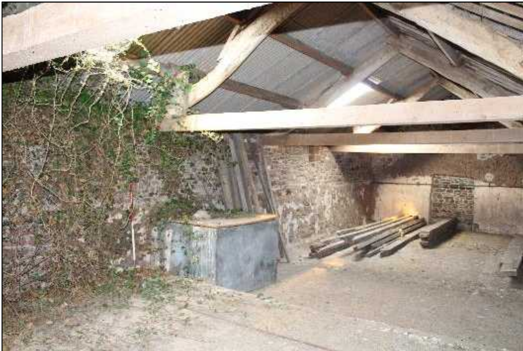
Plate 89: Building F, loft space, north elevation (Feature 111) and northern extent of western elevation
