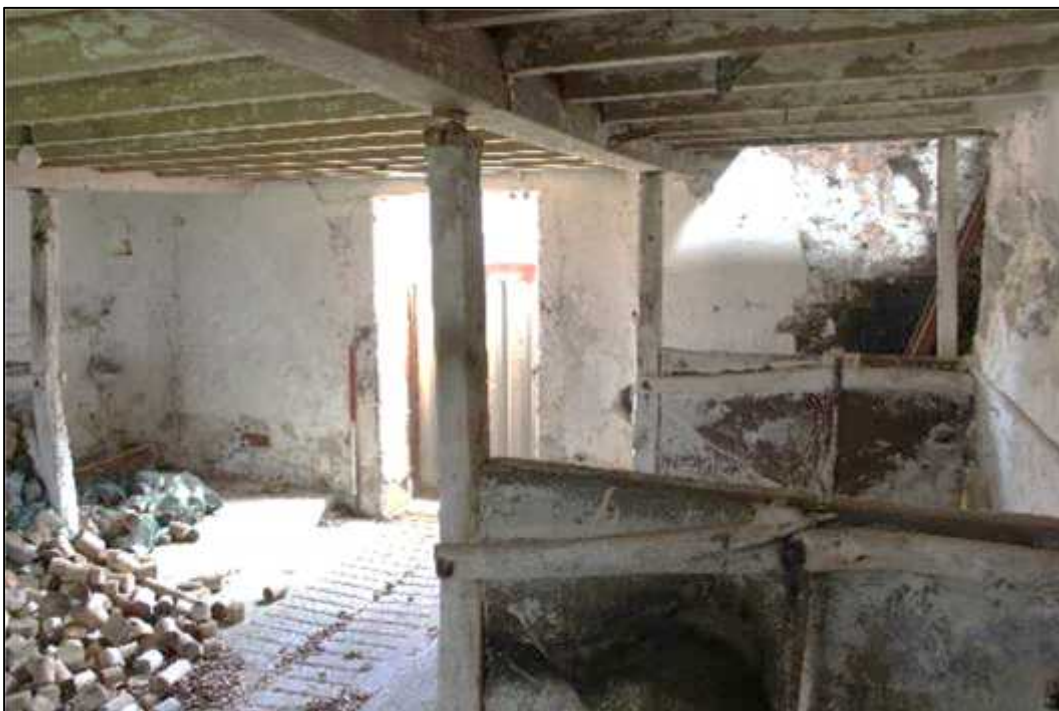
Plate 76: Building F, southern byre, east elevation with door, stalls and boskins (Feature 109)
