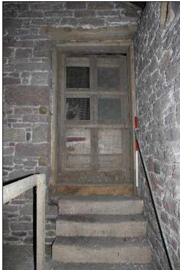
Plate 24: Interior of Building B, northern extent, showing doorway at first floor level
