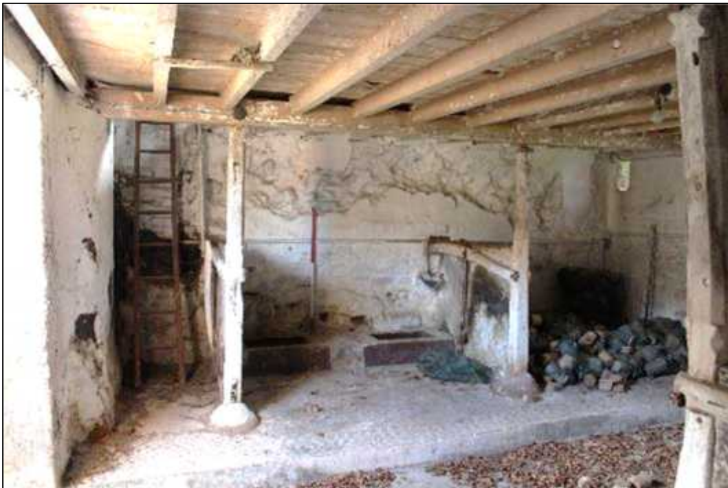
Plate 74: Building F, southern byre, south elevation with stalls, boskins (Feature 109) and loft access
