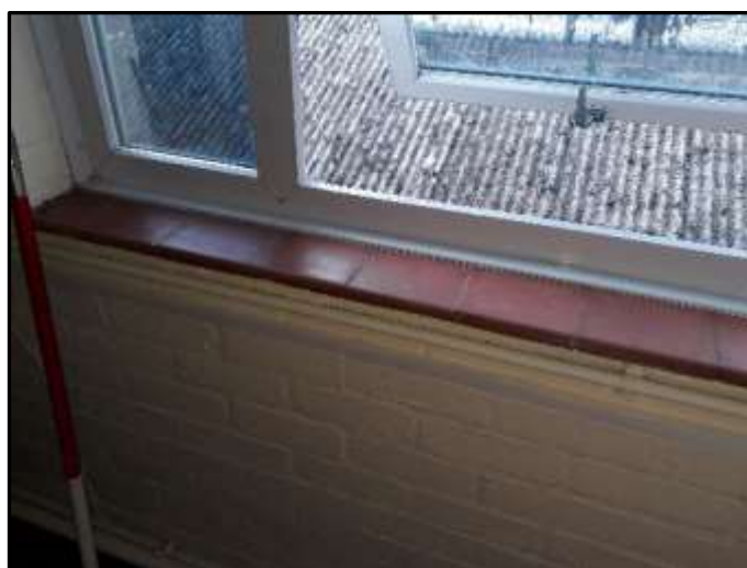
Plate H34 – H Building, tiled sill and painted brickwork interior to the first offices of the north range
