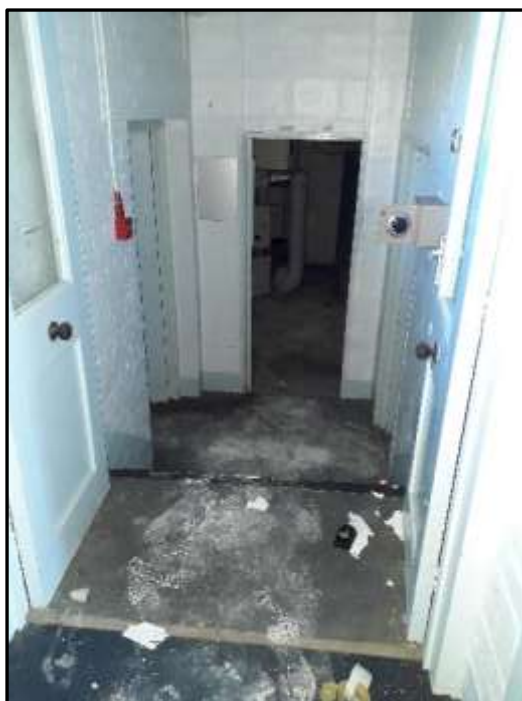
Plate A52 – A Block, steps down into the original boiler house area accessed from the central corridor opposite the main central entrance
