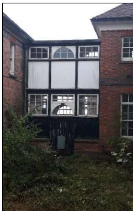
Plate S10 – Block S, west elevation of the timber link addition between the central and southern ranges
