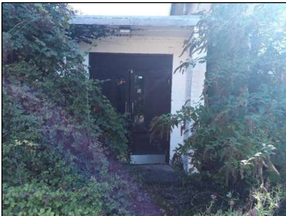
Plate A23 – A Block, secondary entrance to the central corridor range at the junction between spurs 1 (right) and 2 (left)
