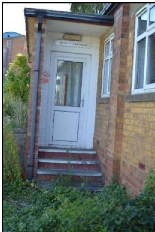
Plate L15 – Library building, north west entrance into later flat roof porch addition to the north east elevation of the original range
