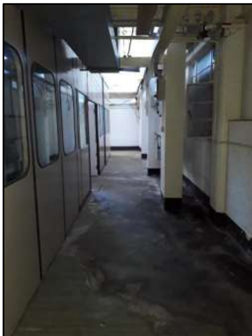
Plate A43 – A Block, infill extension between spurs 2 and 4 originally used for climatic testing of complete systems. Remaining features indicate research use continued within the space
