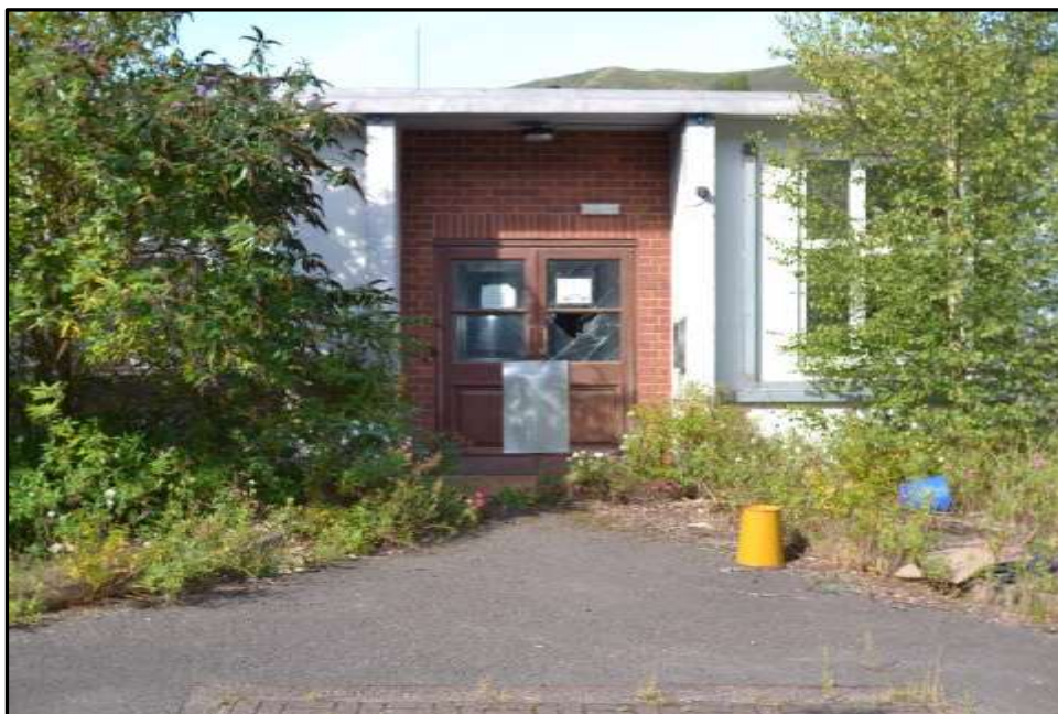
Plate D17 – D Block, secondary entrance into the block from the east. Entrance marks the central corridor location which separate spurs 1, left, and spur 2, right
