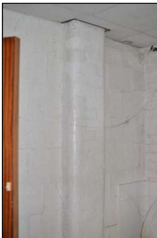
Plate KF10 – Example of rounded edge of brick column visible to the corridors and internal rooms
