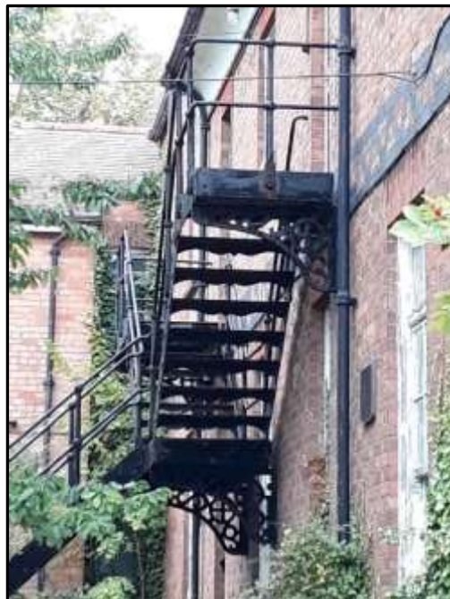
Plate S16 – Block S, external metal stair to the south elevation of the southern range
