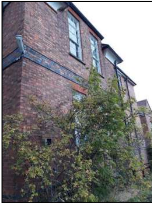
Plate S5 – Block S, detailing to the east elevation of the southern range
