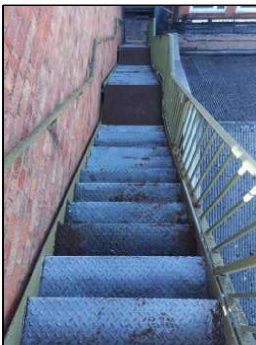
Plate H24 – H Building, external metal staircase to roof of former bunker on the east elevation
