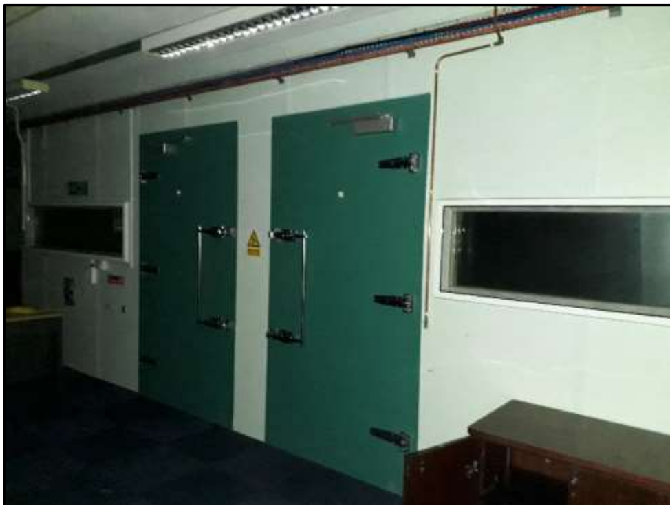
Plate H54 – H Building, first-floor. Sound proof office and conference pods to east wall with wide, secure, metal doors
