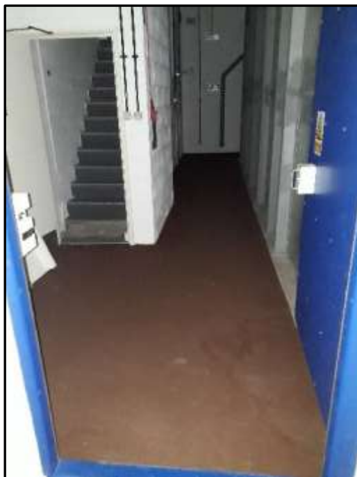
Plate H51 – H Building, ground floor. Enclosed stairwell to first floor, inserted sometime after 1952 and before 1983, likely inserted when the first was created in the late 1950s
