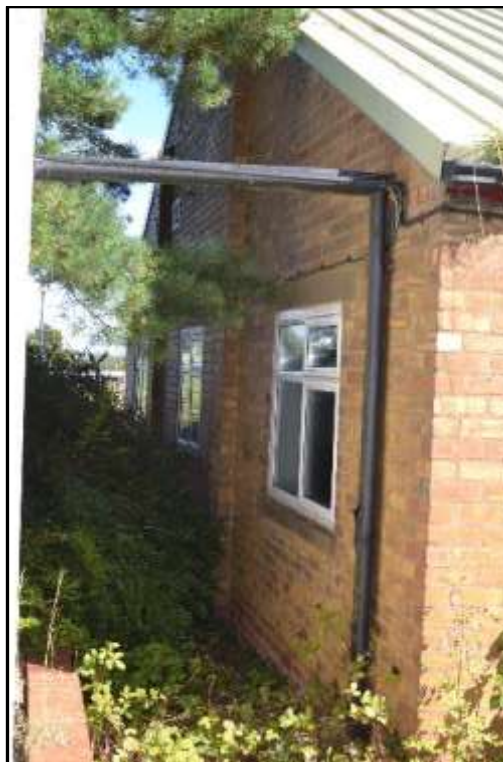
Plate L4 – Library building, part north west end elevation of north east (original) range
