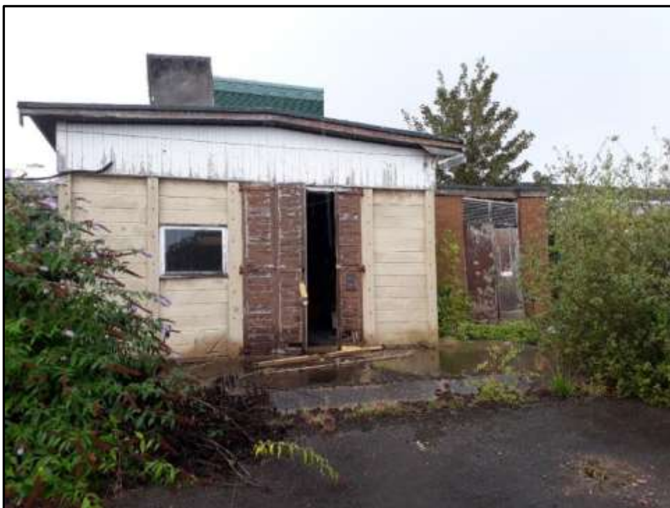
Plate 7b – Building 7, part east elevation of main range and east elevation of garage/store
