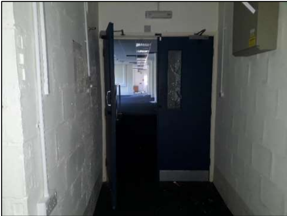
Plate D35 – D Block, looking north into spur 8 from the corridor, not brick structural columns within main space beyond the doors and the brick tile internal walls
