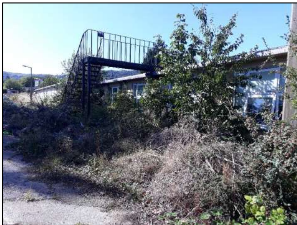
Plate A14 – A Block, south east elevation of spur 8 with later external staircase addition
