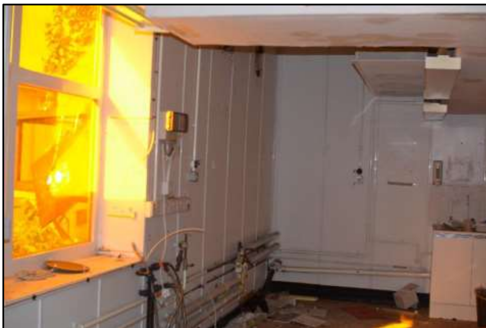
Plate E51 – E Block, spur 8, fixtures and fitting relating to most recent laboratory and research use, the film to the window indicating importance of controlling the type of light into the space
