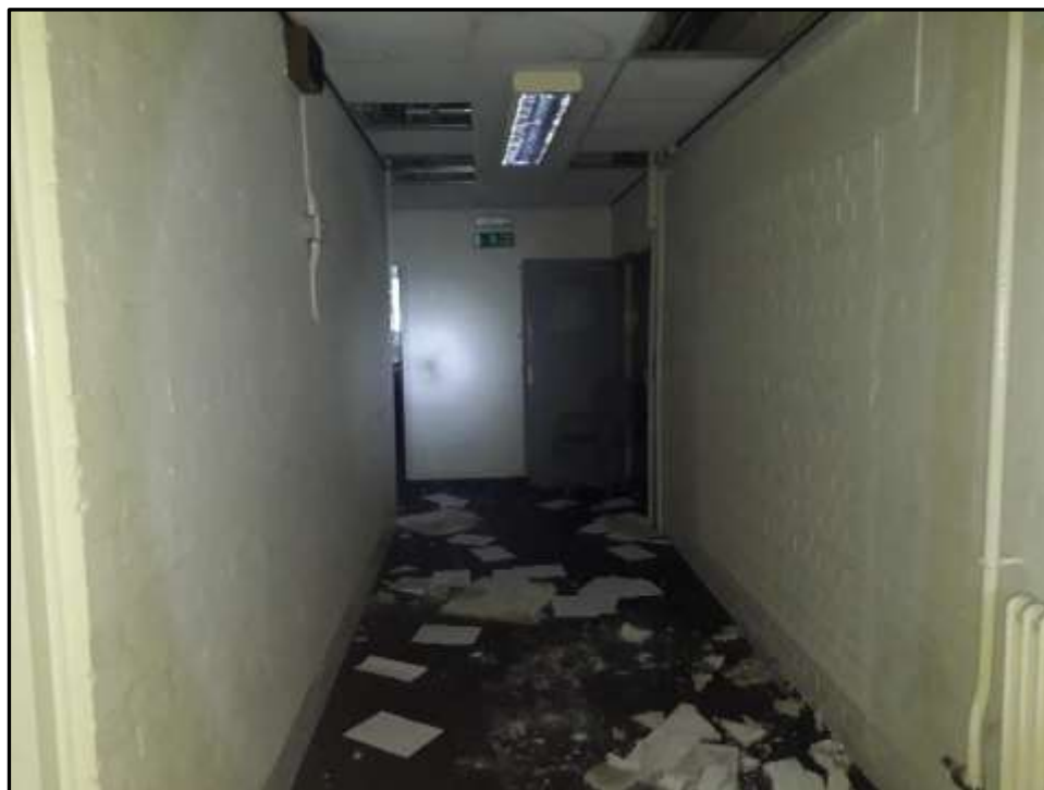
Plate H39 – H Building, ground floor corridor link north and south ranges; former bunker to right of image
