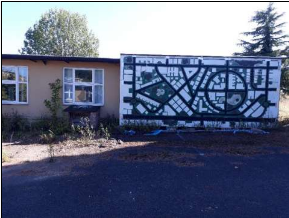
Plate A5 – A Block, laser camera test panel to end bays of spur 5 (north west elevation)
