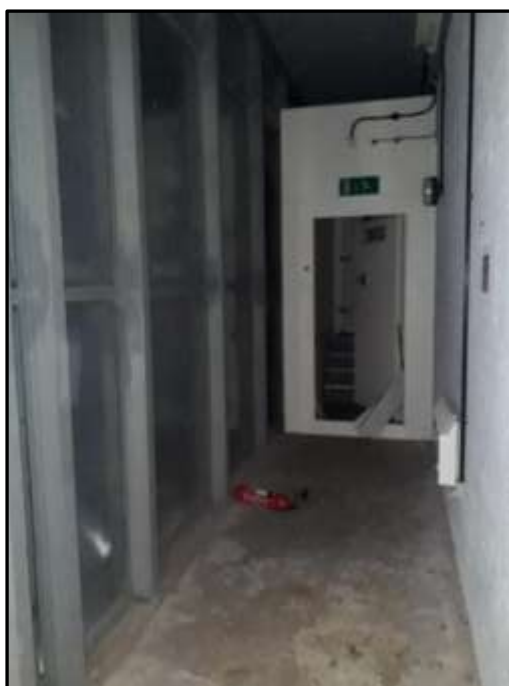
Plate H42 – H Building, perimeter corridor within former bunker area; faraday cage to left of image
