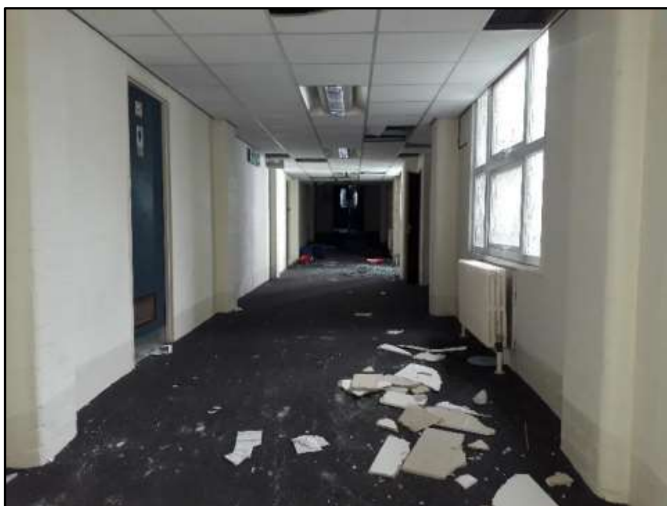
Plate D33 – D Block, central corridor looking west from between spurs 5 and 6. Note inserted ceiling to conceal ducts and services and rounded edges of brick columns and brick tile internal walls to the left
