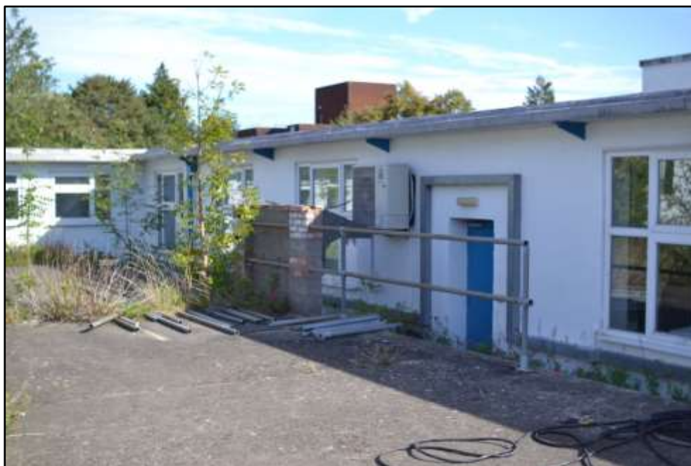
Plate D15 – D Block, west elevation of spur 5 with altered pattern of openings
