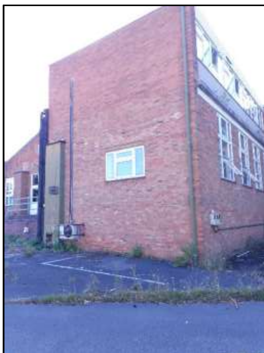
Plate H13 – H Building, part east elevation; change in brickwork denotes first floor extension
