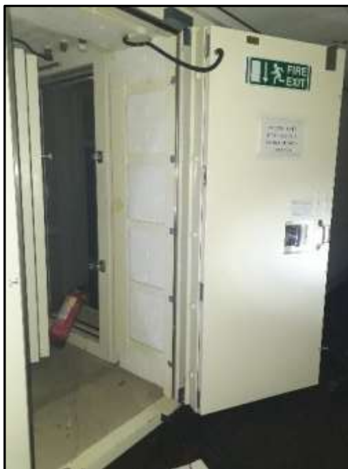
Plate H41 – H Building, main entrance into the former bunker area with dense, wide metal security door
