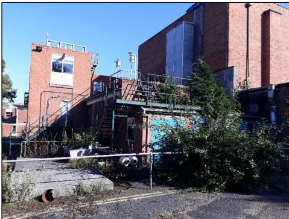
Plate H9 – H Building, part west elevation and part north elevation of former bunker
