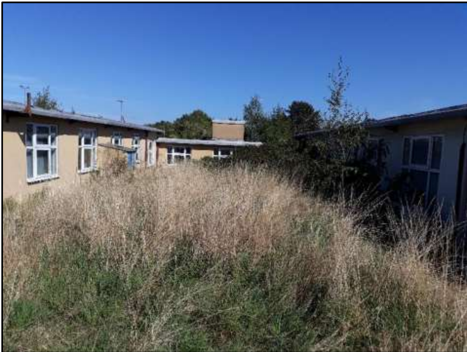
Plate A9 – A Block, view towards central corridor between spurs 5 (left) and 7 (right)
