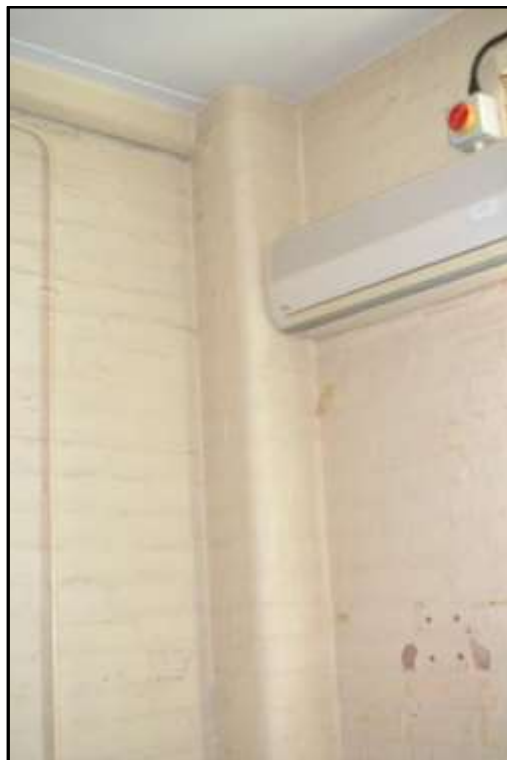
Plate D36 – D Block, spur 5, rounded edge of brick column typical within the individual rooms of each spur
