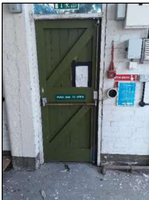
Plate A51 – A Block, early boarded and braced door within the north east elevation of later addition to spur 4
