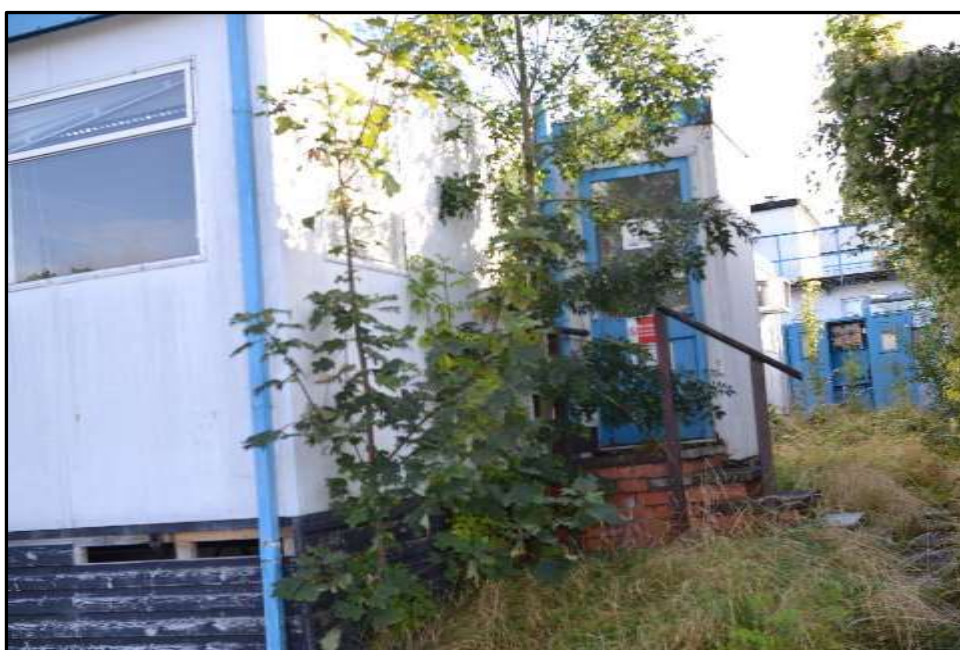
Plate E18 – E Block, part north elevation of central corridor range between spurs 2 and 4 with building 14 to centre and left
