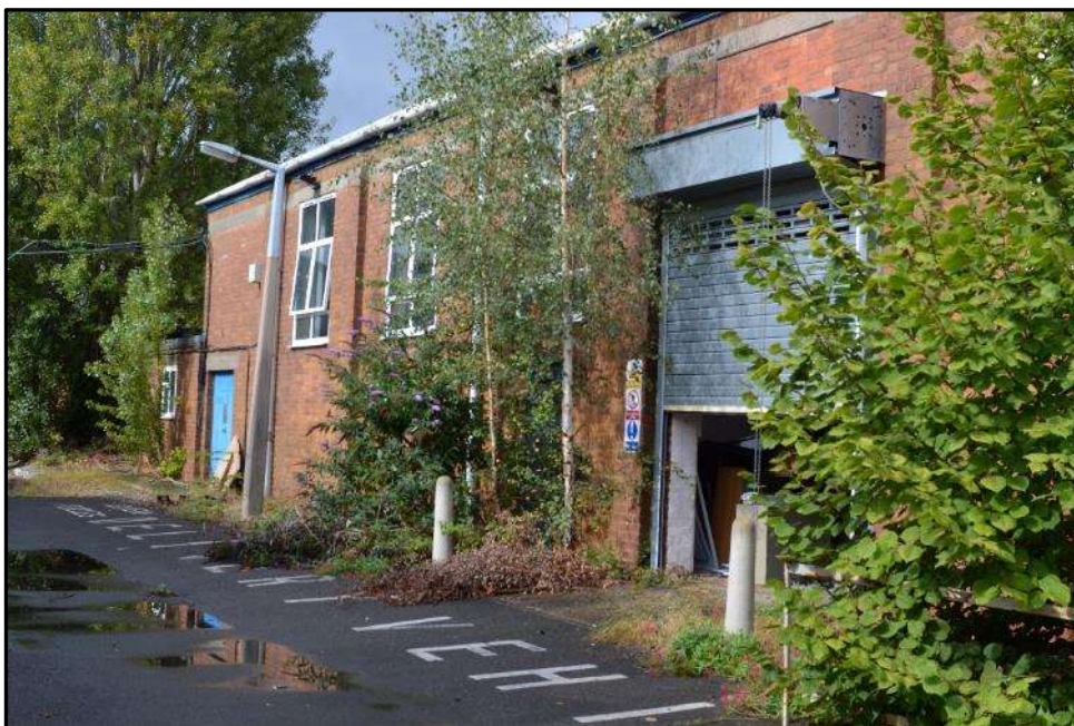
Plate 8h – Building 8, part south elevation of the south; not later alteration to create vehicle access
