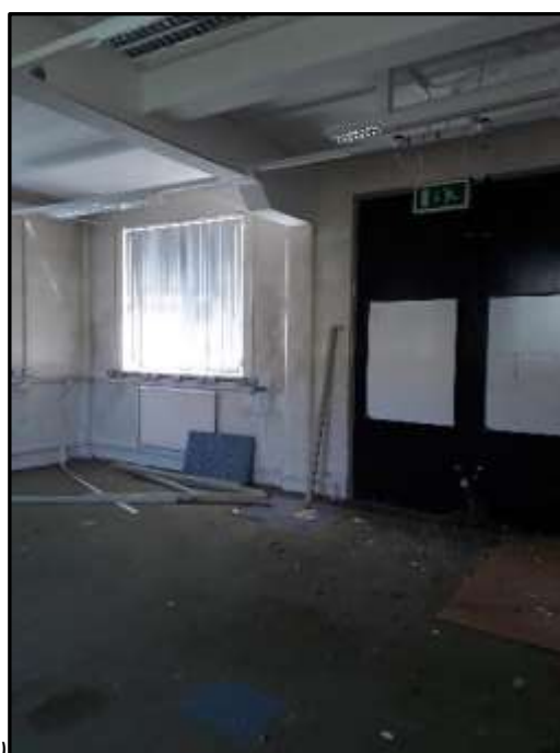
Plate A46 – A Block, interior of original boiler room space, subsequently adapted and used for research
