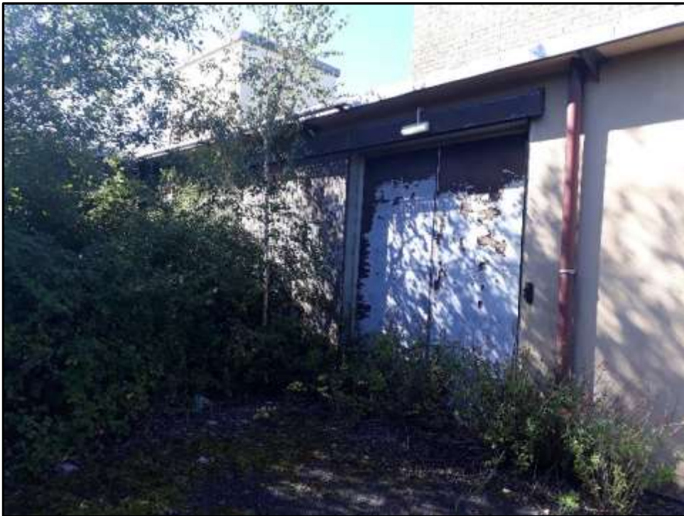
Plate A21 – A Block, enlarged entrance to south east elevation of original boiler house range
