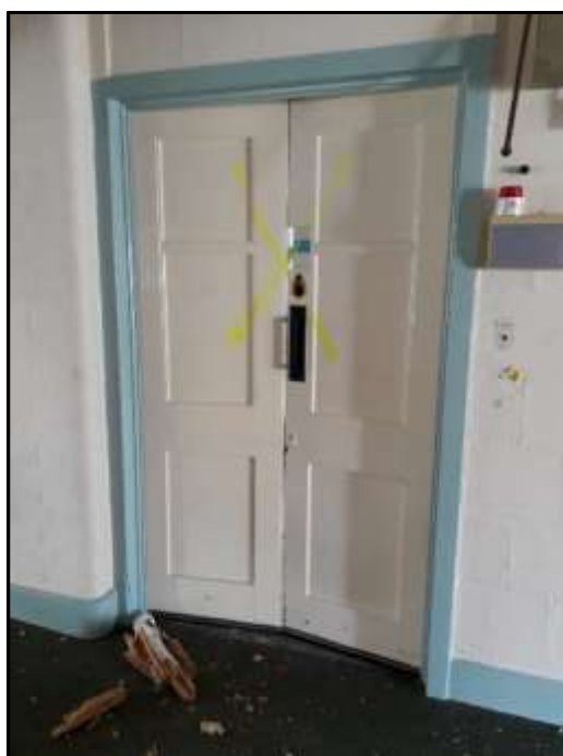
Plate E28– E Block, early/original double doors within internal north dividing wall in central corridor range between spurs 12 and 14
