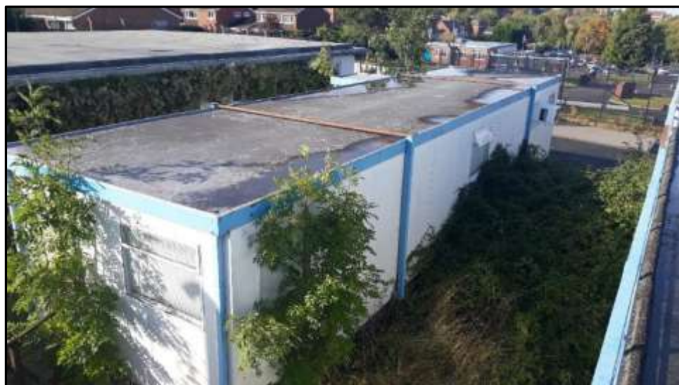
Plate 14d – Building 14, roof and east elevation viewed from roof of E Block
