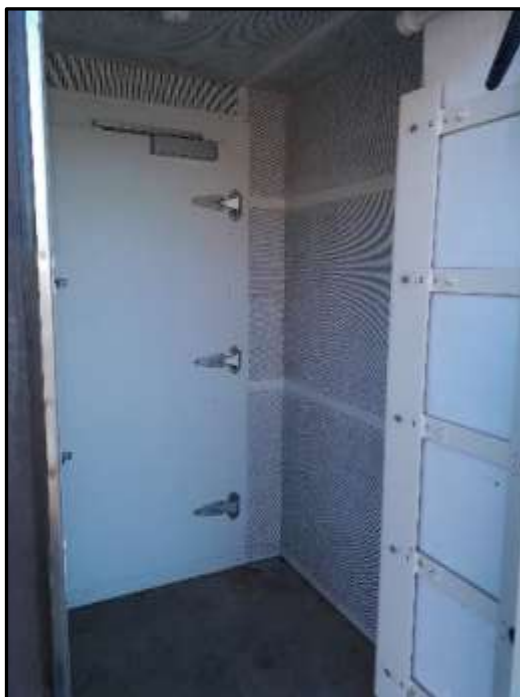
Plate H21 – H Building, external opening in north elevation into internal porch of second floor area of the former bunker
