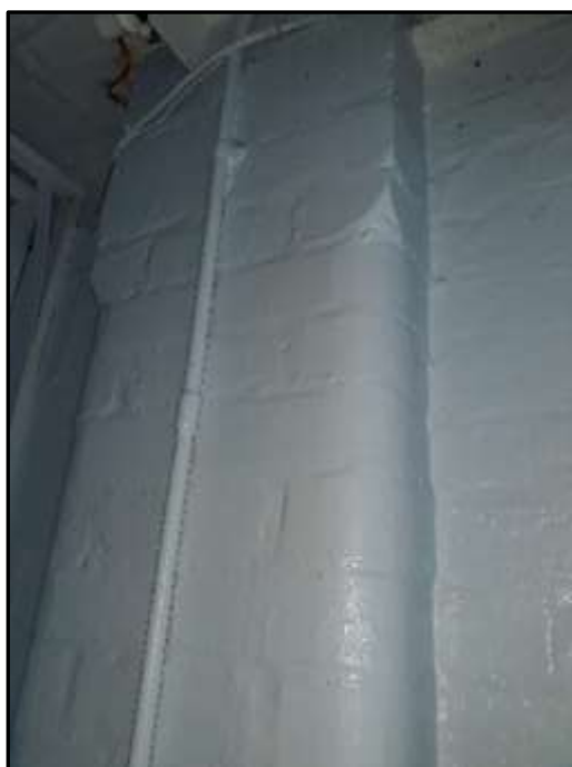
Plate A31 – A Block, rounded edge of structural brick column with stop chamfers, typical feature of the corridors
