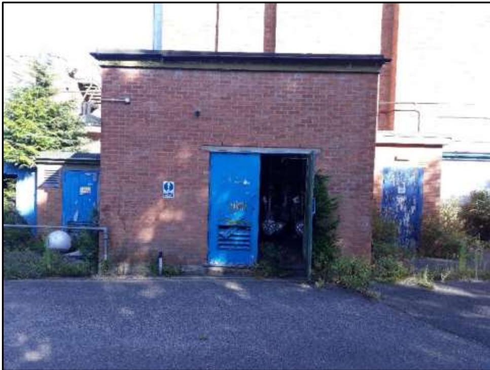
Plate H7 – H Building, later addition to the west elevation of the former bunker
