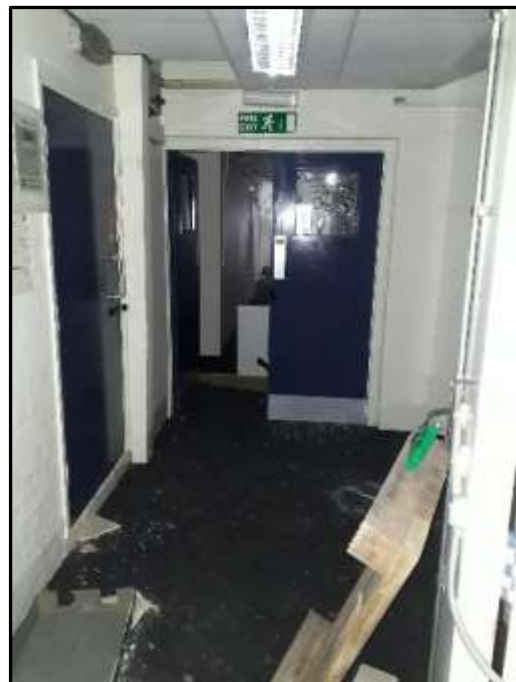
Plate H38 – H Building, ground floor corridor within the south range which retains its original proportions in part
