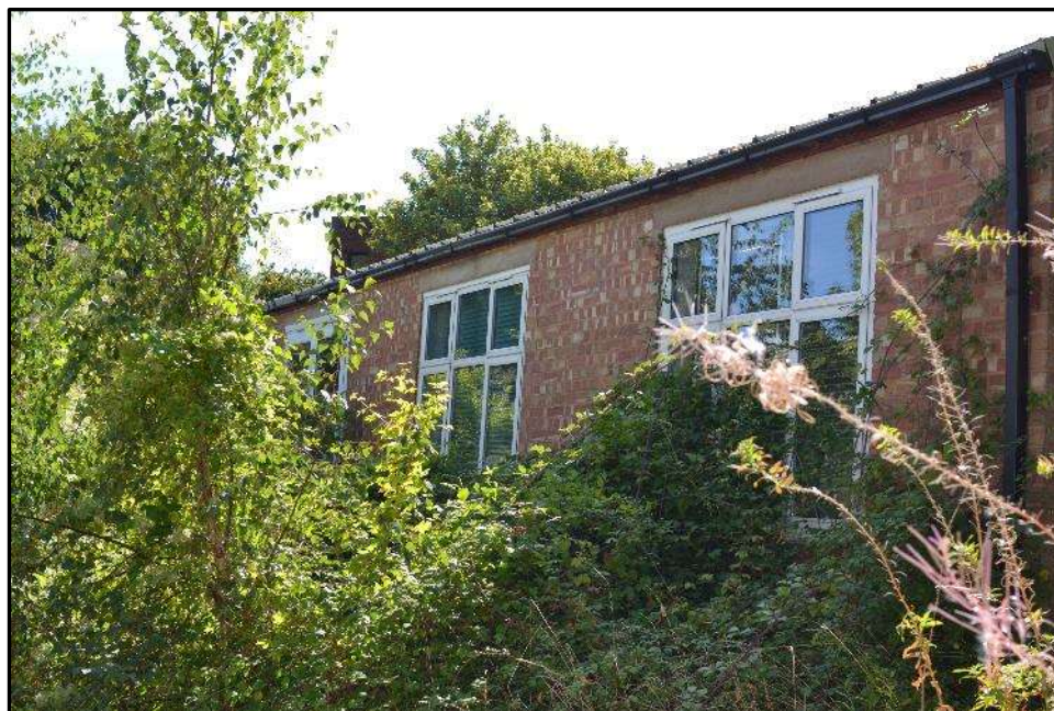
Plate L6 – Library building, north east elevation of the later south west range, opposing elevation to the inner facing south west elevation of the north east range
