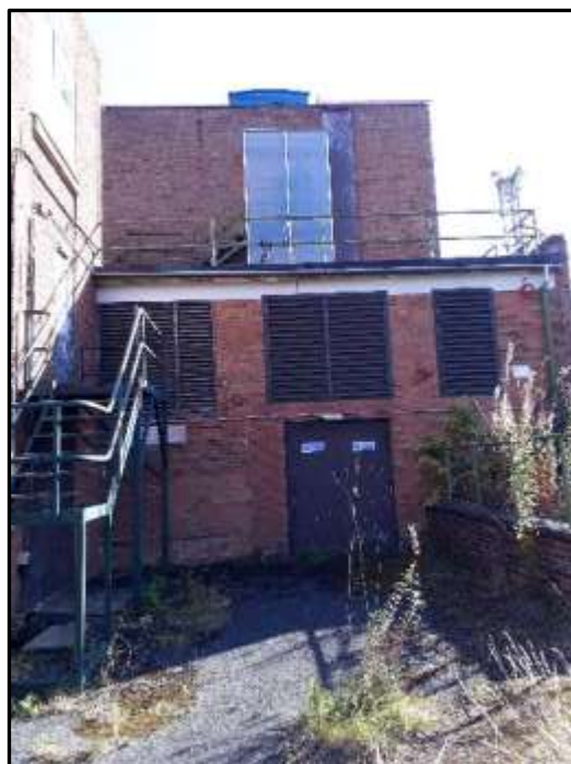
Plate H10 – H Building, west elevation of plant room and former bunker
