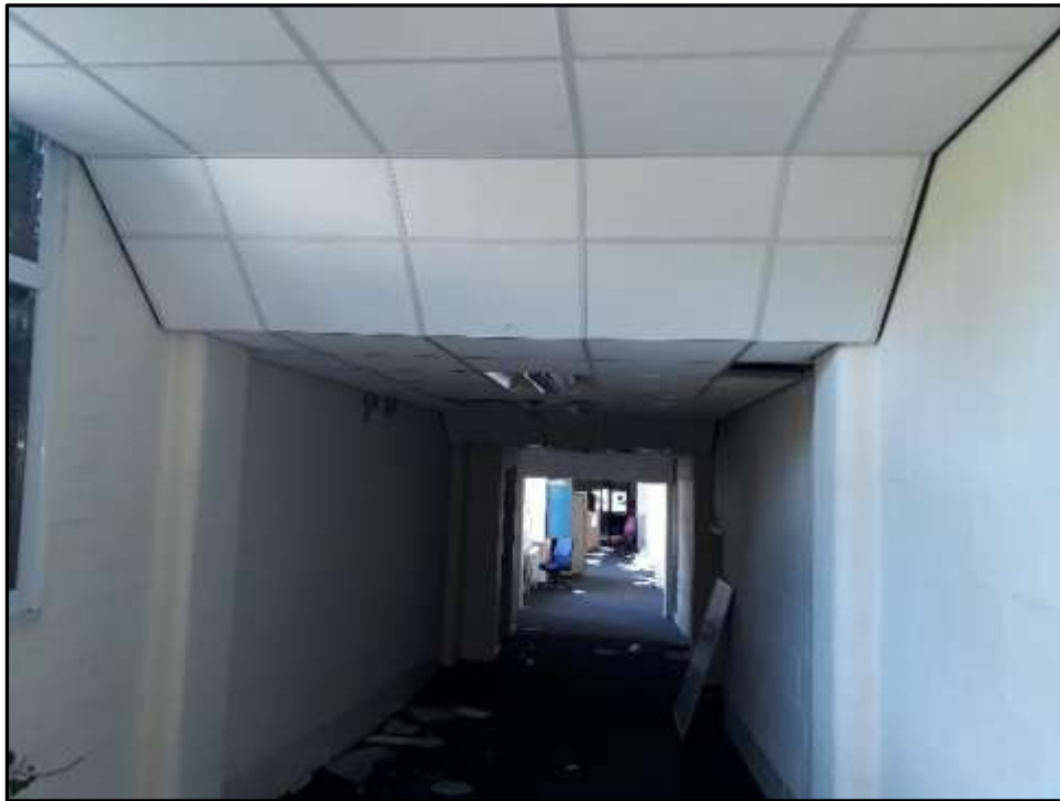
Plate D31 – D Block, central corridor looking east from central lobby area. Note inserted ceiling to conceal ducts and services and rounded edges of brick columns and brick tile internal walls to the right
