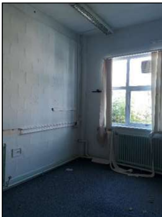
Plate A54 – A Block, brick tile internal wall and rounded corner of brick column evident of early method of subdivision observed within spur 1
