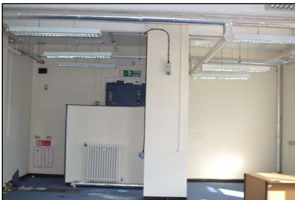
Plate D45– D Block, former boiler house within the south projection between spurs 3 and 5
