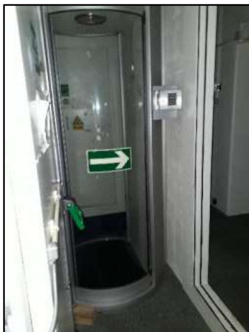
Plate H52 – H Building, first-floor level. Security pod to access the first-floor space; opening to right leads to a small lobby area where opening in the south wall of bunker leads to the first floor of the south range
