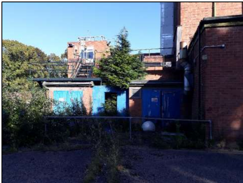
Plate H8 – H Building, plant room additions to the north west corner
