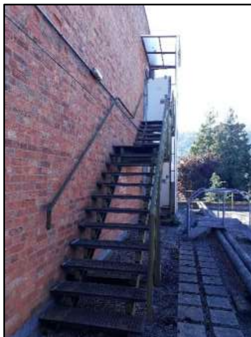
Plate H20 –H Building, external metal stair leading to the second-floor area of the former bunker
