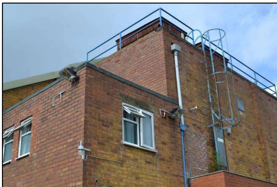
Plate 8e – Building 8, upper storeys of the east elevation of the south range
