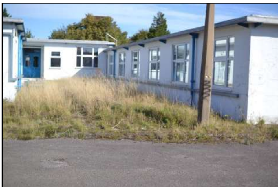
Plate D22 – D Block, south entrance to corridor range and west elevation of spur 3
