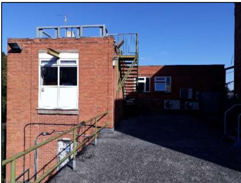
Plate H18 – H Building, west elevation of the first extension to the north
