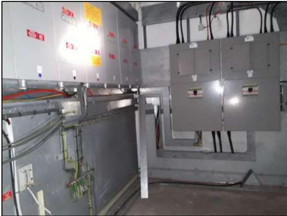
Plate H45 – H Building, north east corner of the ground floor showing the extent of electrical equipment and its projection within metal faraday caging
