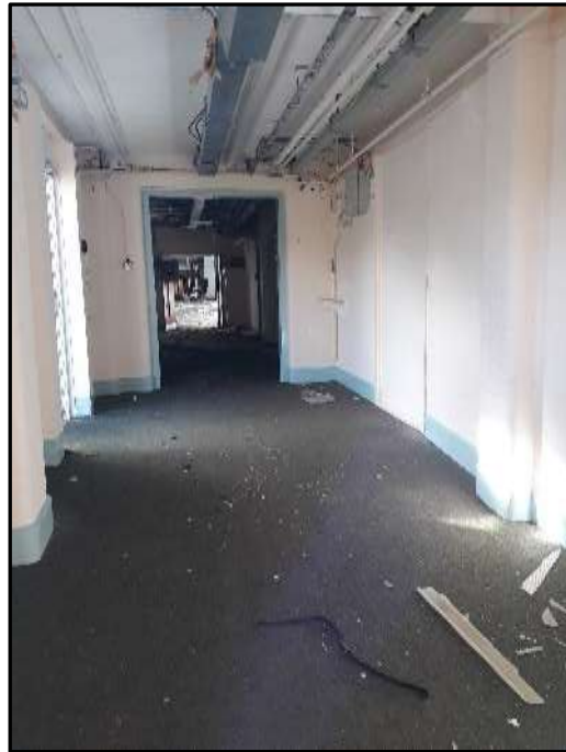
Plate E31 – E Block, view west along central corridor range from outside spurs 13 and 14
