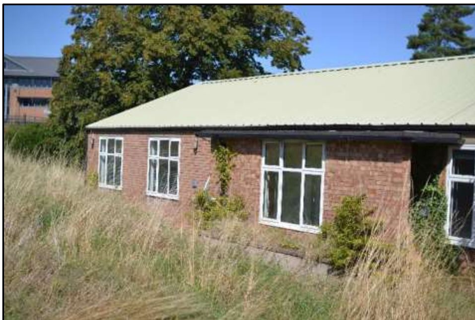
Plate L9 – Library building, part south west elevation of later south west range with central, projecting flat roof entrance porch
