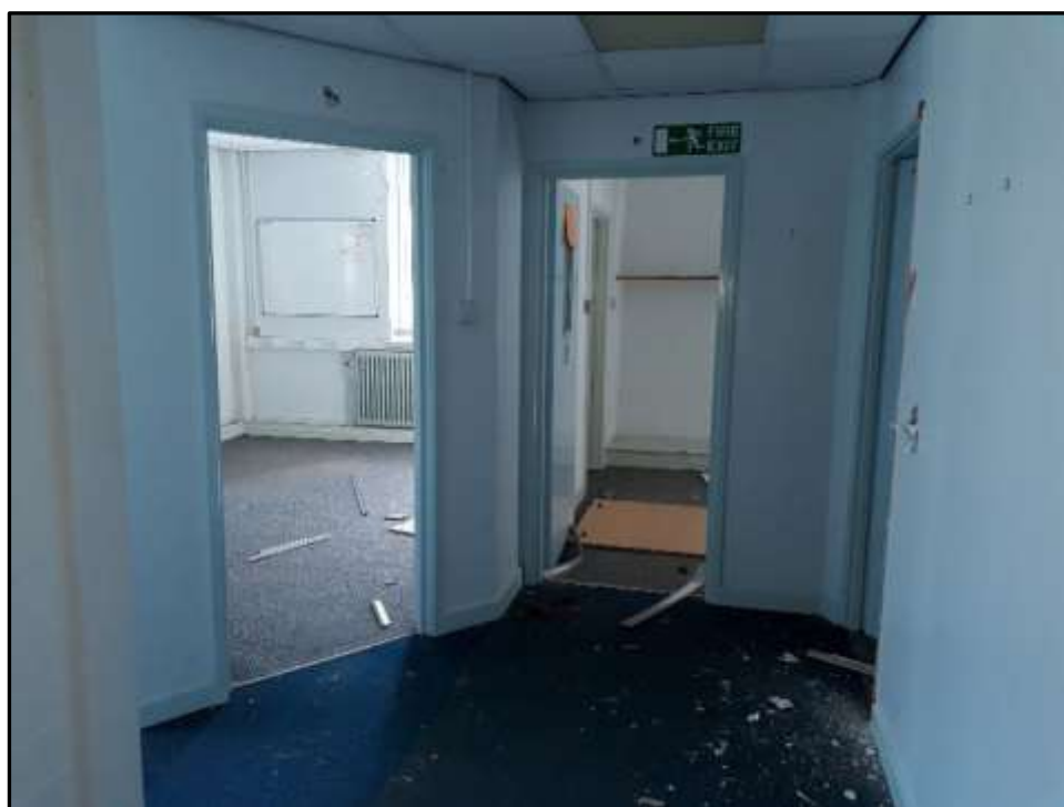
Plate A37 – A Block, south western extent of spur 5 with altered configuration of rooms
