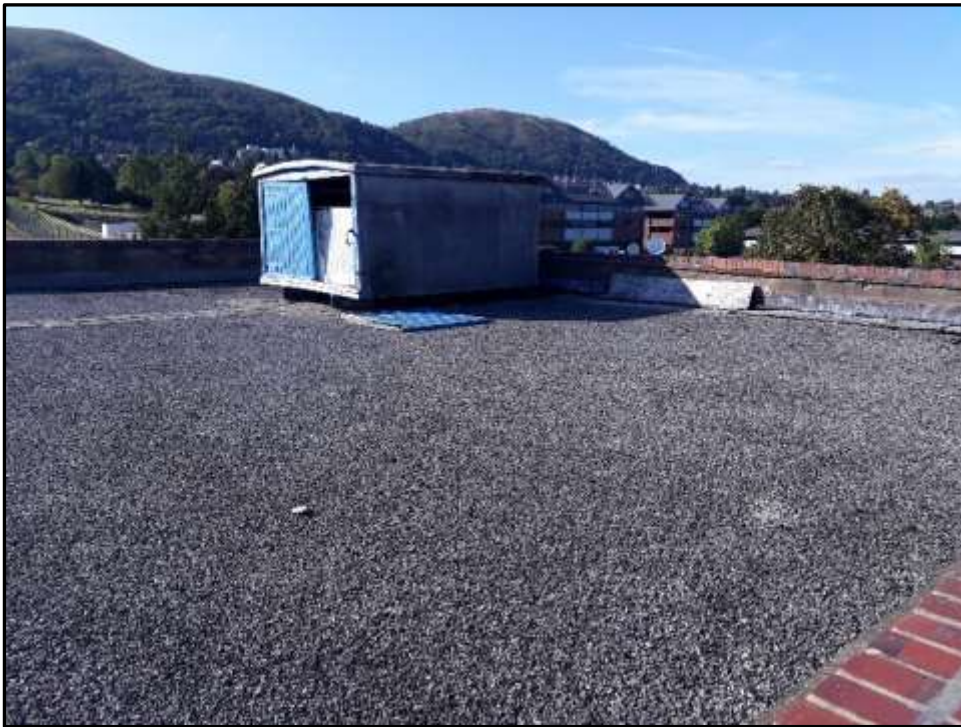
Plate H25 – H Building, north west area of the roof of the former bunker
