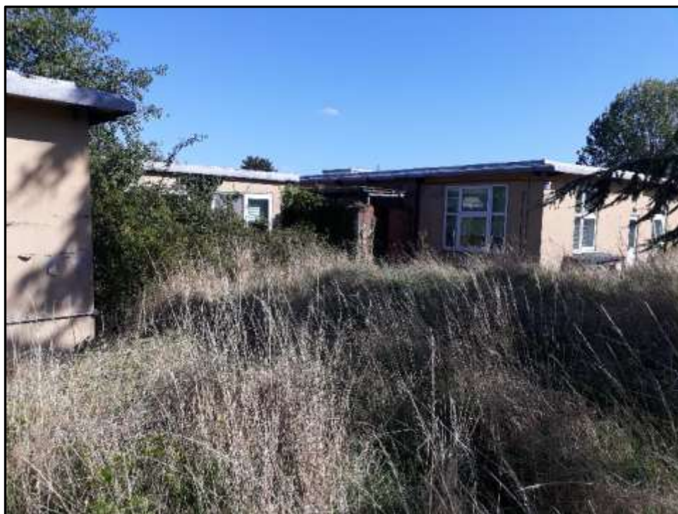
Plate A26 – A Block, part north west elevation of spur 3 with infill addition connecting spur 3 to spur 1
