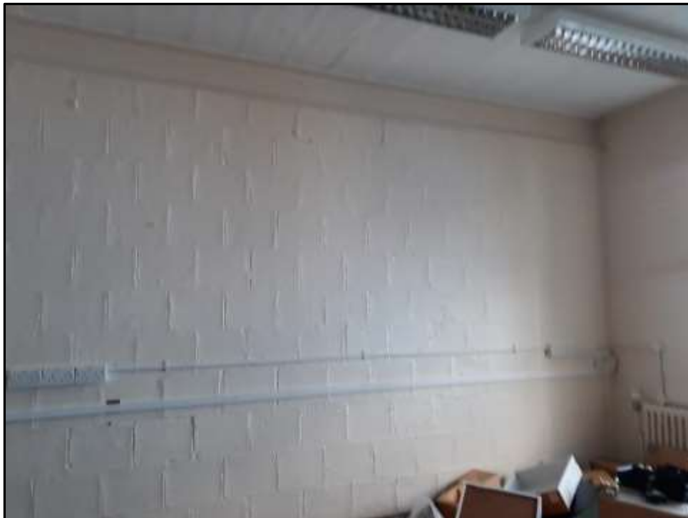
Plate E40 – E Block, brick tile internal dividing construction typical of the interior of the block
