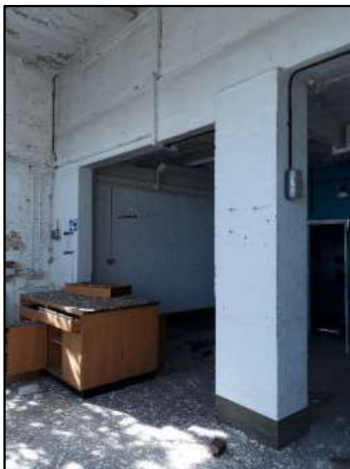
Plate A49 – A Block, interior of later addition to the south east elevation of spur 4, extent of original external wall of spur 4 in line with the brick piers
