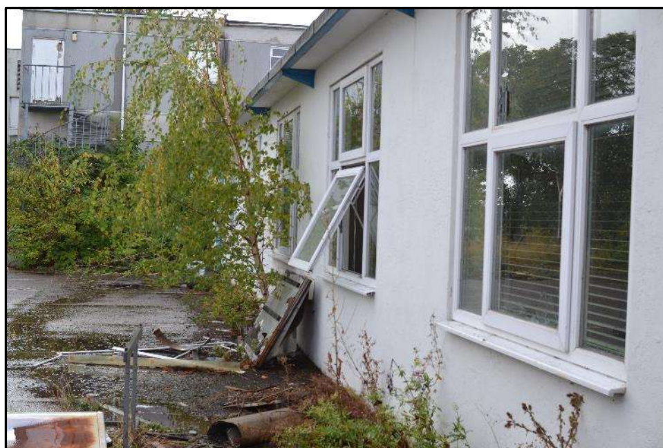
Plate E6 – E Block, east elevation of spur 7 with ET Block (building 15) in the background
