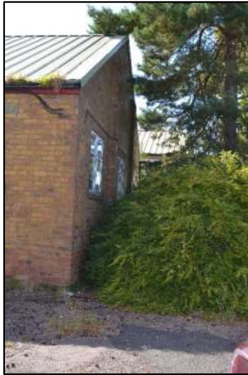
Plate L3– Library building, part north west end elevation of north east (original) range
