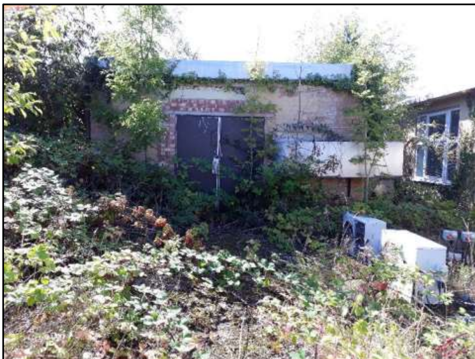
Plate A15 – A Block, north east end elevation of shorter projection between spurs 8 (left) and 6 (right)
