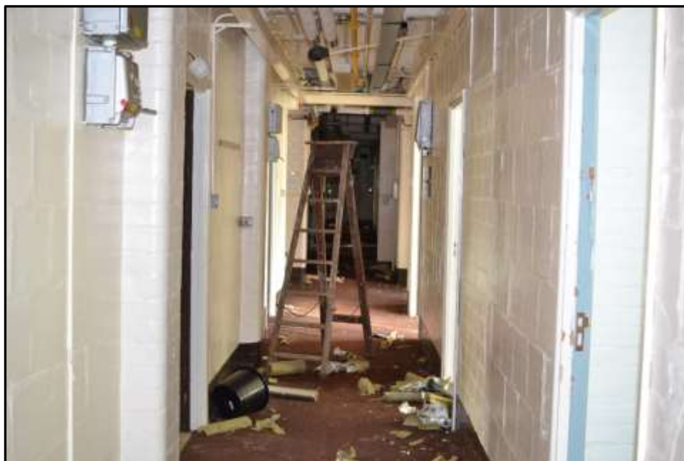
Plate KF9 – Central corridor (looking into southern half), brick tile internal dividing walls and rounded edge of brick columns visible
