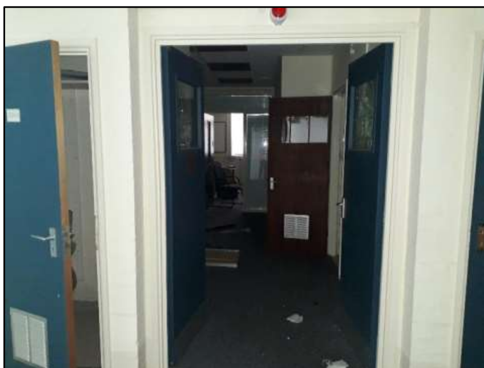
Plate D50 – D Block, view north into original morgue area, now reconfigured as offices
