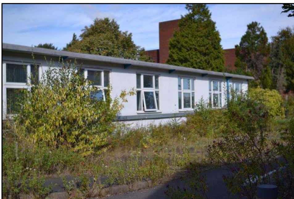
Plate D14 – D Block, east elevation of spur 2 (typical window arrangement presented)
