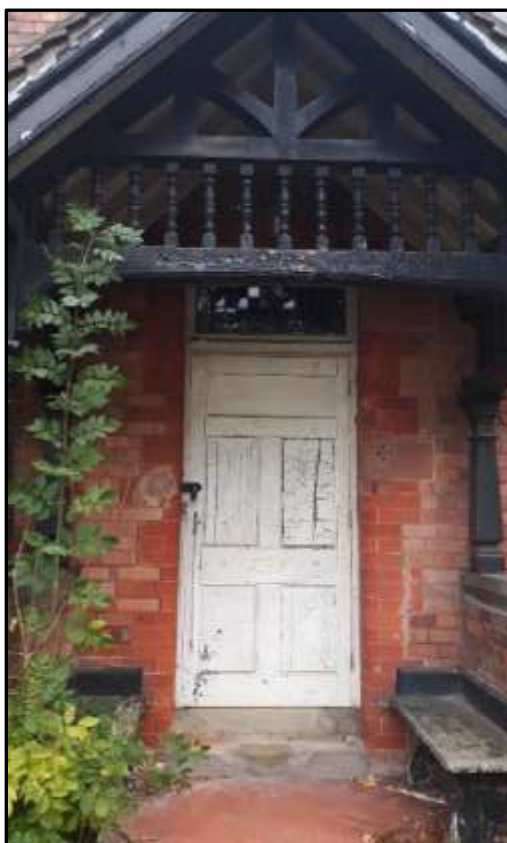
Plate S14 – Block S, main entrance door into the central range; note gauged brickwork jambs and decorative fanlight
