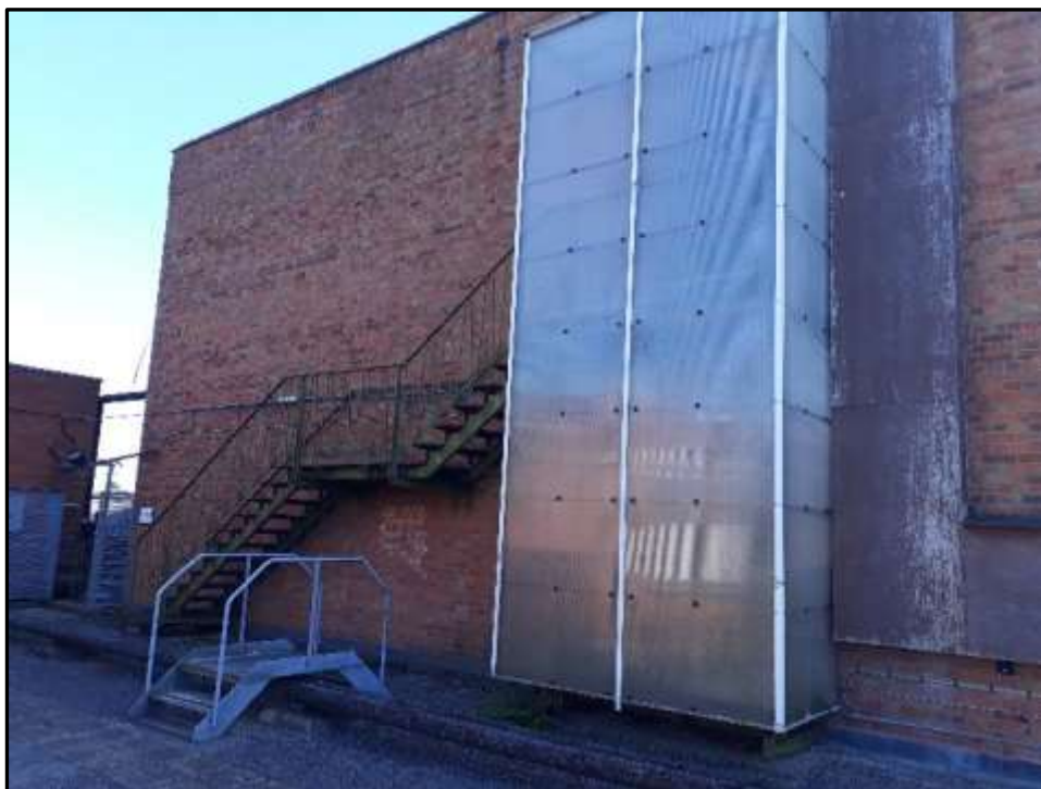
Plate H19 – H Building, enclosed first and second floor exits and metal external stair to the north elevation of the former bunker
