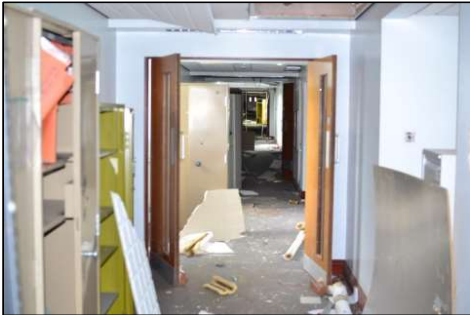
Plate E41 – E Block, view west along central corridor from main entrance; section of corridor has been subject to alteration to stud partition walls and new ceiling altering the original the original proportions
