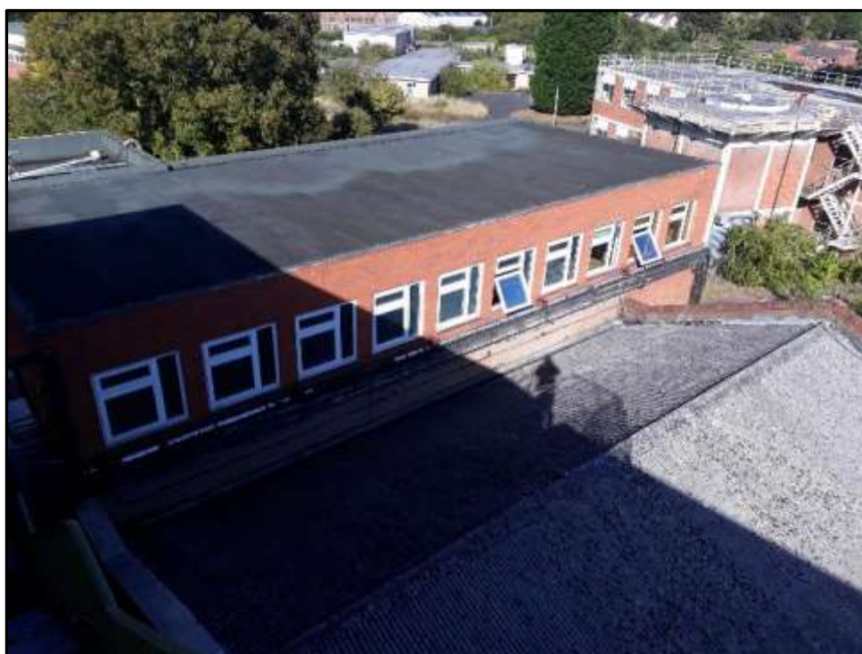
Plate H23 – H Building, south elevation of the first floor addition to the north range
