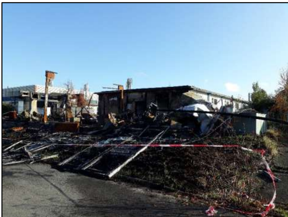
Plate E13 – E Block, north end elevation of spur 12 where previously addition has been destroyed by recent fire
