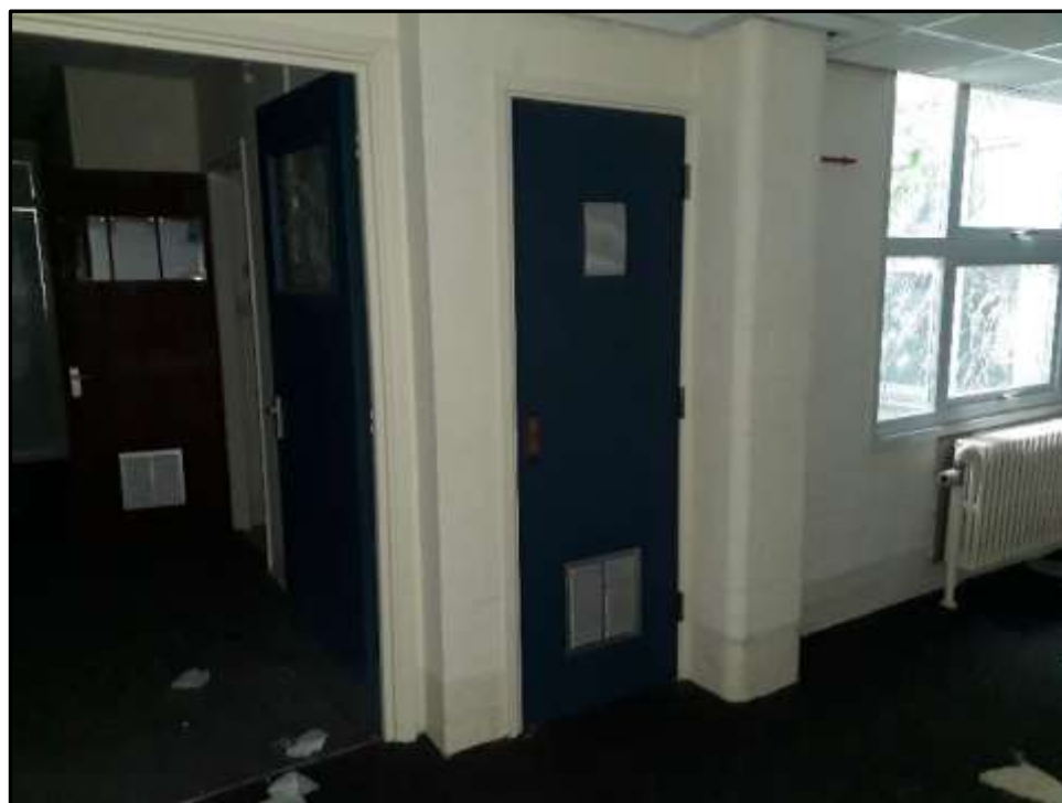
Plate D34 – D Block, arrangement of openings and brick column where the corridor leads into the north projection between spurs 8 and 6 which was originally the morgue
