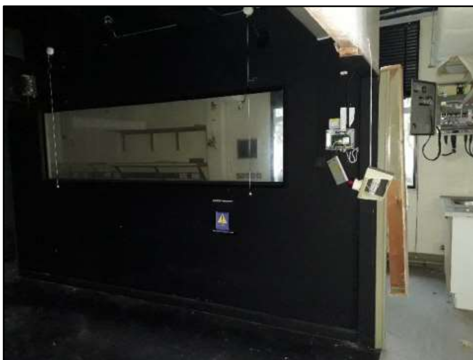
Plate A50 – A Block, Remains of fixture and fittings to laboratory space in spur 1
