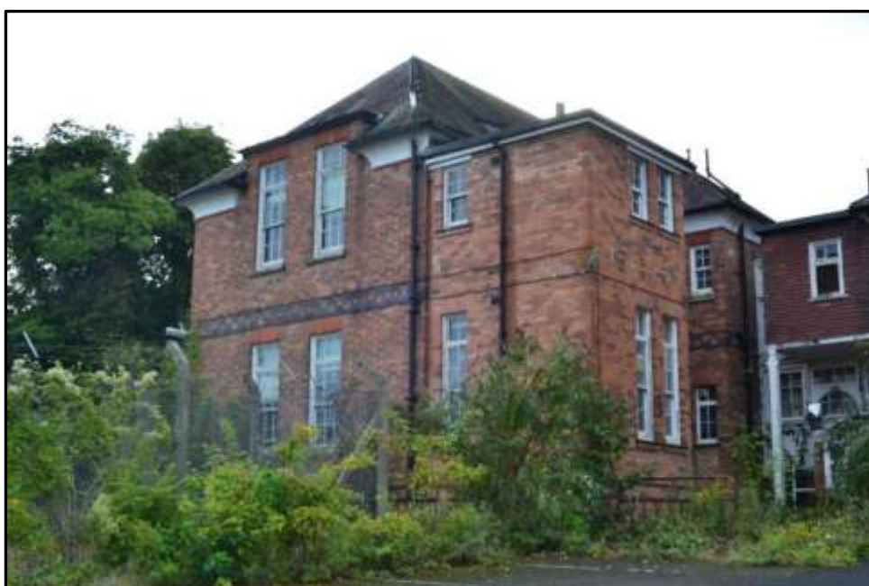
Plate S4 – Block S, east elevation of the southern range; note later two storey extension to the right of the main range
