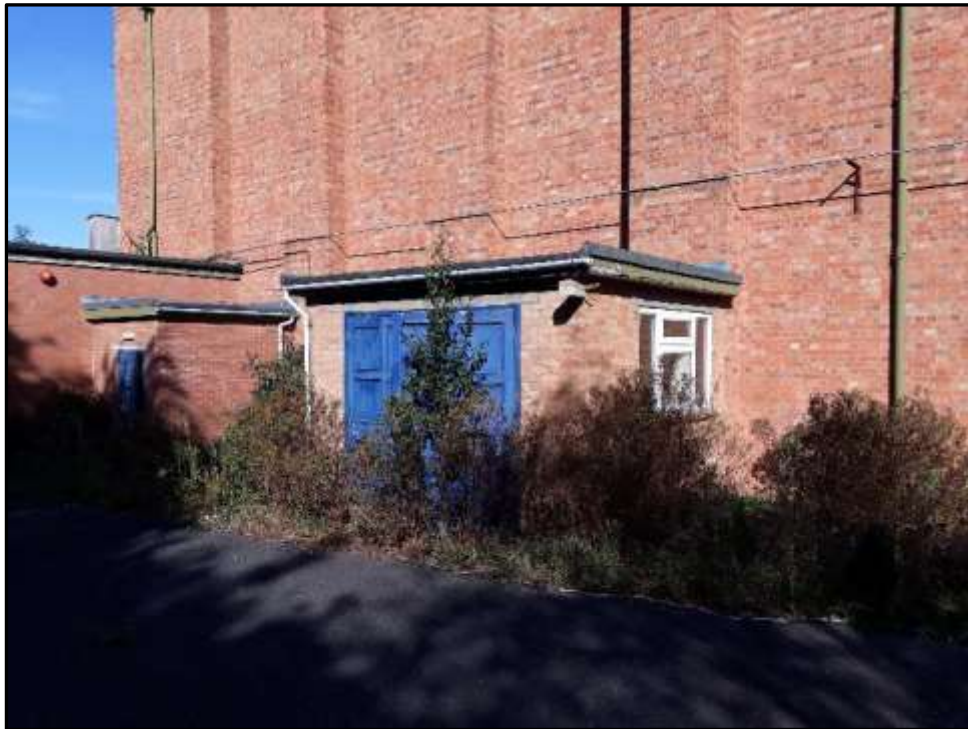
Plate H5 – H Building, later addition to west elevation of former bunker
