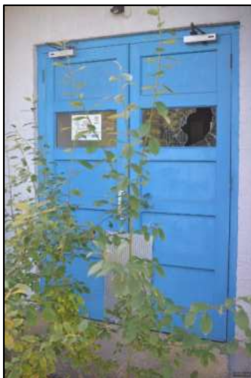
Plate D9 – D Block, timber doors to main entrance from the north
