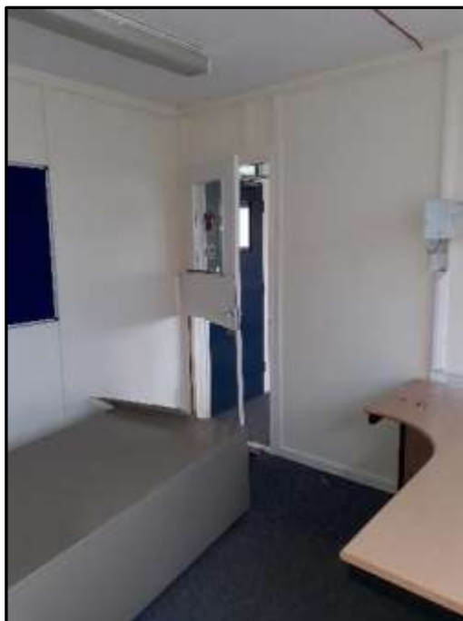
Plate H31 – H Building, typical appearance of the first floor office to north range
