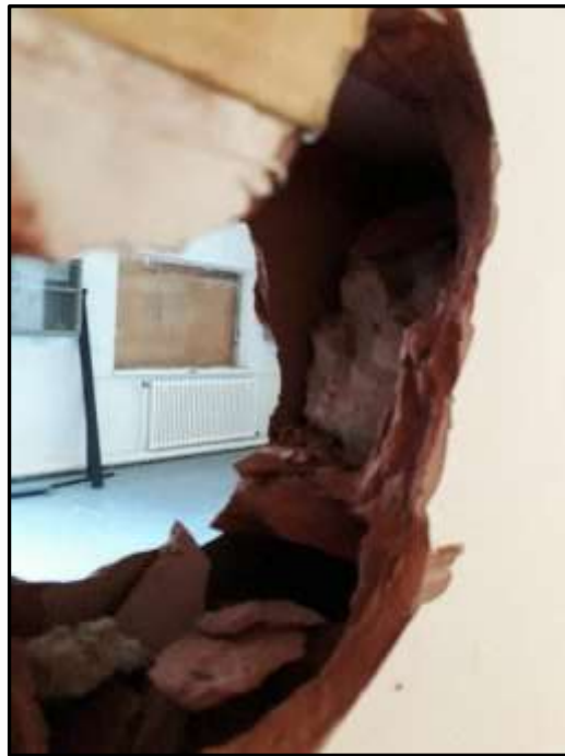
Plate E29 – E Block, hole in partition wall exposing brick tile construction typical to the internal walls within the original WWII blocks
