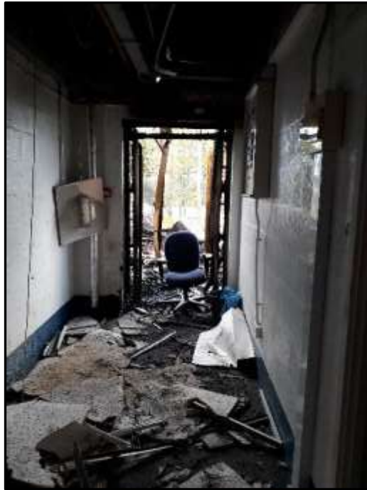
Plate E39 – E Block, view north along spur 12 which has been damaged by recent fire
