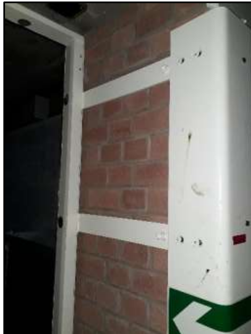
Plate H48 – H Building, depth of external blast walls to the former bunker area
