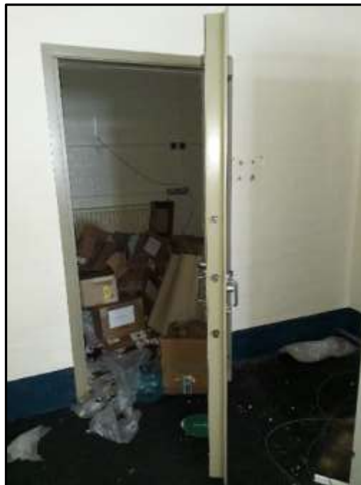
Plate D48 – D Block, secure document store roof to the most southern bay of spur 5
