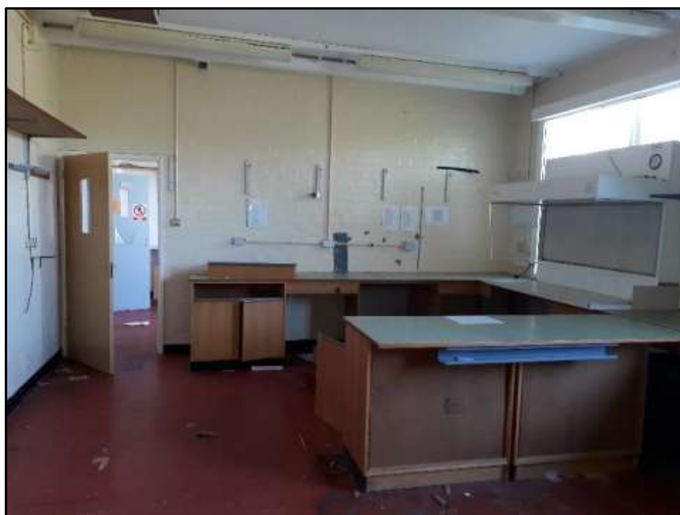
Plate A41 – A Block, fixtures associated with laboratory use observed in spur 4
