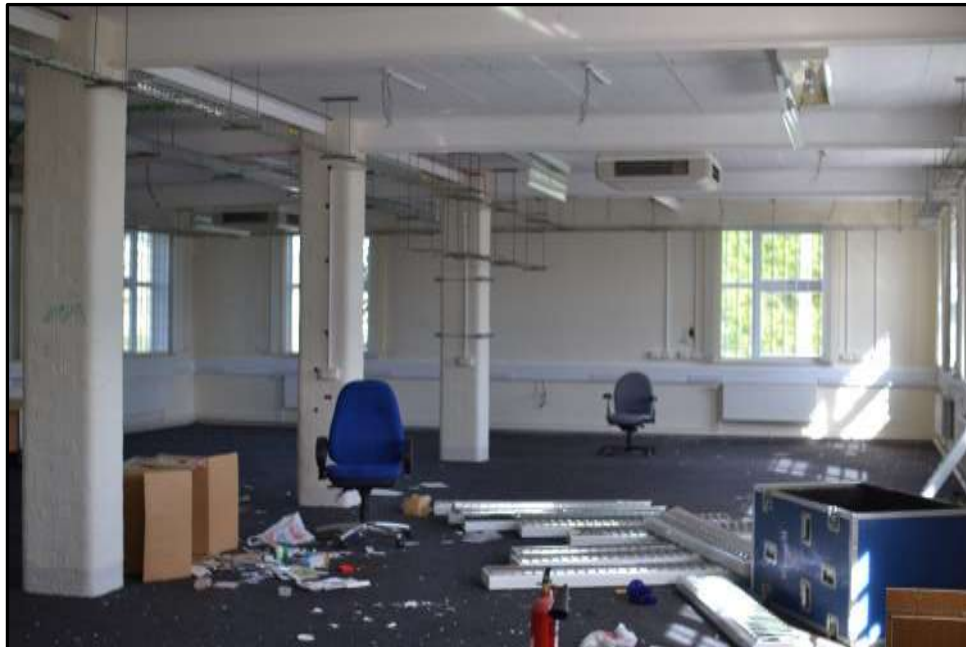
Plate D40 – D Block, spur 6. Open plan arrangement with structural brick columns of the original construction method to centre of the room
