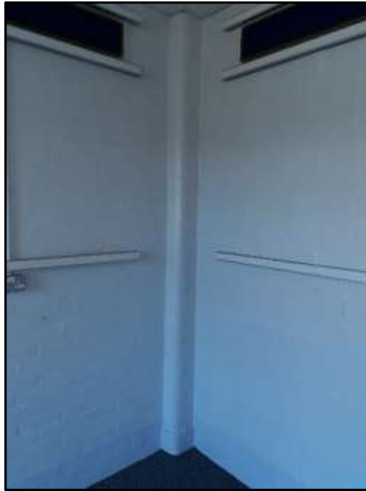
Plate A33 – A Block, corner of the structural brick column typical of interior rooms to the spurs
