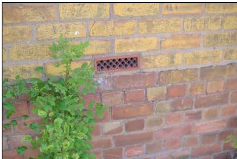
Plate L16 – Library building, north east elevation of the original range. Change in brickwork and coursing indicative of alteration or rebuilding, possibly contemporary with the later addition of the south west range
