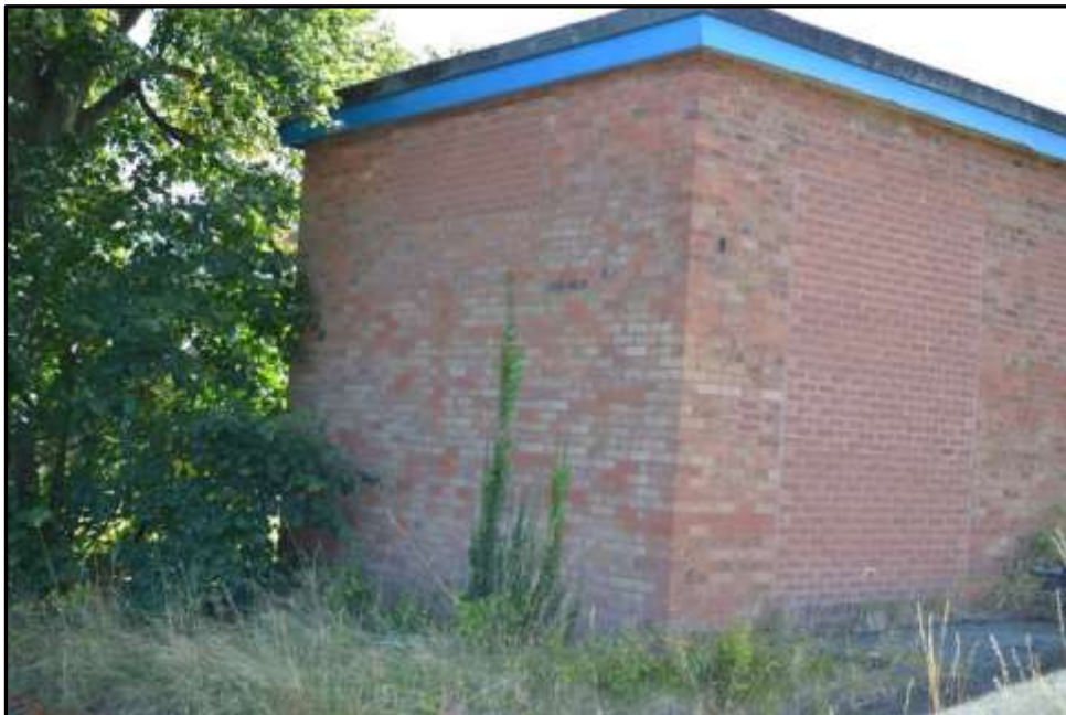
Plate 22c – Building 22, part west and north elevations west elevation; note blocked former openings
