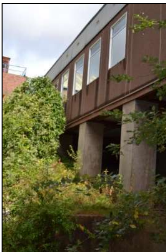
Plate 10d – Building 10, concrete pillars supporting first floor element (viewed from the south west)
