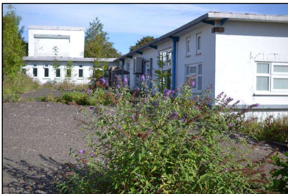
Plate D26 – D Block, central corridor range between spurs 5 and 7 and west elevation of spur 5; nota altered pattern of windows to corridor range
