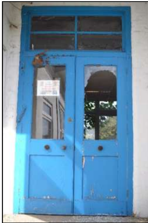
Plate D29 – D Block, timber entrance doors to south entrance between spurs 3 and 5
