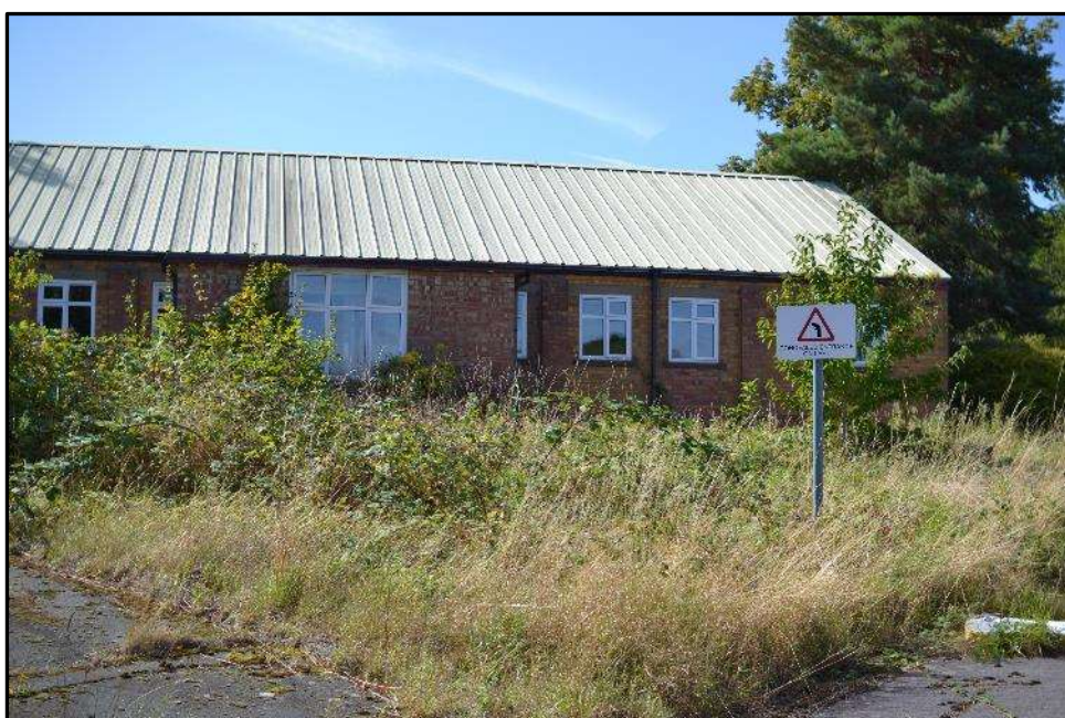
Plate L2 – Library building, part north east elevation of north east range (original section)
