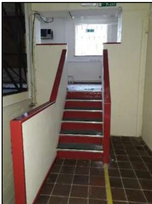
Plate H35 – H Building, ground floor of the north range; steps lead up to battery room extension
