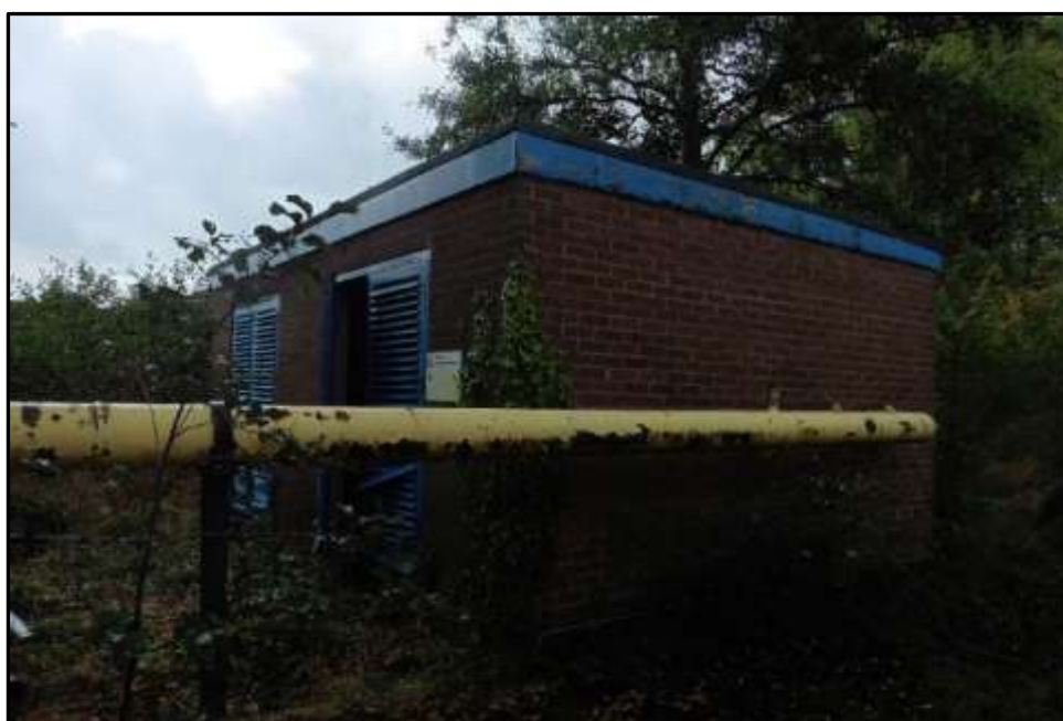
Plate 20d – Building 20, north elevation and part east elevation with gas pipe entering the north elevation
