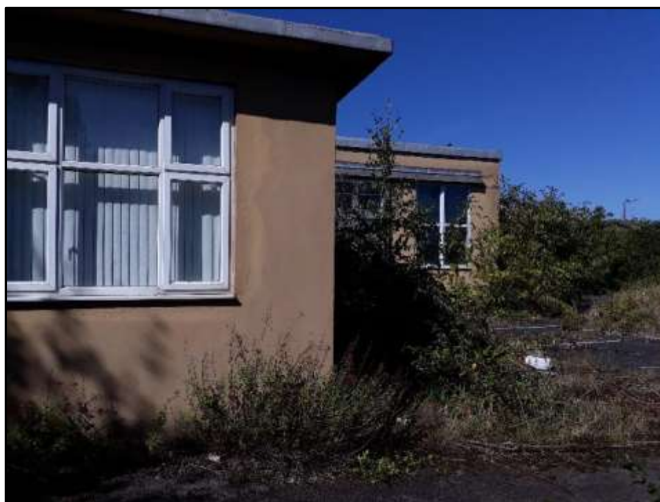
Plate A20 – A Block, part south east elevation of later addition to spur 4 (centre) and part south east elevation of former boiler house (left) positioned to oppose the central entrance
