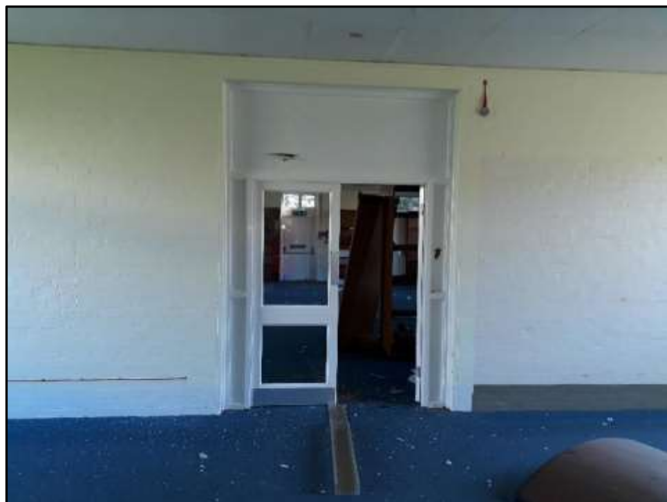
Plate L28– Library building, south west range. Doors lead into a later addition added to the south east end of the south west range
