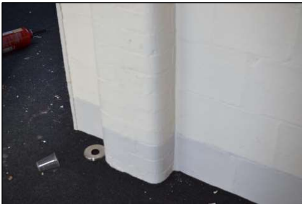
Plate D37 – D Block, typical detail of rounded brick columns as exposed to the main central corridor and the secondary spur corridors
