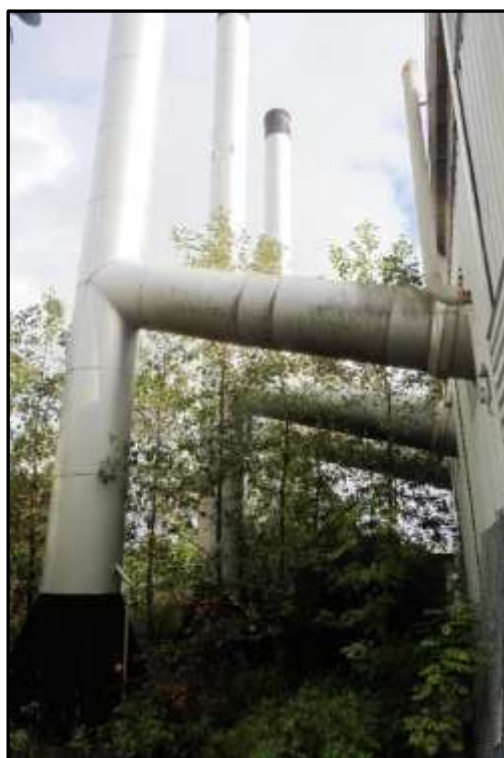
Plate 19c – Building 19, external flues to the main boilers (north elevation)
