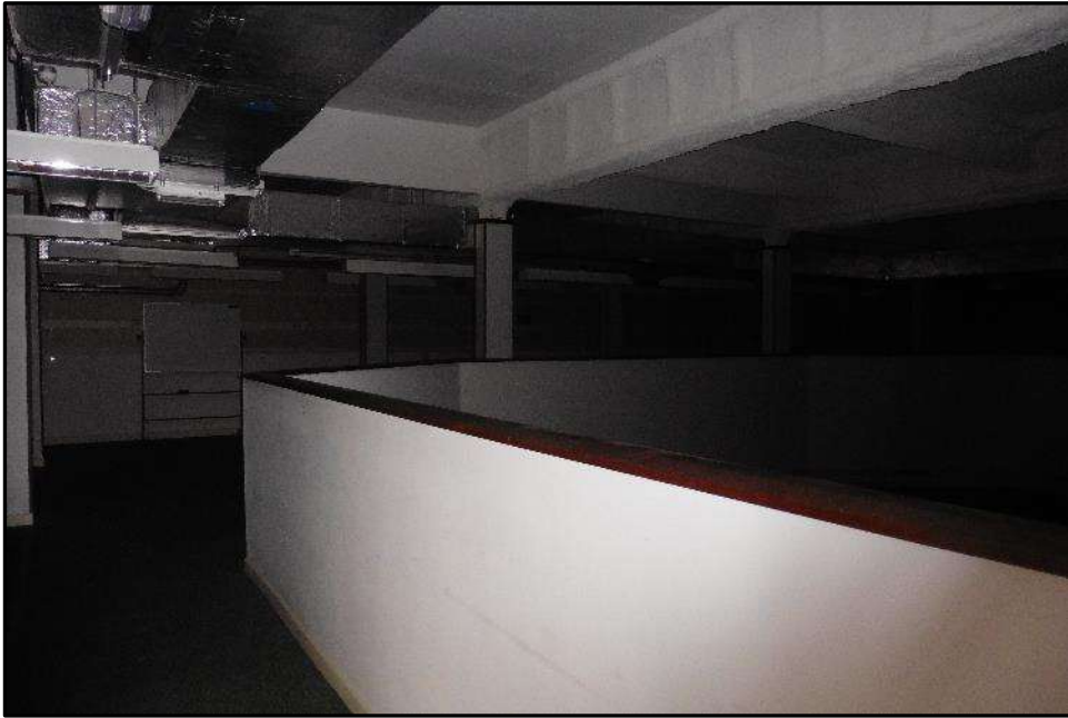
Plate H57 – H Building, second floor. View across the second floor mezzanine level. This configuration is the only obvious remains of the original R4 bunker configuration. Metal joists have been coated with an intumescent covering to metal structural steels. Original floors of the R4 bunker were hung from these joists
