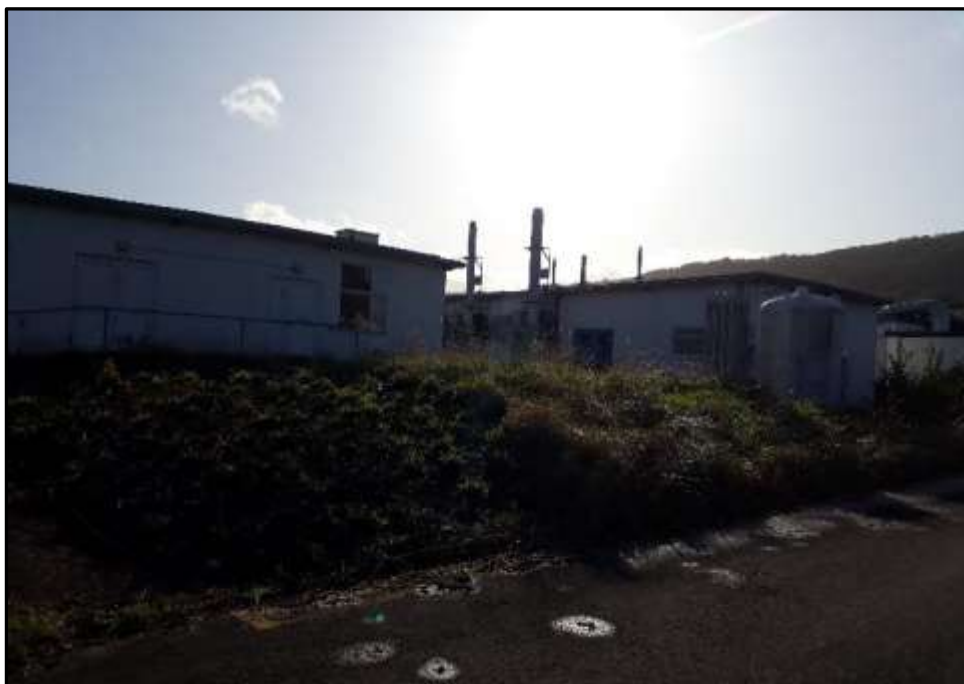
Plate E15 – E Block, part north end elevation of spur 10 and north end and part east elevation of spur 8
