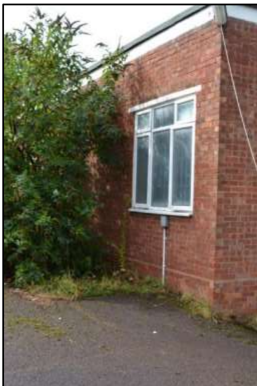
Plate 36j – Building 36, part south east elevation of single storey wing which formerly housed the centrifuge machine
