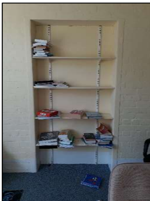
Plate D38 – D Block, blocked opening in spur 5. Brickwork internal walls indicate area of original air raid shelter, this function requirement more solid walls as opposed to the typical brick tile internal walls
