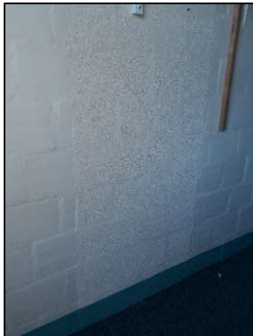
Plate A34 – A Block, evidence of a blocked doorway observed in spur 8
