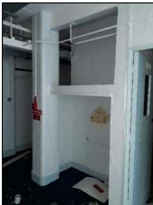
Plate A45 – Internal recess space, identified as being an original feature on the 1940 plan (see appendix 10), to main corridor range
