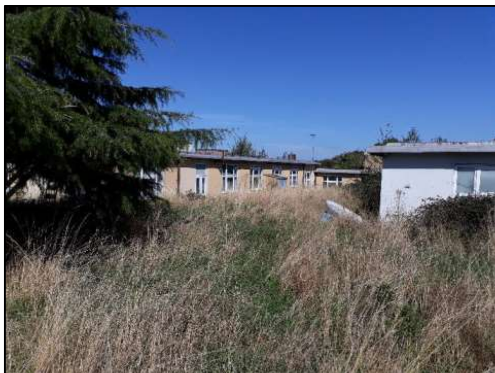
Plate A8 – A Block, south east elevation of spur 5 and part south west end elevation of spur 7
