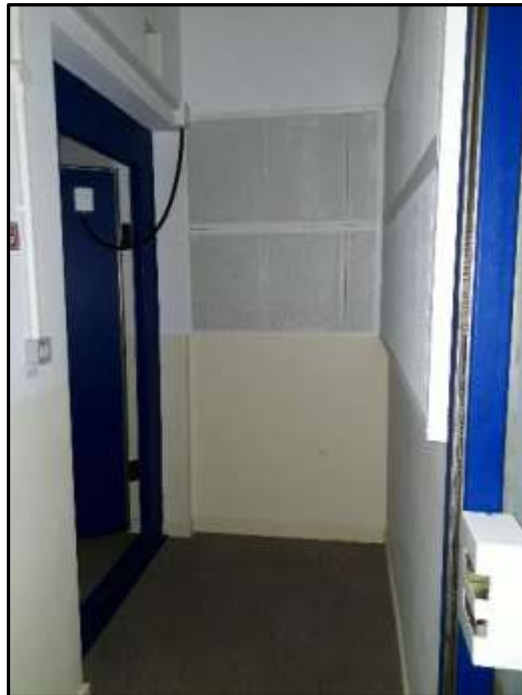
Plate H49 – H Building, ground floor. RF lock entry into the central faraday cage
