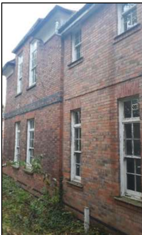
Plate S7 – Block S, west elevation of the south range; note extension to the right of the elevation
