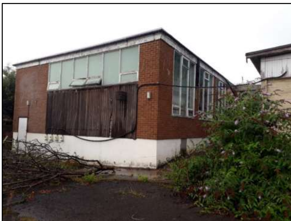
Plate 7c – Building 7, part north and east elevation of main L shape range; garage/store to right of image
