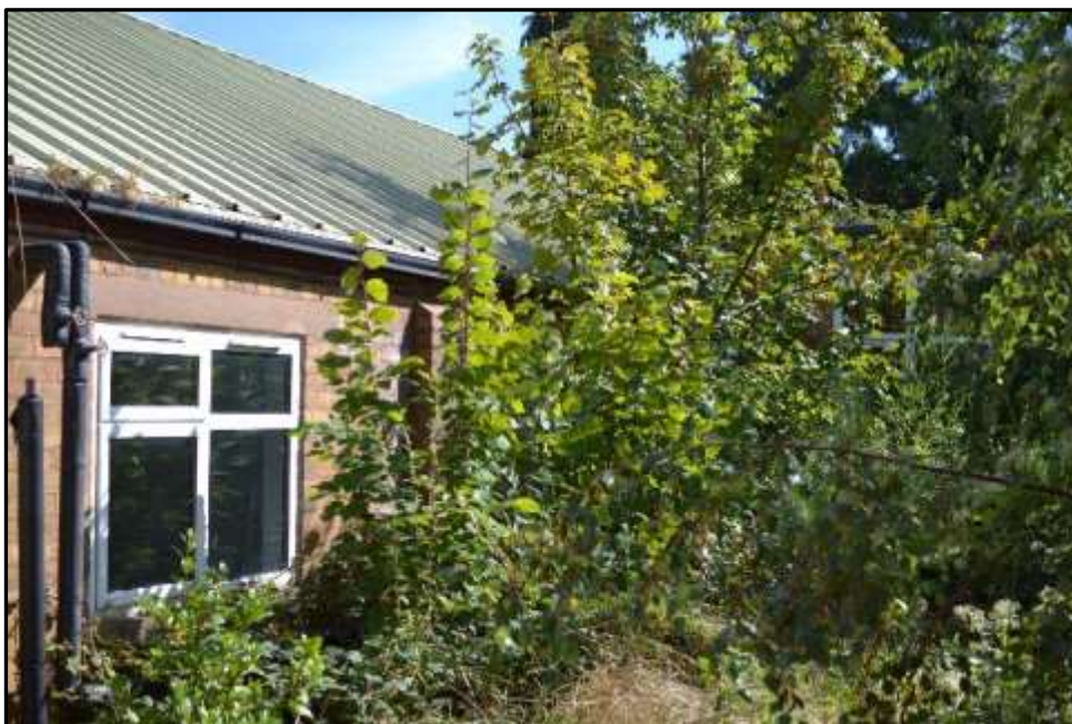
Plate L5 – Library building, part south west elevation of original range, now enclosed by the later south west range where its north east elevation opposes
