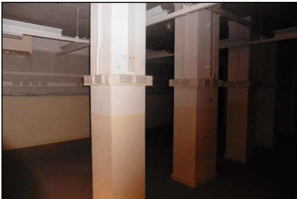
Plate H46– H Building, ground floor of former bunker. View of interior space within the faraday cage with 5 columns across centre, likely encasing service and duct work rather than being structural
