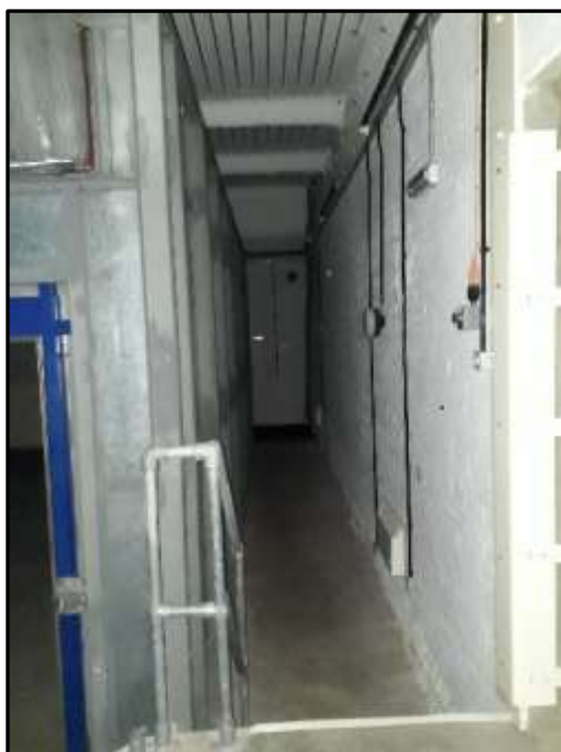
Plate H44 – H Building, view of the ground floor perimeter corridor of former bunker from the elevated lift platform in the north west corner; west external wall to right of image
