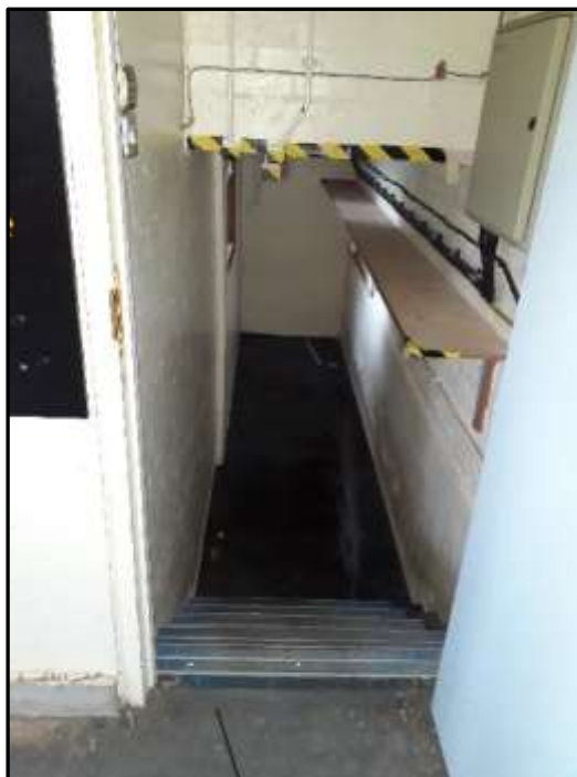
Plate H29 – H Building, lower ground floor level of battery room extension to the north
