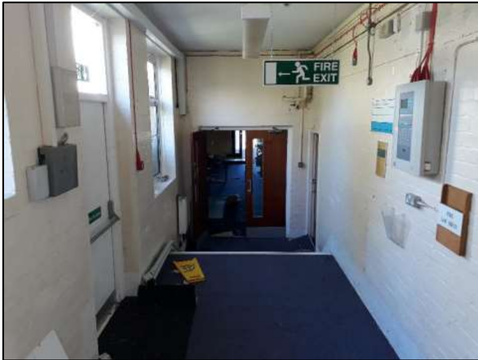
Plate L23 – Library building, link corridor with painted brickwork wall and steps to address changes in level between the two ranges (facing north east)
