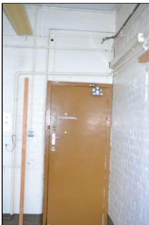
Plate KF20 – Door leading into the area which formerly housed TREAC; note the brickwork construction to the right (north) internal wall which depicts the use as a former air raid shelter
