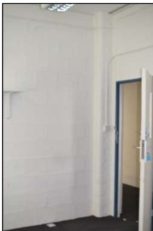
Plate D42 – D Block, spur 3. Typical internal arrangement of flanking rooms with rounded edge of brick column and brick tile internal walls
