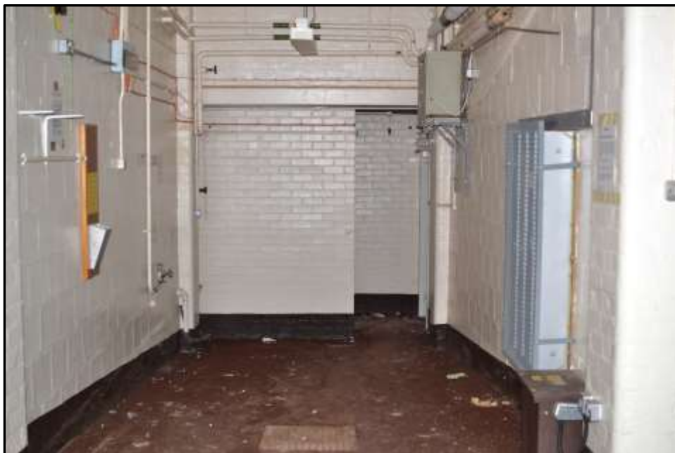
Plate KF14 – Brick infill work to modern extension where KF block was previously adjoined to F Block
