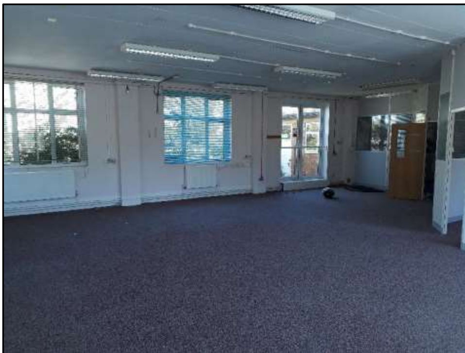
Plate L25 – Library building, south west range. Open plan space within the north west half of the range
