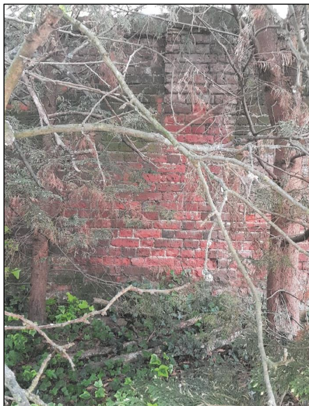
Plate 10: North boundary wall of No. 20 St James Way (Urban and Rural Ltd)
