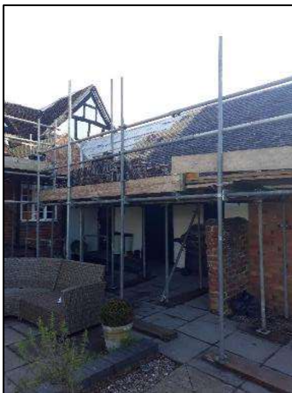
Plate MF24 – Covered walkway to north elevation of single storey west wing of south range
