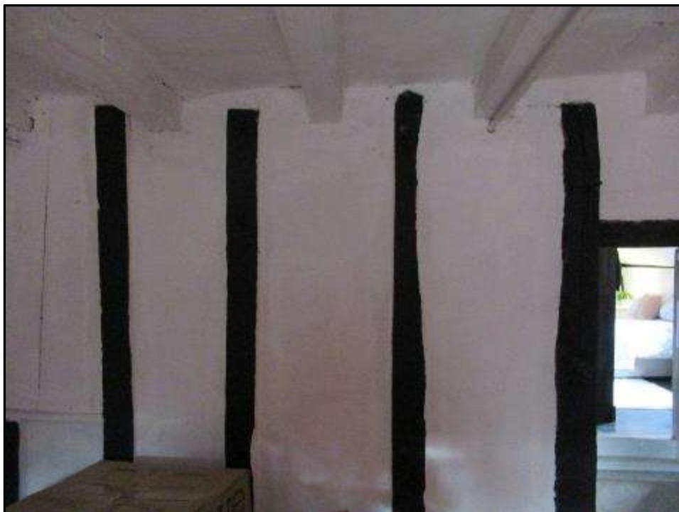
Plate MF138 – Close stud framing to the internal subdividing wall between the small first floor room and the first-floor landing area
