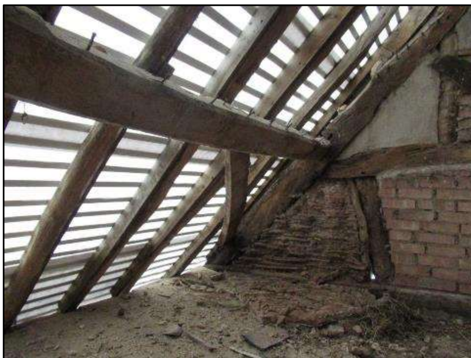
Plate MF146 – Clasped purlin and arched wind brace to south roof slope
