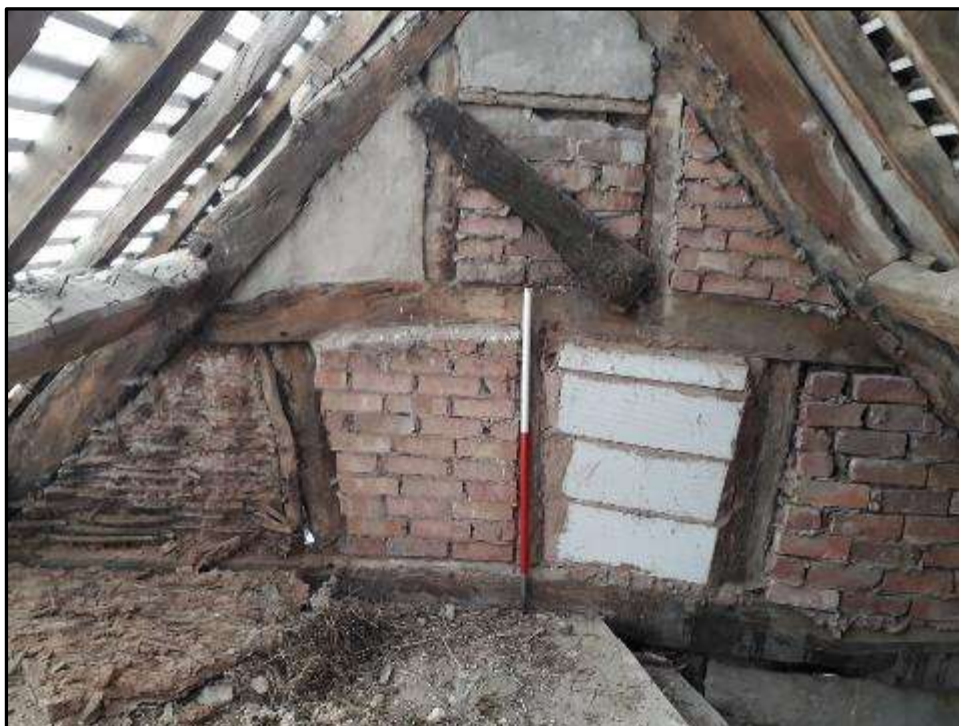
Plate MF145 – West gable end elevation of the south range with double queen post roof truss and original wattle and daub infill panels to the south (left side)
