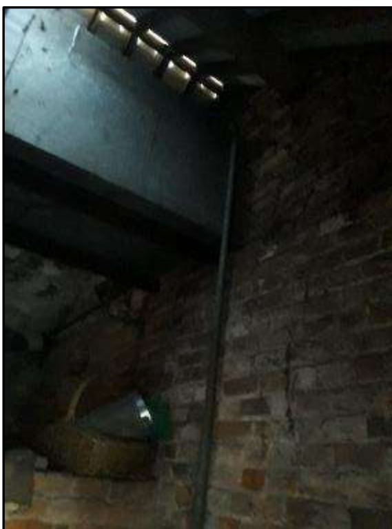
Plate MF84 – Remains of water tank to the single storey west of the south range
