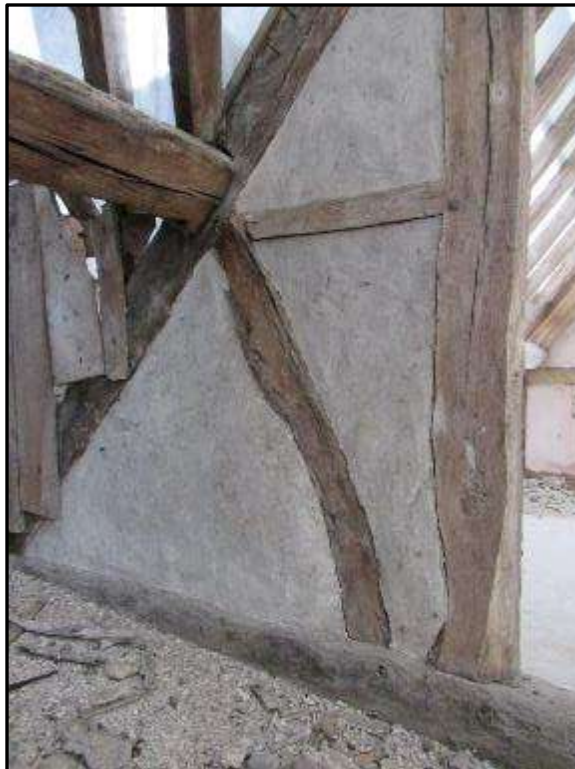
Plate MF148 – Wattle and daub infill panels and strut to the central roof truss
