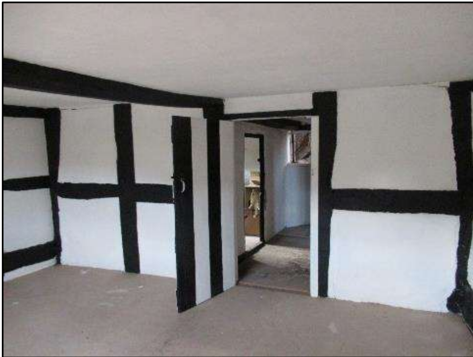
Plate MF141 – West internal dividing wall to the first floor of south range between large room (eastside) and landing area
