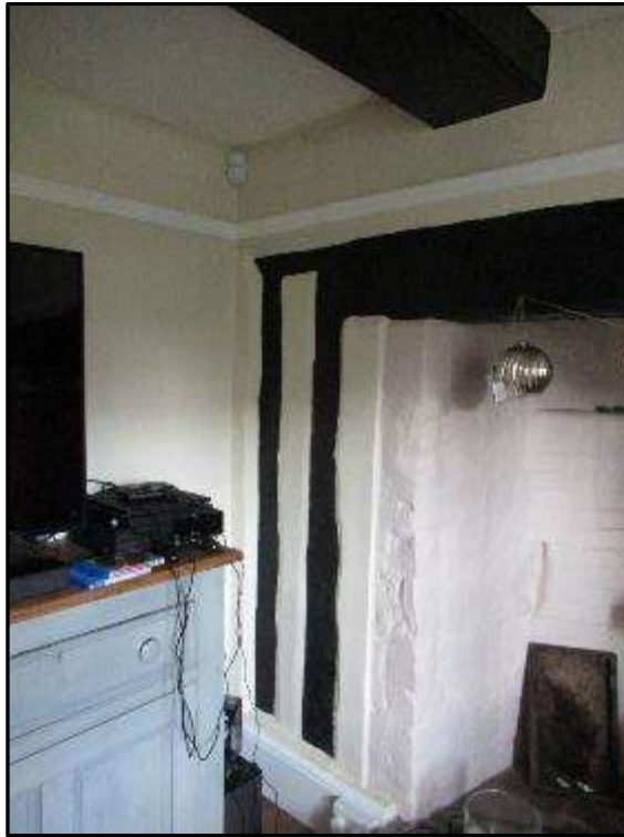
Plate MF69 – Stud posts to west of inglenook, possibly indicative of former partition wall
