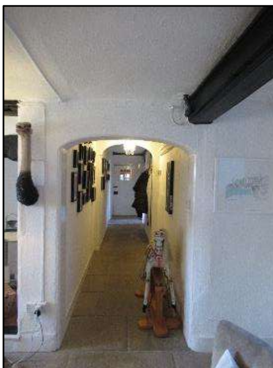
Plate MF64 – Main g/f passageway with arched entrance looking south from the entrance hall, note remains of girding beam to the top right of the image
