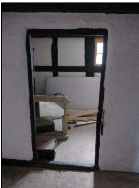
Plate MF136 – Opening within the south partition wall to small first floor room within the south range
