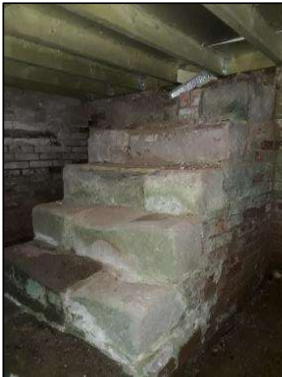
Plate MF104 – Stone steps to the original stair access to the cellar area below the south range located in the north west corner of the cellar
