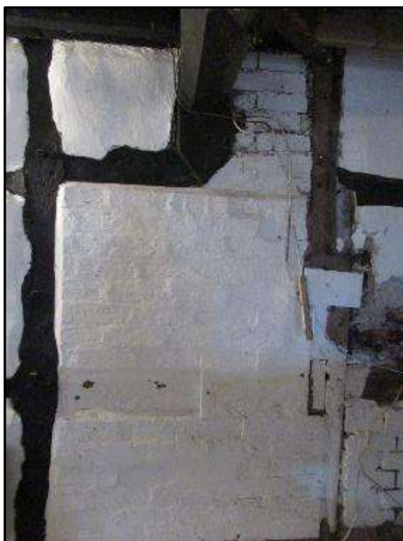
Plate MF95 – Infilled door opening in the west elevation of the south range
