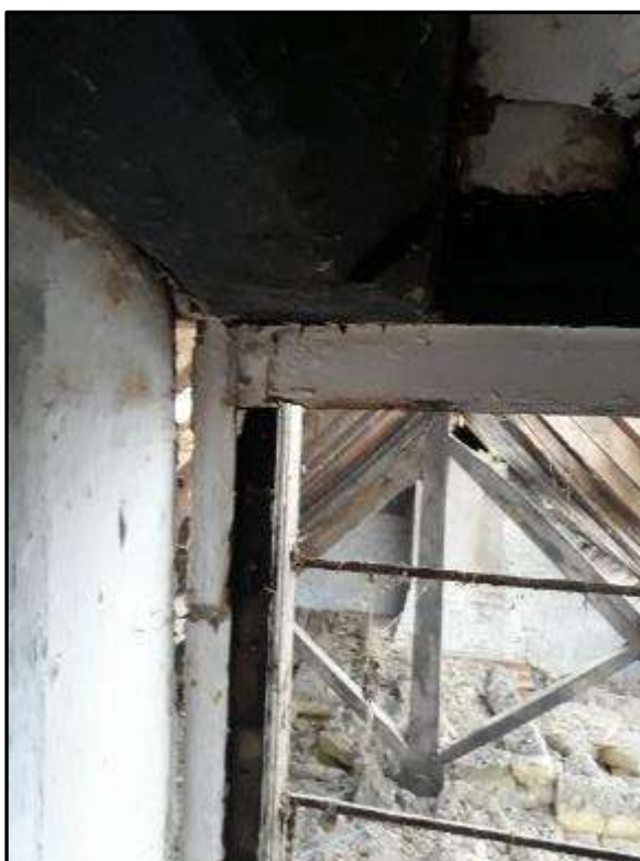
Plate MF135 – Metal casement window inserted to the west elevation of the range looking towards the roof space of the single storey west wing; note the king post and brick stack serving the large brick fireplace to the extant kitchen area
