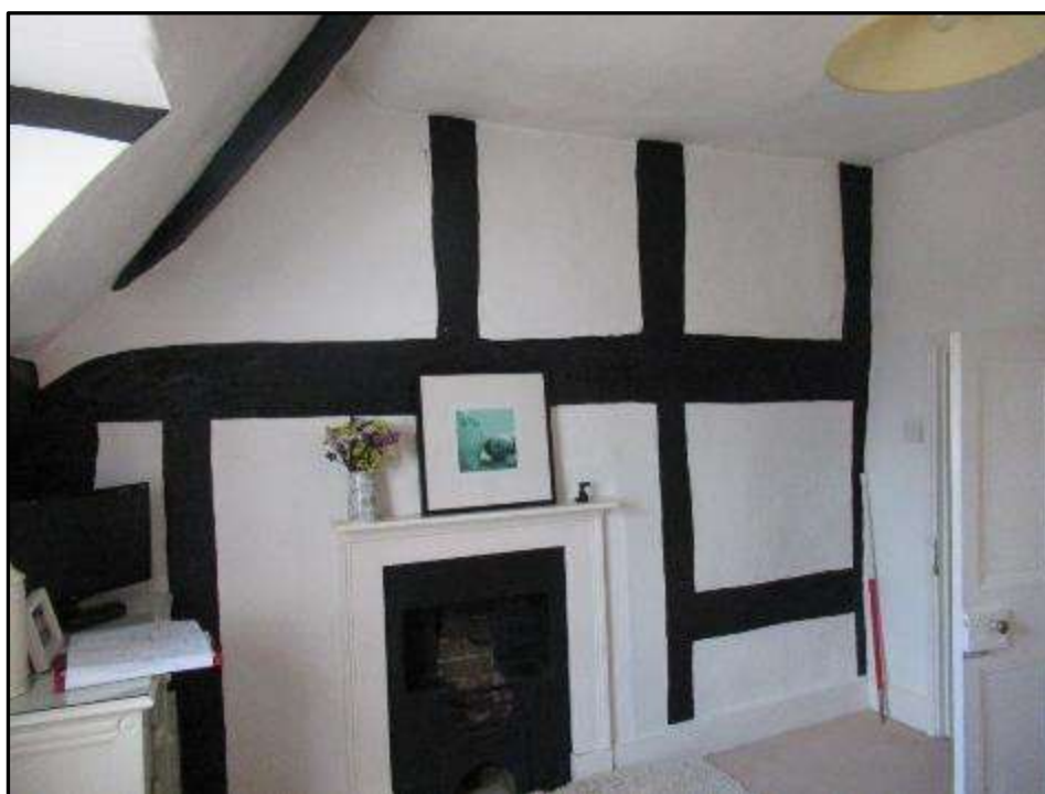
Plate MF123 – Timber frame construction to the south wall of the bedroom within the north bay of the central range (aligned above the main entrance hall)
