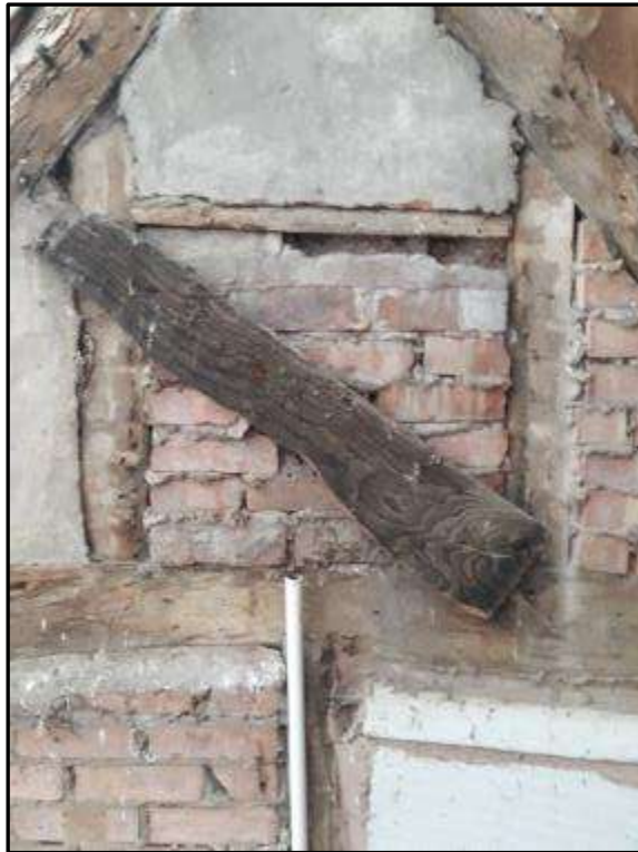
Plate MF155 – Evidence of previous repairs and alterations to the gable apex of the west elevation of the south range
