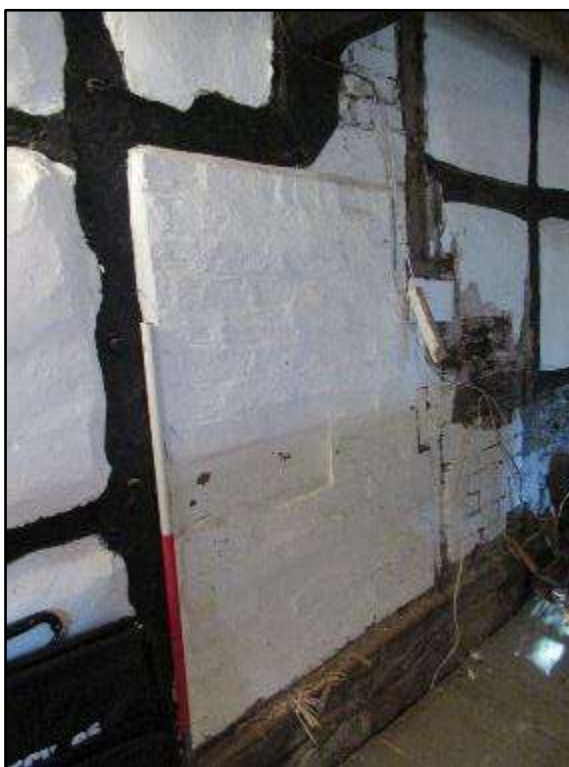
Plate MF94 – Infilled former doorway in the west wall of the south range indicative of former connection between the g/f room of the south range and the single storey west wing (extant kitchen area)
