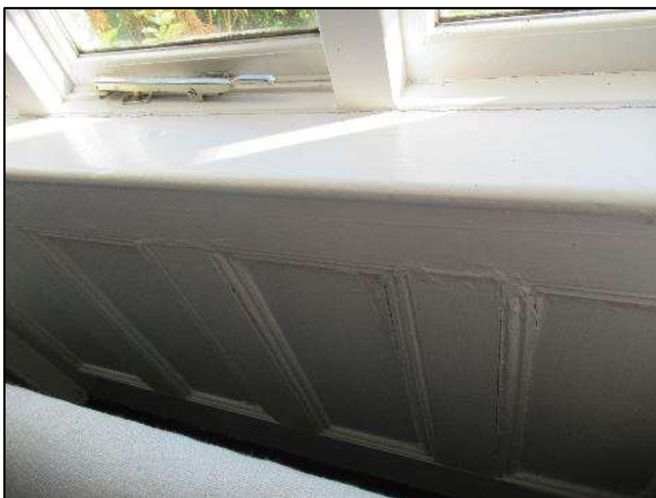
Plate MF51 – Fielded panels to base of the east window of the main sitting room
