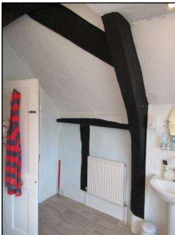
Plate MF118 – Remains of timber framing to the west wall of the first-floor bathroom
