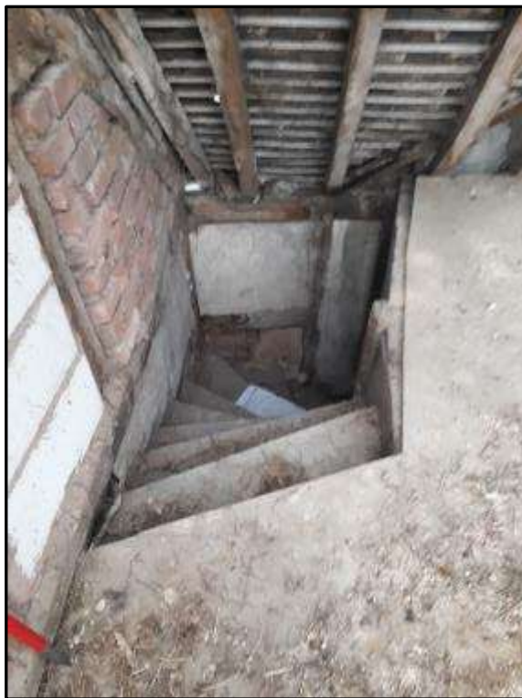
Plate MF144 – Dogleg stair within the north west corner of the south range
