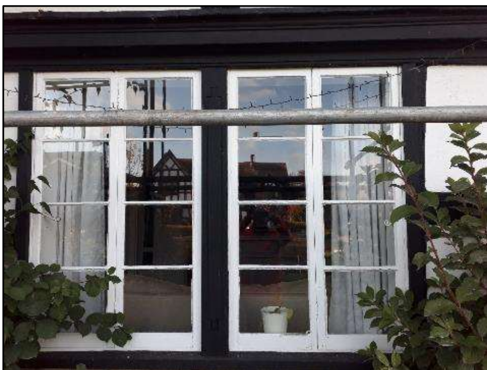
Plate MF3 – ‘Worcester’ style window to ground floor east elevation of central range
