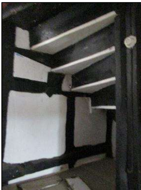
Plate MF134 – Underside of the second-floor staircase with framing to the west wall of the south range
