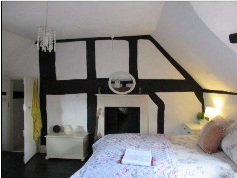
Plate Q – Timber frame to north cross wall of south bay of central range
