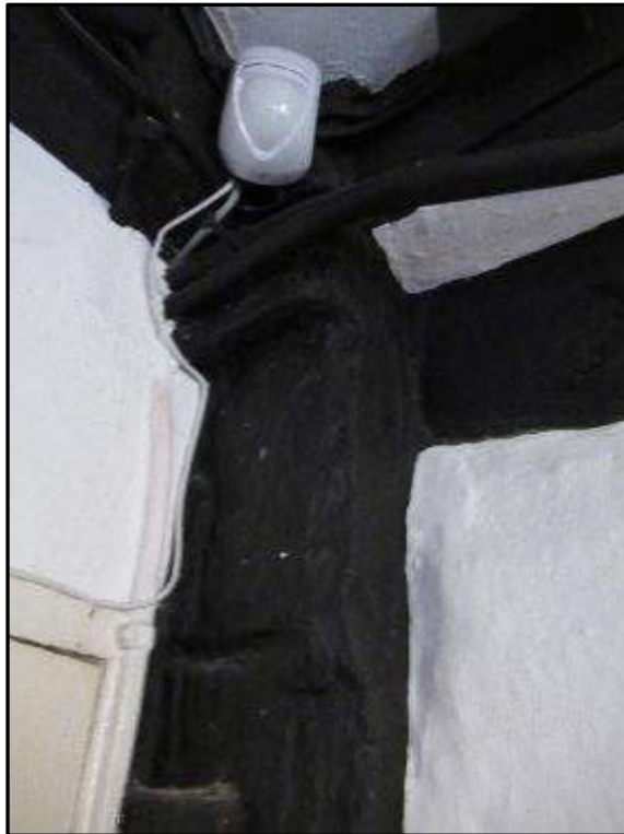
Plate MF57 – Junction of post and rail of remains of timber frame to south west corner of g/f bathroom
