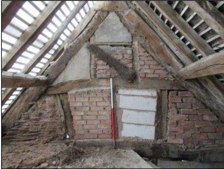
Plate T – Timber frame with original wattle and daub panels to the west end elevation of the south range
