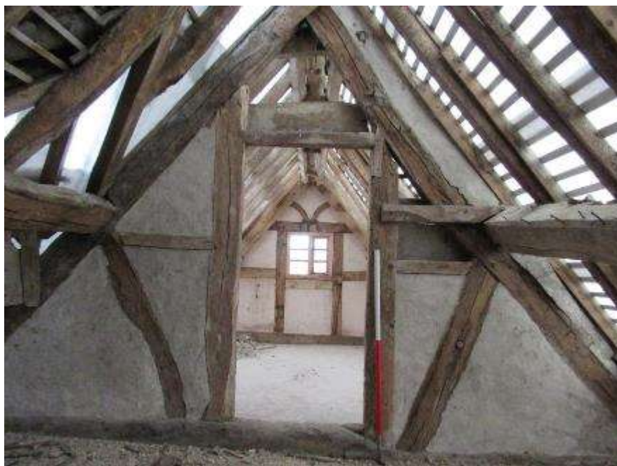
Plate U – Internal cross wall to the second wall of the south range
