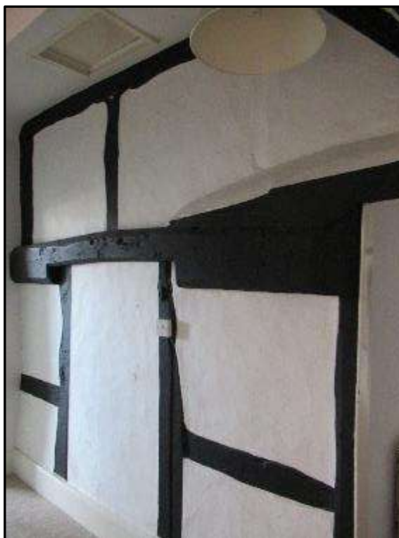
Plate MF116 – Timber box frame wall to the north wall of the central range (viewed from passageway within the north range)
