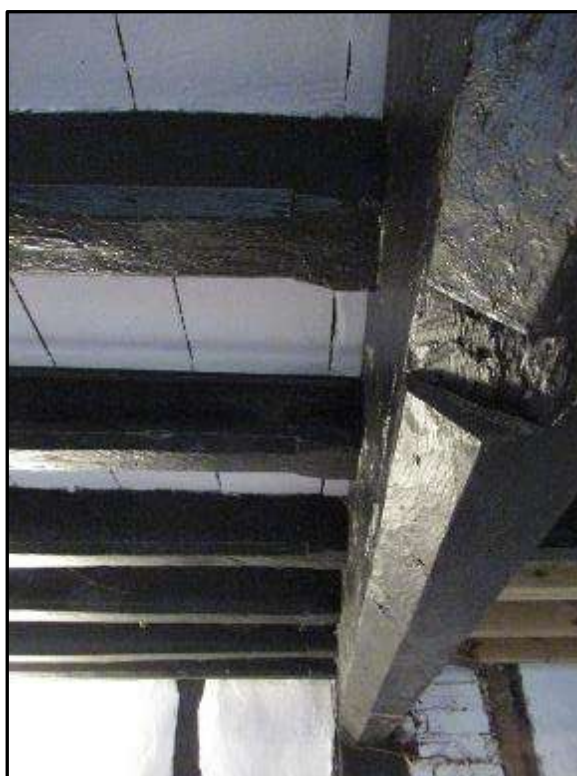
Plate MF96 – Chamfered bridging beam to g/f of the south range with chamfered joists; notch in beam may indicate line of former partition
