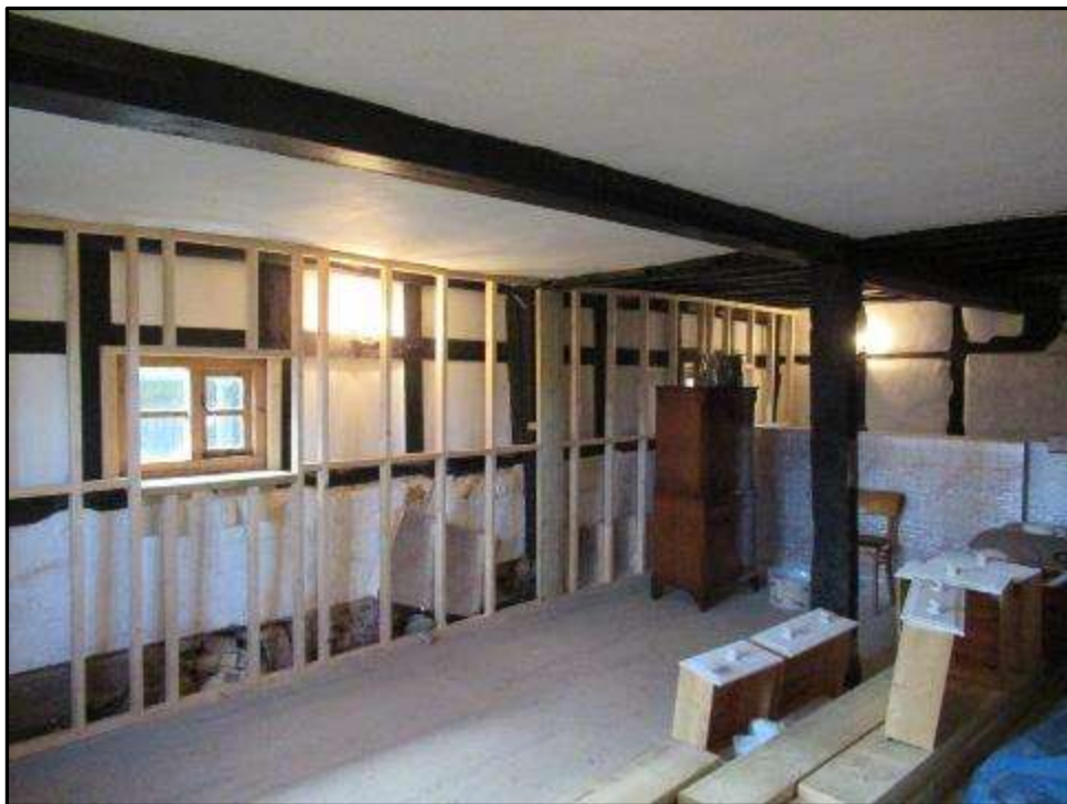
Plate MF92 – Renewed timber frame construction to the south wall of the g/f room of the south range
