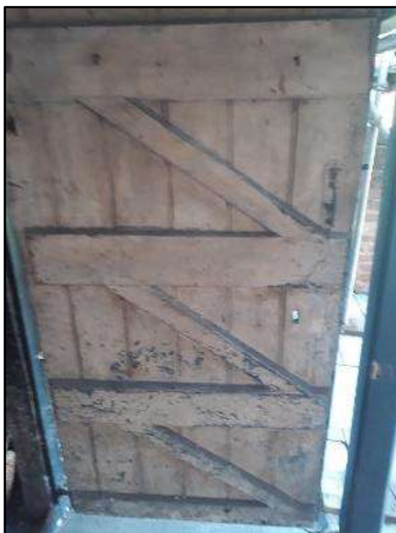
Plate MF22 – Interior view of external boarded door to north elevation of the single storey range showing timber ledge and braces
