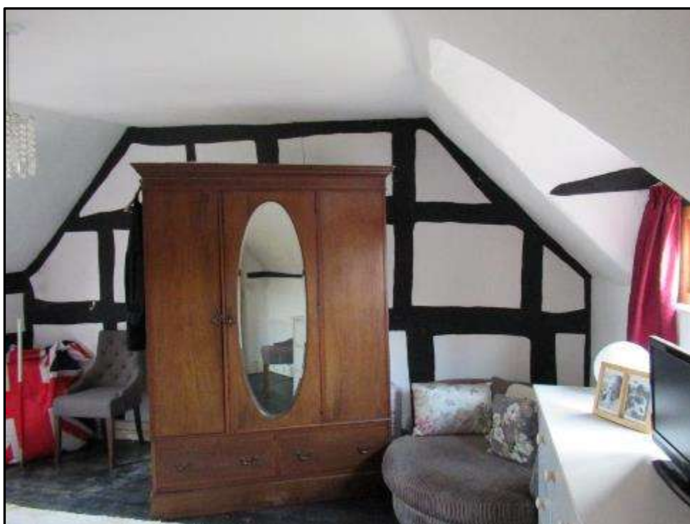
Plate MF129 – Timber frame construction to the south wall of the central range
