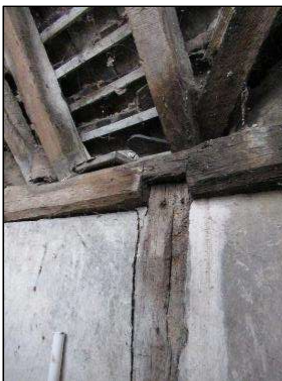
Plate MF154 – Joinery detail to the roof construction of the south range
