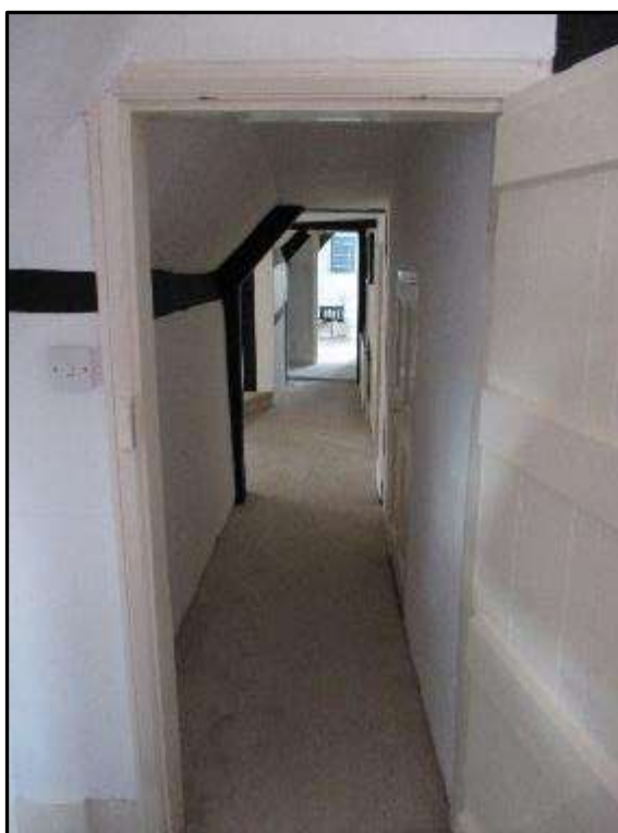
Plate MF126 – Main first floor passageway looking north towards the north rang; principle rafters of the roof trusses visible
