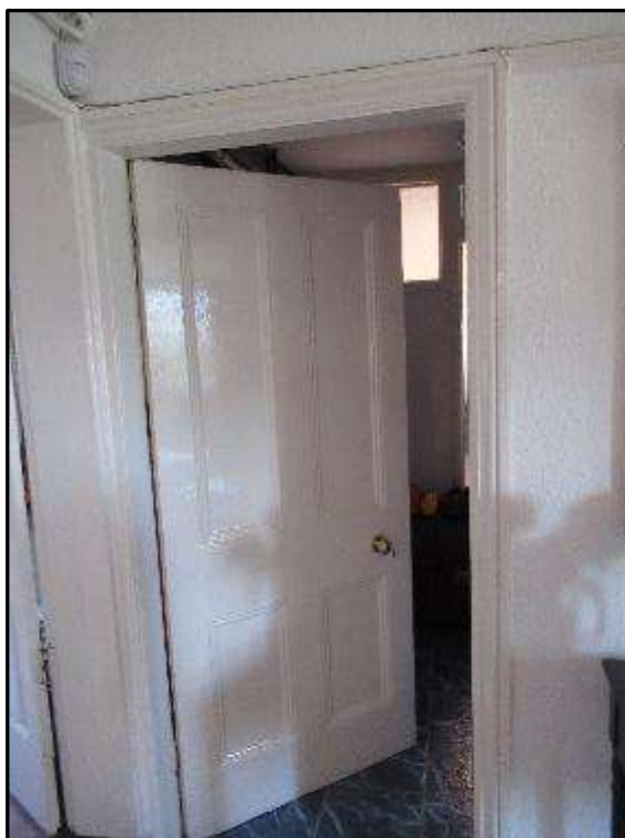
Plate MF54 – Four panel door and architrave to g/f bathroom (viewed from entrance hall)
