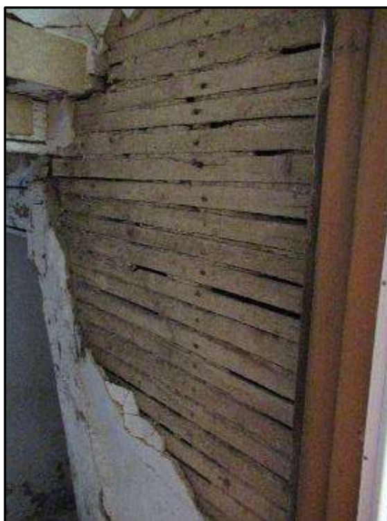
Plate MF62 – Exposed laths to interior of cellar stair
