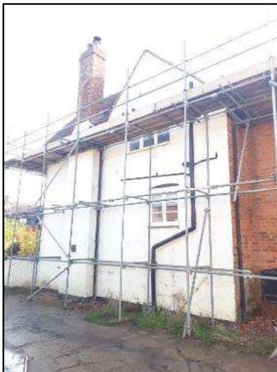
Plate MF38 – North elevation of the north range (east addition and connective gabled range)
