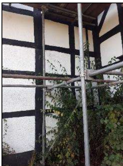
Plate MF4 – Timber frame to north return elevation of south range (viewed from the east)
