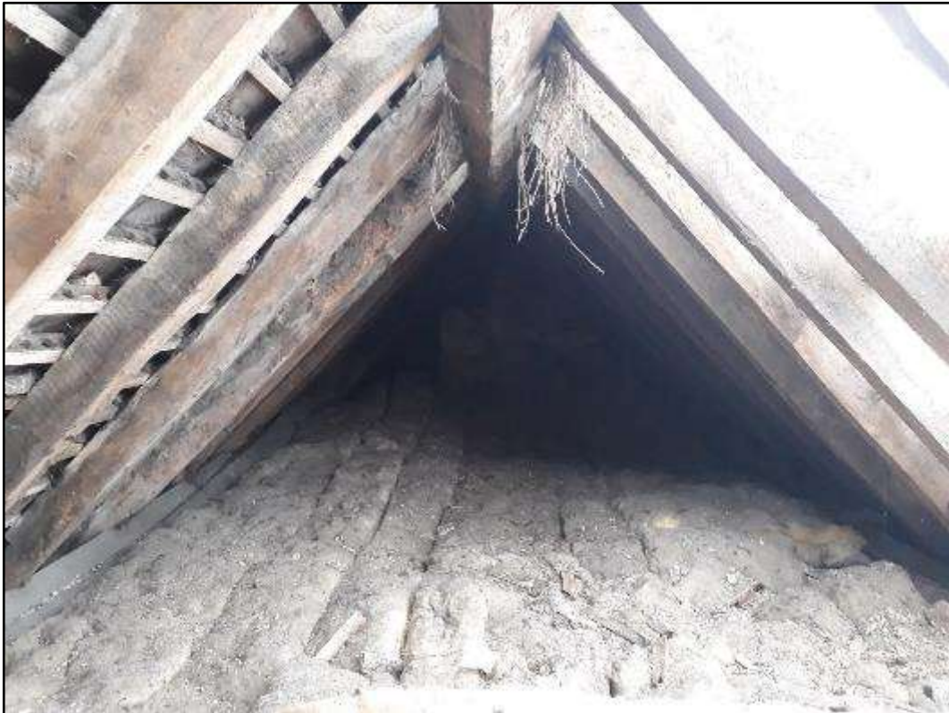
Plate V – Roof space above the south bay of the central range looking northwards towards the chimney stack
