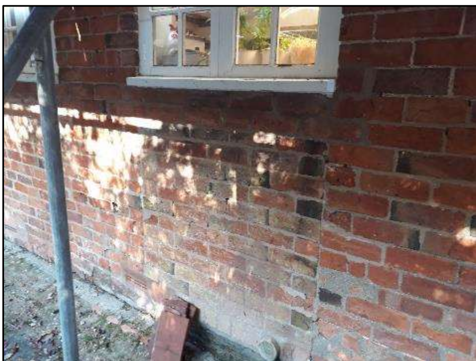
Plate MF17 – Infilled door opening to single storey wing adjoining the south range
