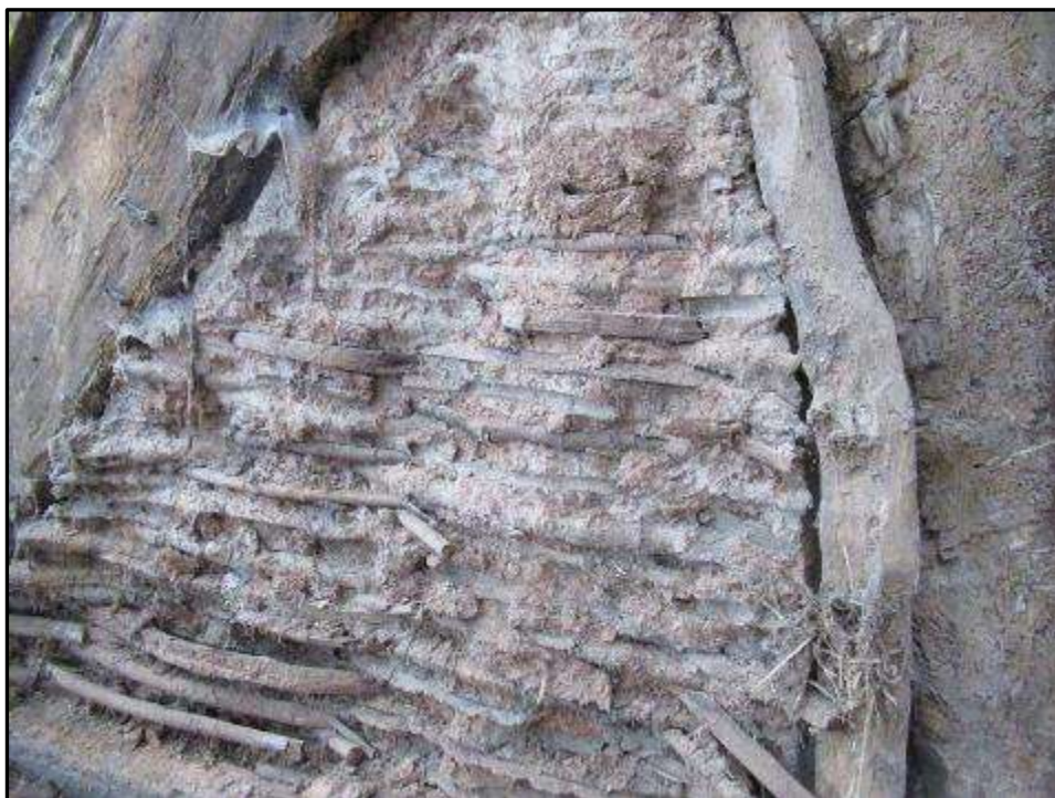
Plate MF153 – Exposed interior of the original wattle and daub panel showing the staves and mud/dung binding material
