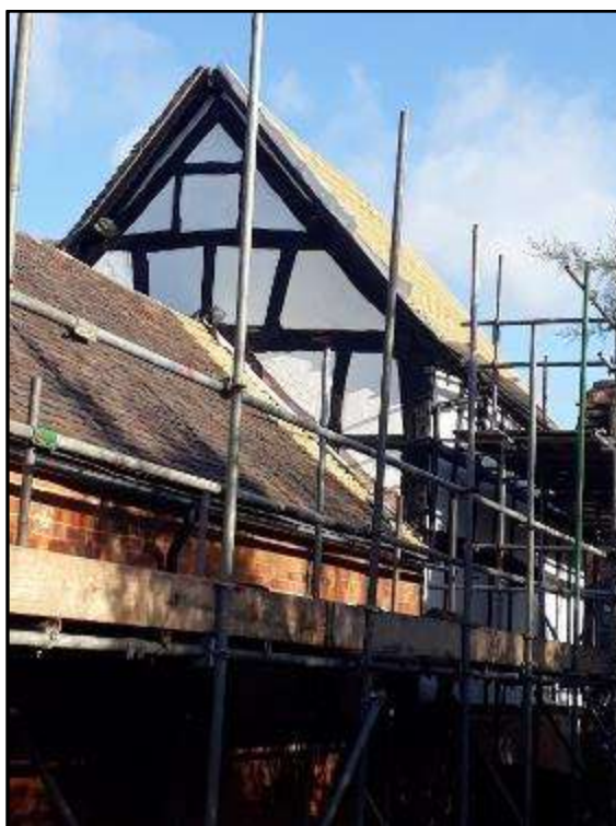
Plate MF18 – West gable end of south addition and south elevation of single storey wing
