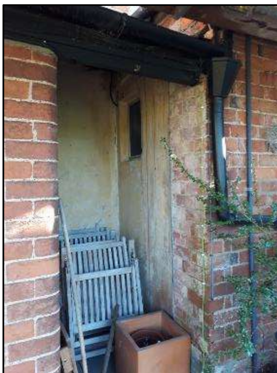
Plate MF29 – Infilled former rear door opening and canopy entrance porch to west elevation
