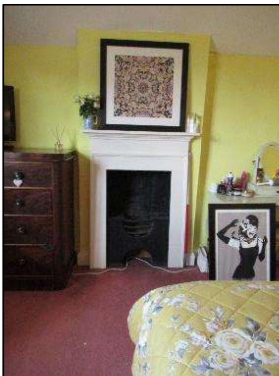
Plate MF112 – Early 19 th Century fireplace to bedroom in the west addition of the north range
