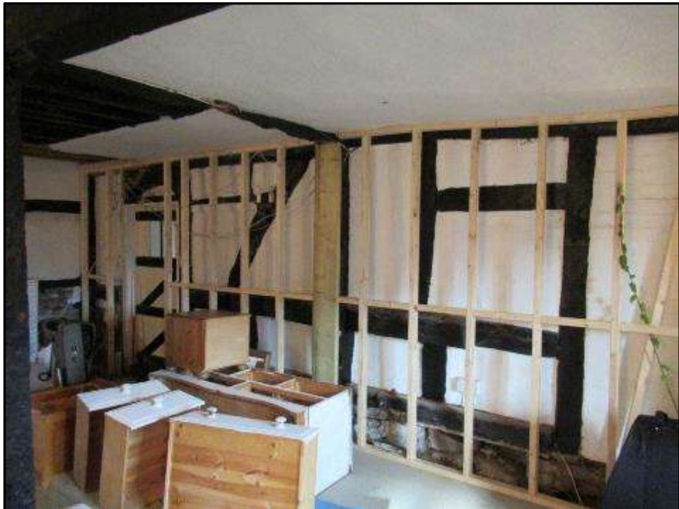
Plate MF89 – Timber frame to the dividing north wall of the south range and central range
