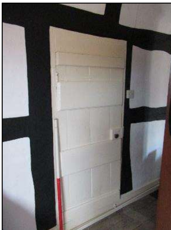
Plate MF130 – Plank and braced door to the south wall of the central range giving access to the first floor of the south range
