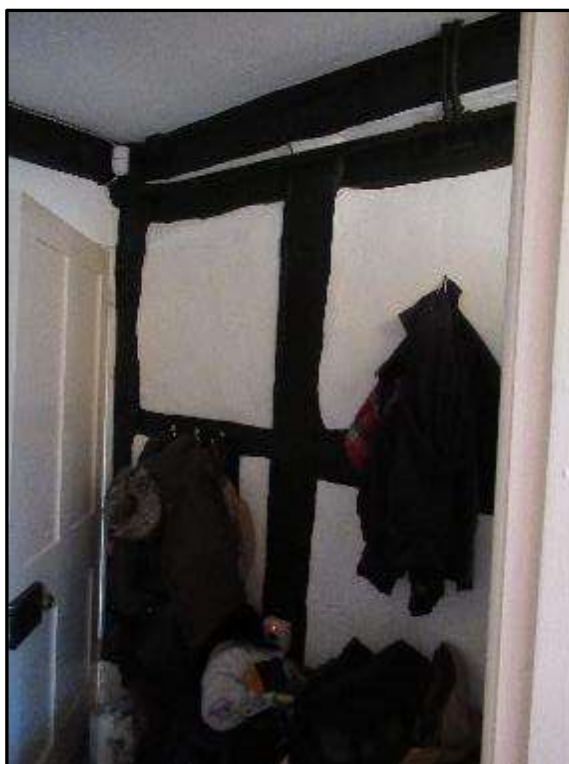
Plate MF55 – Timber frame to part west wall of g/f bathroom
