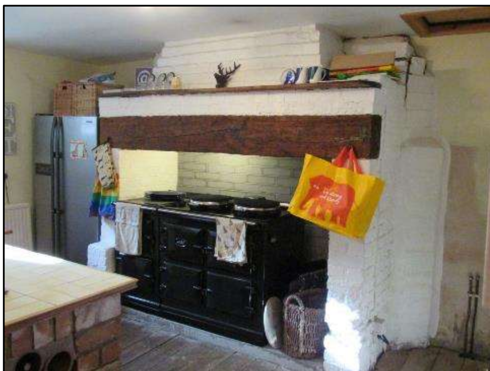
Plate MF80 – Brick fireplace and timber bressumer beam inserted to the single storey west wing of the south range
