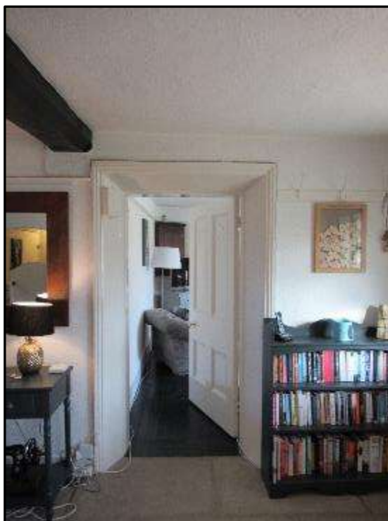
Plate MF47 – splayed timber architrave to main sitting room in the east addition of the north range (viewed from entrance hall)
