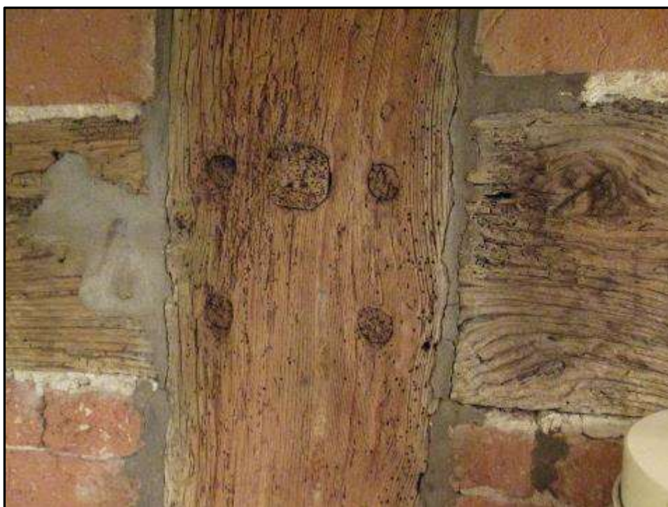
Plate MF82 – Exposed timber frame with pegs to the west wall of the three-storey south range (viewed from the kitchen area)
