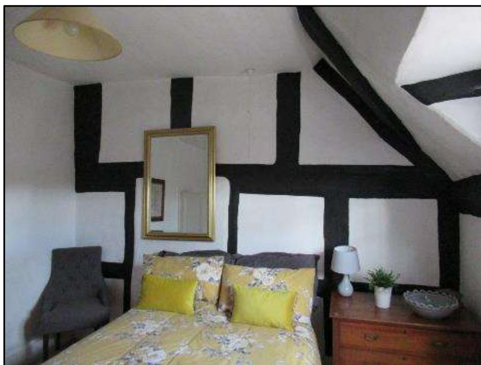
Plate MF121 – Timber frame to the bedroom within the north bay of the central range
