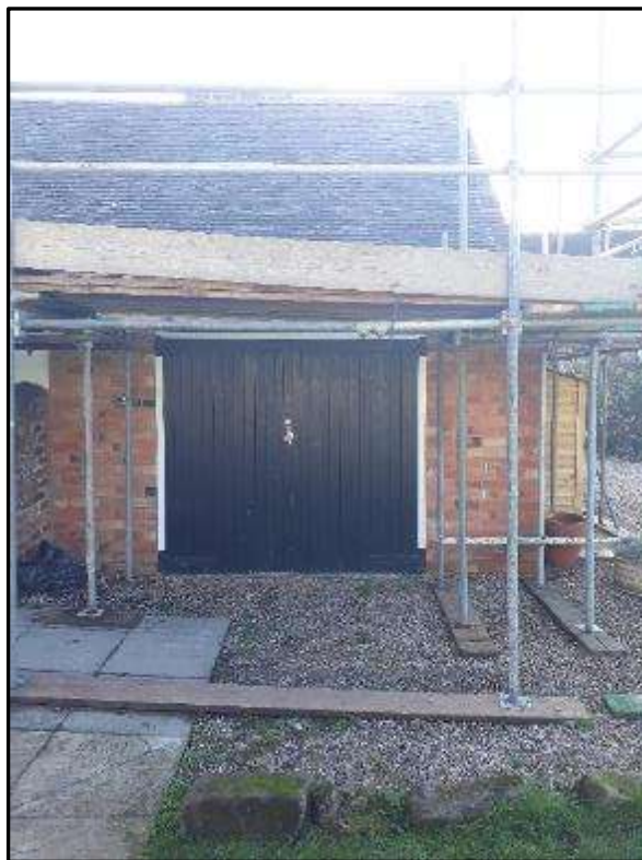
Plate MF20 – North elevation of single storey addition (overlooking rear garden) with modern side hung doors within later infill extension
