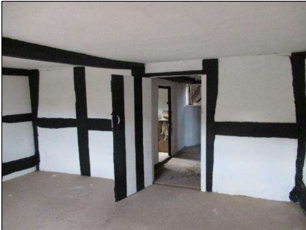
Plate S – Timber frame and boarded door to internal cross wall to first floor of south range
