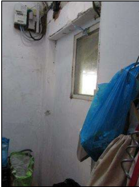
Plate MF77 – Infilled former rear entrance door to rear porch in west elevation
