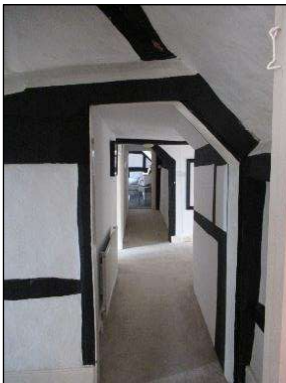
Plate MF115 – First floor passageway looking south along the west end elevation through the central range
