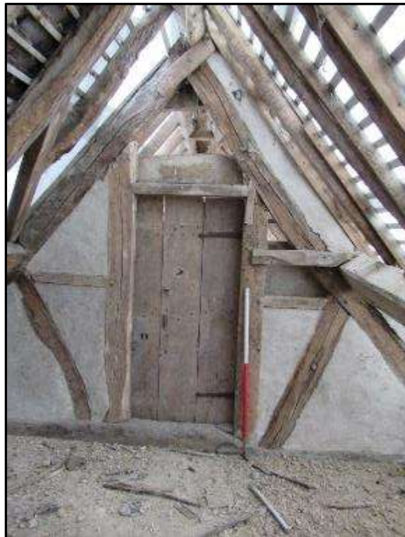
Plate MF150 – 17 th Century oak boarded door to the second floor of the south range looking east
