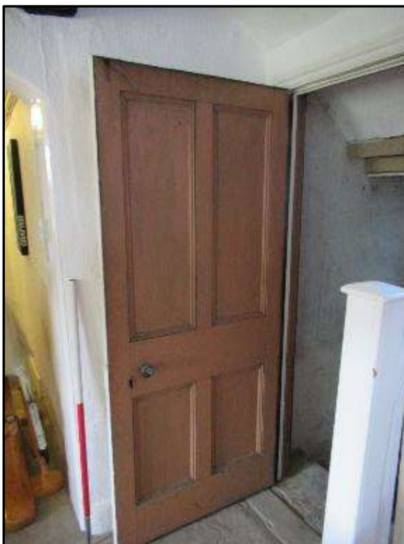
Plate MF61 – Four panel door (interior) to cellar area below the west addition of the north range
