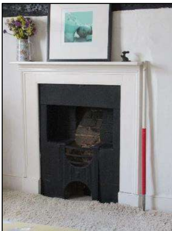
Plate MF 124 – Early 19 th Century fireplace to the bedroom in the north bay of the central range
