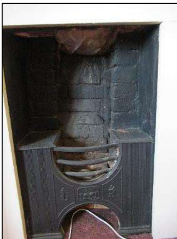
Plate MF113 – Hob grate and brick fireback to early 19 th Century fireplace in bedroom within the west addition of the north range
