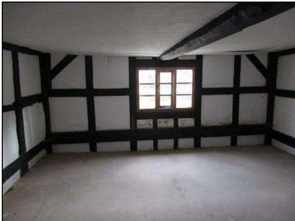
Plate MF142 – East elevation of the south range with renewed timber frame construction and window opening and chamfered bridging beam below modern ceiling
