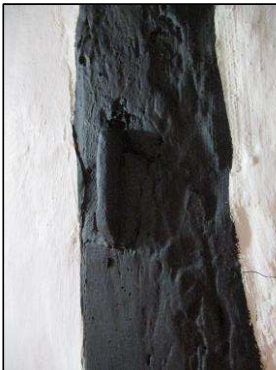
Plate MF117 – Remains of metal pintle to timber post within the north wall of the central range indicative of a former door opening
