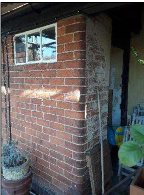
Plate MF28 – Rounded brick edge to single storey rear porch addition (west elevation)
