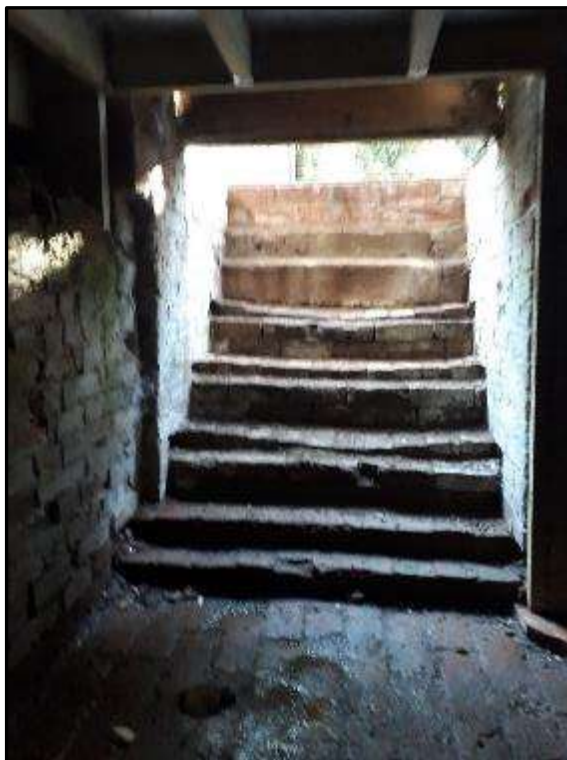
Plate MF106 – Steep, narrow brick steps to the cellar from the external entrance hatch in the south
