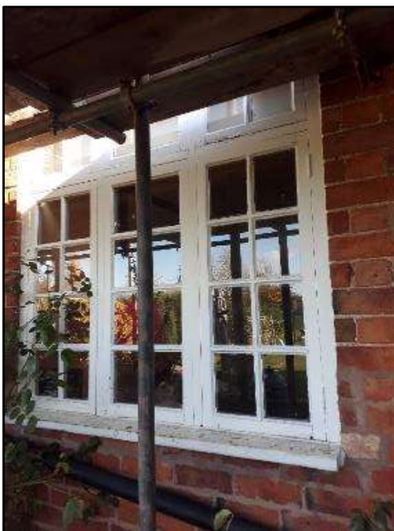
Plate MF27– Timber casement window to single store addition to west elevation
