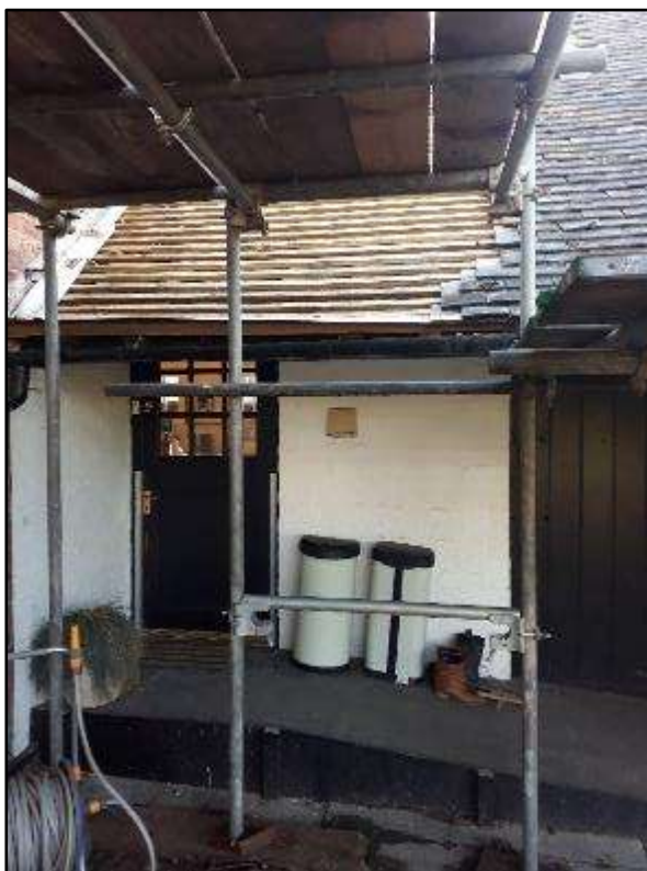
Plate MF23 – Rear entrance door to the north elevation of west wing to south range
