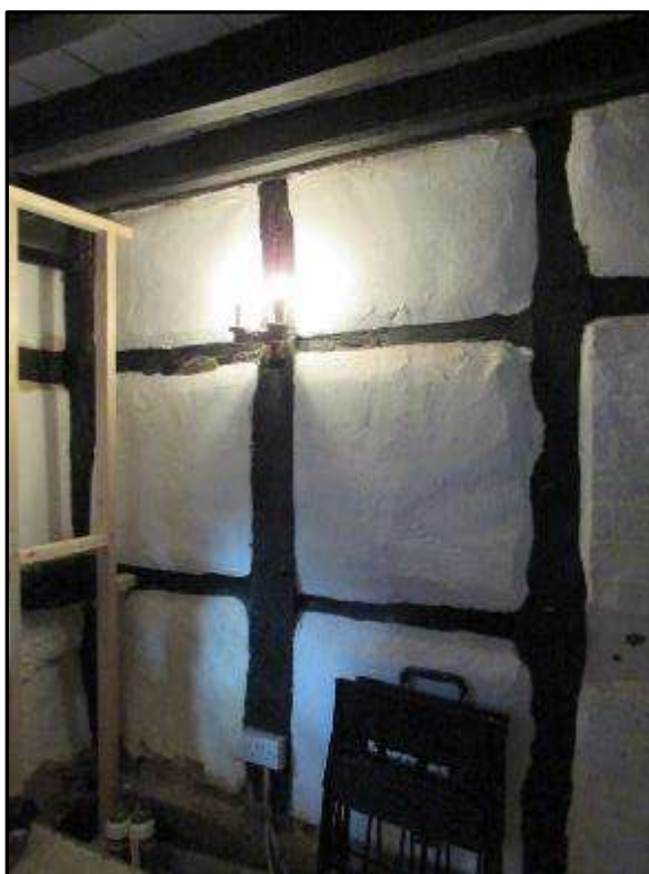
Plate MF93 – Original timber box frame construction to the west wall of the g/f room of the south range
