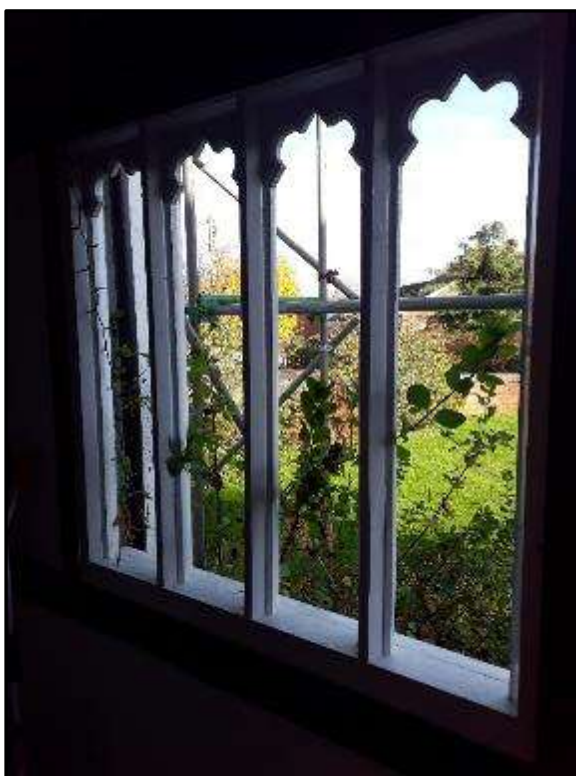
Plate MF8 – East elevation, gothic shaped openings to east elevation of entrance porch
