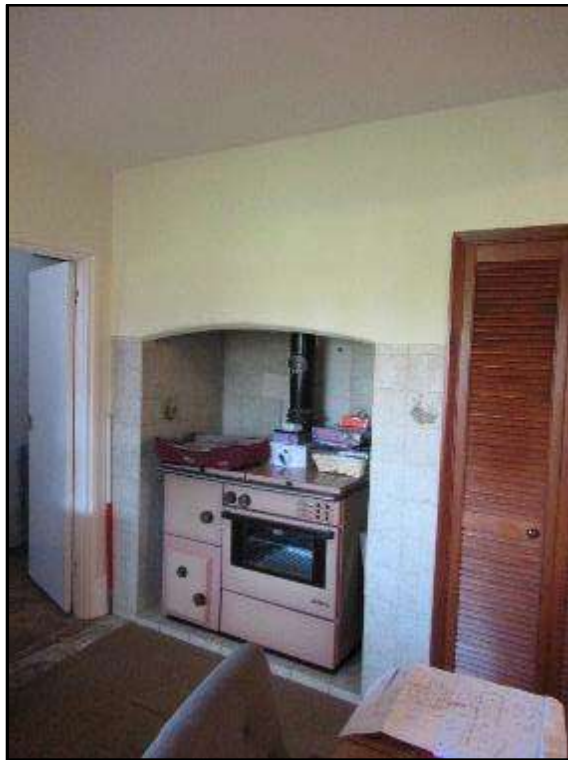
Plate MF75 – Segmental arched fireplace and chimney breast to be removed (built against the west wall of the central range)
