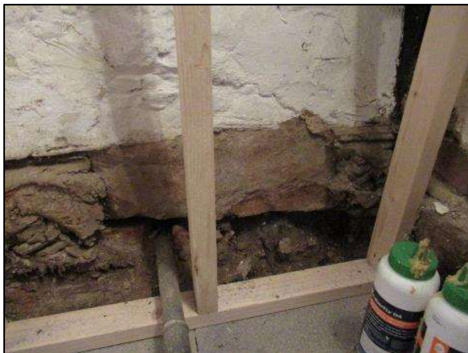
Plate MF102 – Stone plinth to the south wall of the g/f room of the south range
