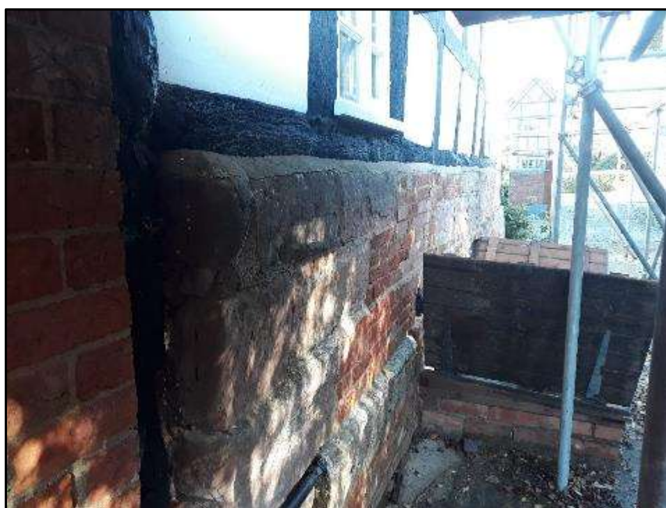
Plate MF16– South elevation, junction of stone plinth and adjoining single storey wing to the west
