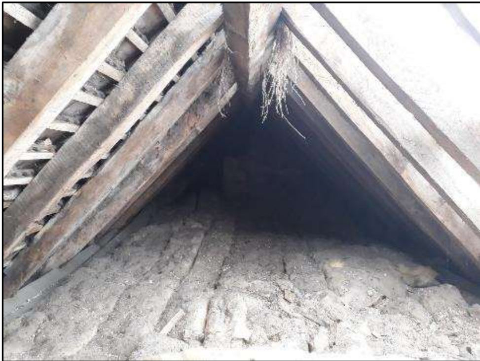
Plate MF157 – Roof space above the central range with renewed timber joists (viewed from the south range)
