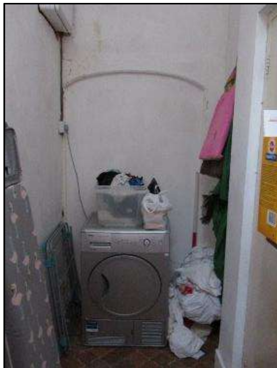
Plate MF76 – Infilled arched opening to west wall of the central range (viewed from within the utility room)
