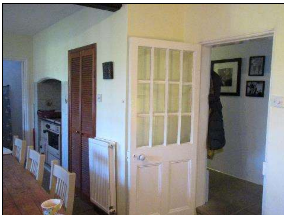
Plate MF73 – Modern cupboard and chimney breast to be removed within the dining room
