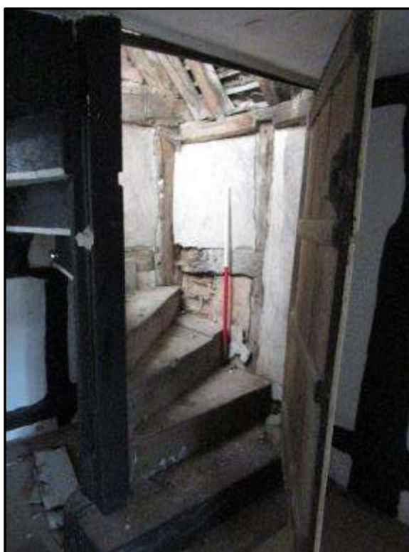
Plate MF132 – Staircase to the second floor of the south range within the north west corner of the first floor of the south range
