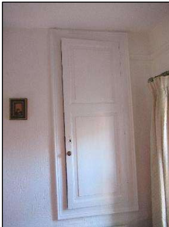
Plate MF58 – Built-in cupboard to sitting room in west addition (north range)
