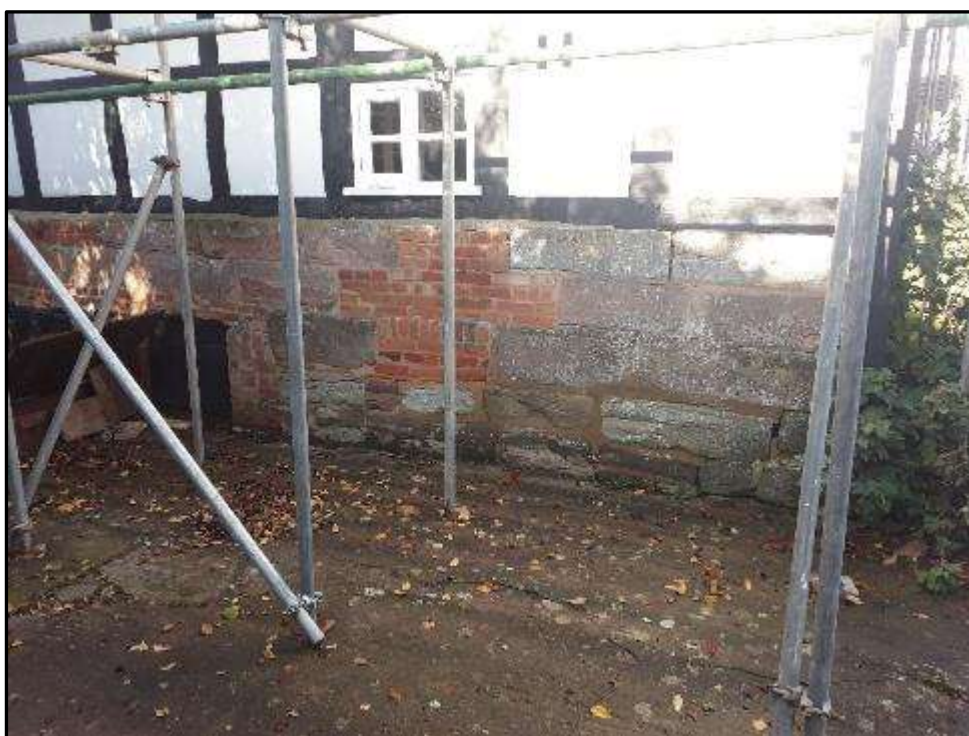
Plate MF15 – South elevation of the south range showing alteration in brick to the stone plinth
