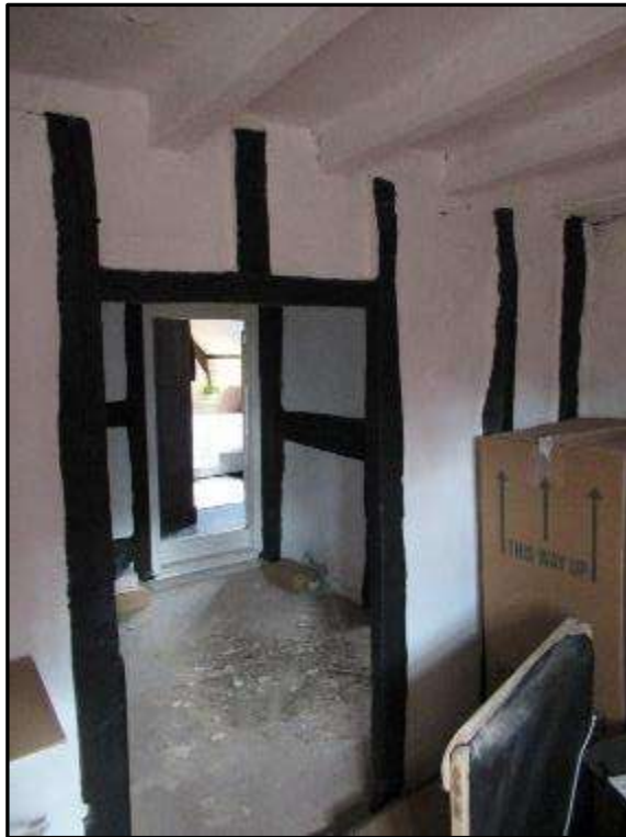
Plate MF139 – Close stud framing to the internal subdividing wall between the small first floor room and the first-floor landing area
