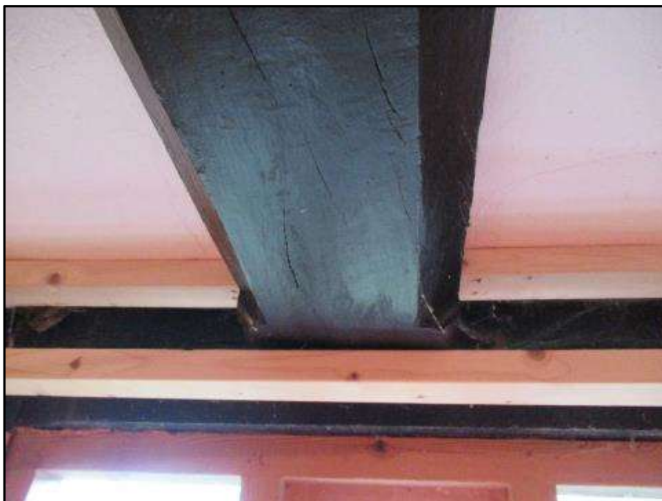
Plate MF97 – Chamfered bridging beam with stops aligned east to west through the g/f room of the south range (east end)
