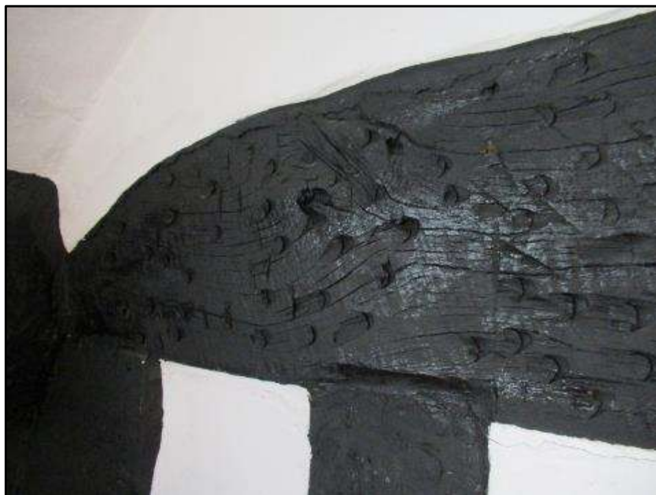
Plate MF122 – Linear and circular scratch marks to the timber frame in the south wall of the northern bay of the central range
