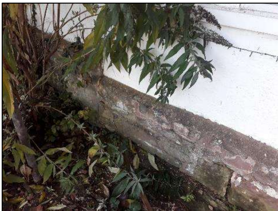
Plate MF6 – East elevation, stone plinth to ground floor of central range
