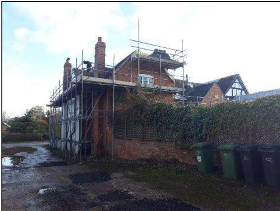
Plate MF36 – Part west and part north elevation from track adjacent to the north elevation
