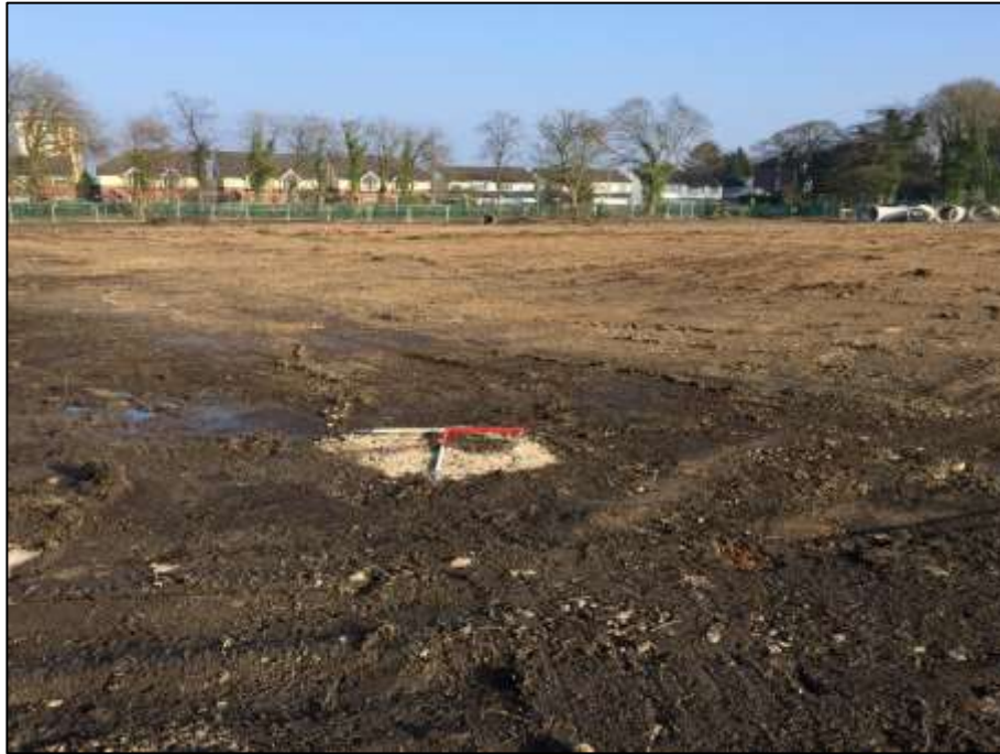
Plate 1; General shot of site after topsoil strip looking east-south-east. Scales = 2 x 1m
