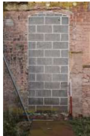
DP 26: Detail of an infilled doorway, where there originally was a window, taken from the south-east.
