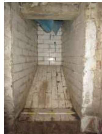
DP 52: Detail of one of the four chutes or light wells, taken from the north-west.
