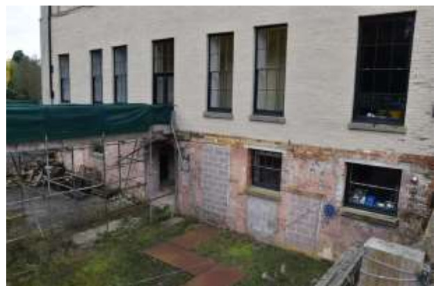
DP 6: General view of the former basement from ground floor level, taken from the east.
