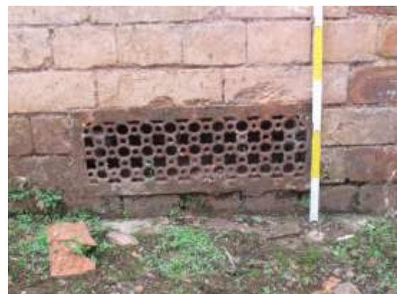
DP 42: An example of the grated vents along the Victorian wall, taken from the north-west.
