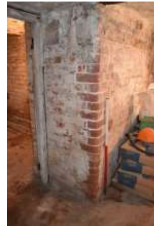
DP 46: The bullnose brickwork of the short linkage to the principal vaulted unit, taken from the east.
