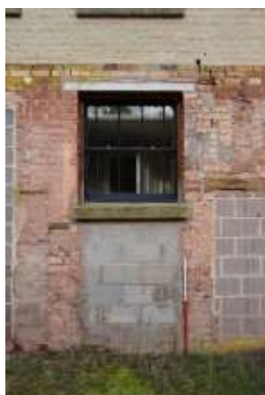
DP 27: Detail of the infilled doorway, likely of the servants' linkage, taken from the south-east.
