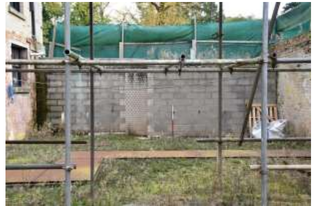
DP 10: The modern retaining wall to the east, taken from the south-west.
