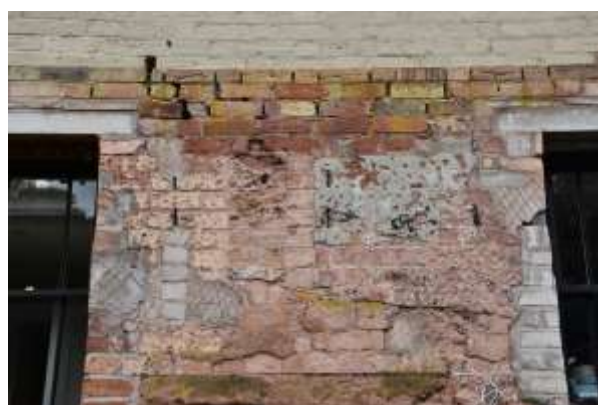
DP 30: View of the remnants of the demolished wall, showing the extent of redevelopment, taken from the south-east.
