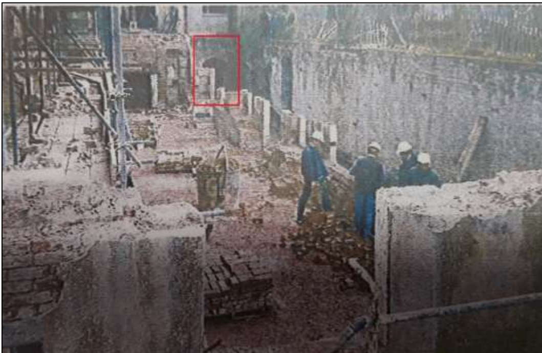
Fig.H: A 1997 photograph of the demolition programme (PWPT 1993), with the probable access to the passageway highlighted by the author.
