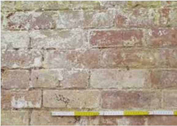
DP 43: An example of the brickwork of the Victorian wall, taken from the north-west.
