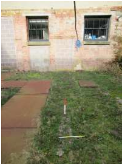
DP 31: Possible remnants of the demolished wall at basement floor level, taken from the south-east.
