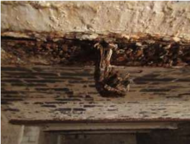
DP 55: Detail of one of the steel I-Beams with an additional hook, taken from the north-east.
