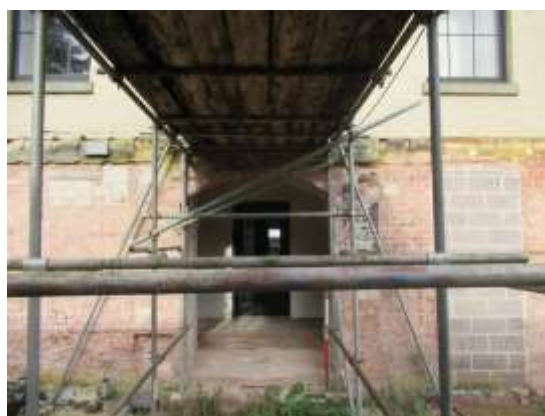
DP 18: General view of the central arched entrance, taken from the south-east.
