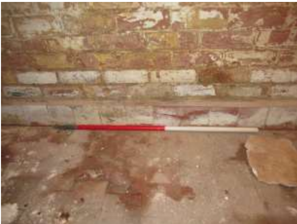
DP 57: Detail of the tile skirting along the northern wall of the vaulted cellar, taken from the south-east.
