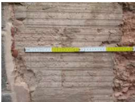
DP 35: Sample of the cement adhesive of the tiles, taken from the south-east.
