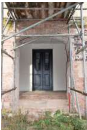
DP 19: Detail view of the central segmentally arched and recessed entrance, taken from the south-east.
