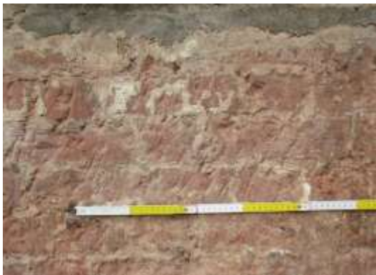
DP 33: Sample of the original brickwork identified below the easternmost window, taken from the south-east.
