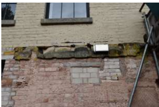
DP 17: Remnants of stonework upon which joists were supported, taken from the south-east.
