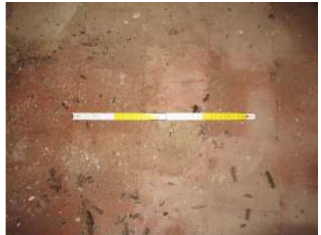
DP 58: Detail of the tiled flooring in the vaulted cellar, taken from the south-east.
