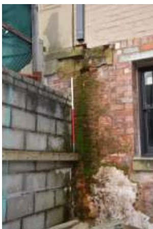
DP 15: Potential remnants of the original retaining wall and remains of former render, taken from the south-east.
