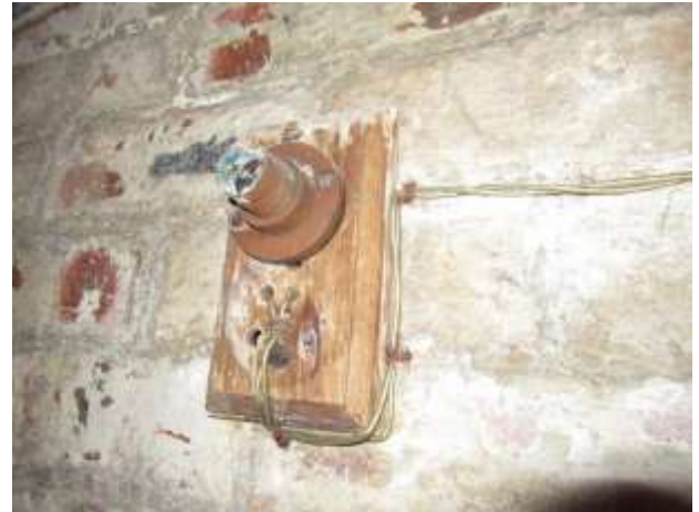
DP 56: Detail of the redundant central light fixture, taken from the south-east.
