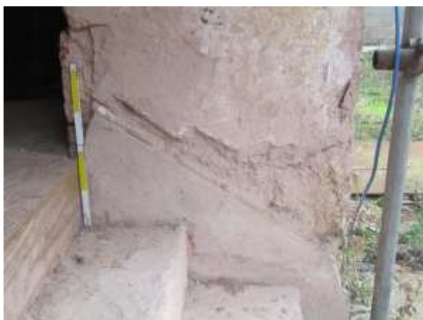
DP 21: Detail of the formed skirting that line the stone steps, taken from the south-west.
