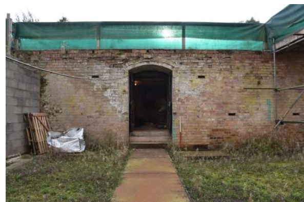
DP 36: The eastern section of the Victorian wall and entrance to Soane's vaulted cellar, taken from the north-west.
