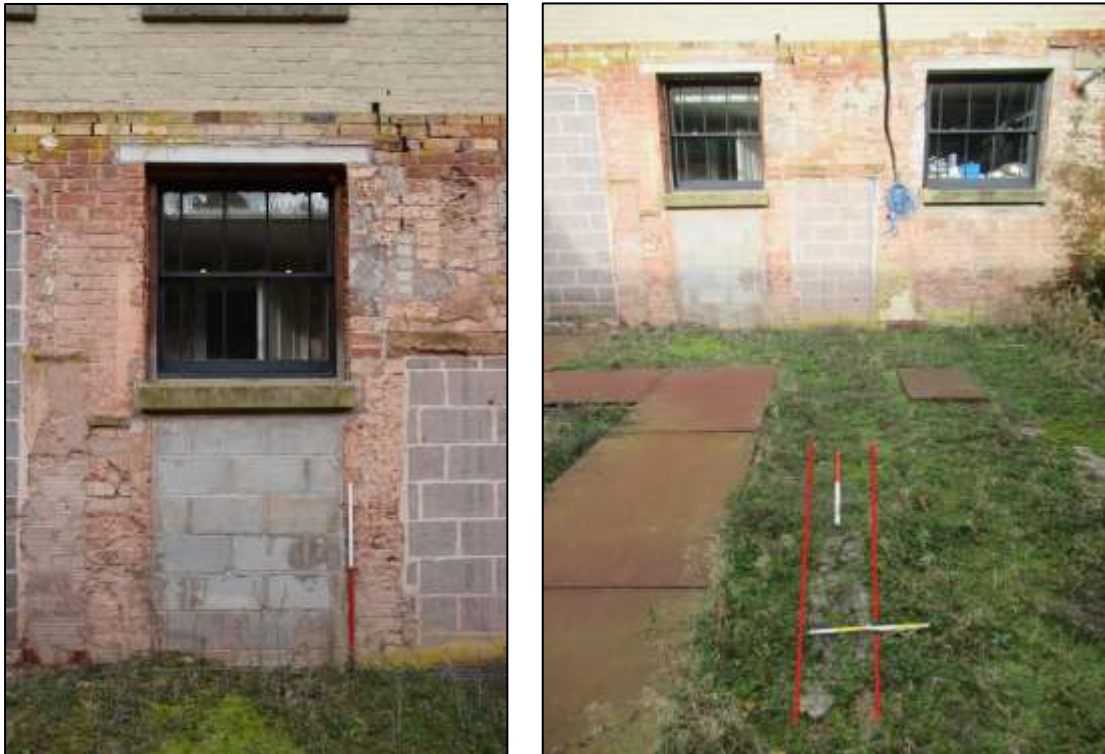
Plate 9: The infilled door of the demolished linkage at basement level – left (DP 27).
