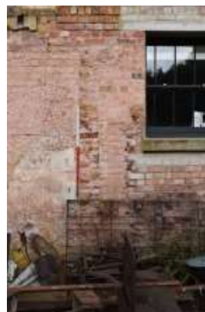
DP 16: The demolished wall of a storage room accessed via the original kitchen, taken from the south-east.
