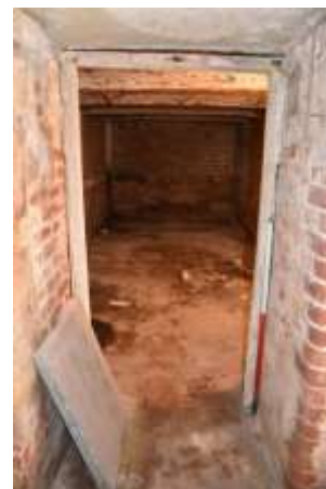
DP 48: The chamfered doorframe of the short linkage, taken from the north-east.
