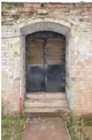
DP 39: The arched and recessed entrance to the vaulted cellar, taken from the north-west.
