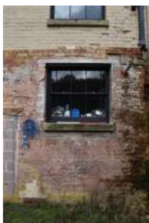
DP 29: Detail of the easternmost modern window, in the same location as Soane's original, taken from the south-east.
