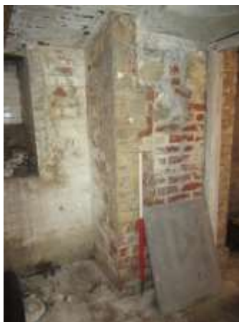
DP 47: The latterly added brickwork, potentially installed for structural strength, taken from the
