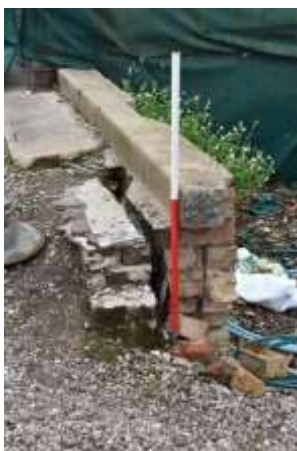
DP 41: The Victorian brick 'skin' at ground level, appended an original wall, taken from the west.
