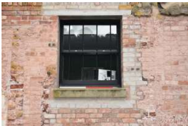
DP 13: Modern window in the position of an original doorway, with infilled area below, taken from the south-east.
