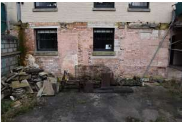
DP 11: The western section of the south-eastern elevation, taken from the south-east.
