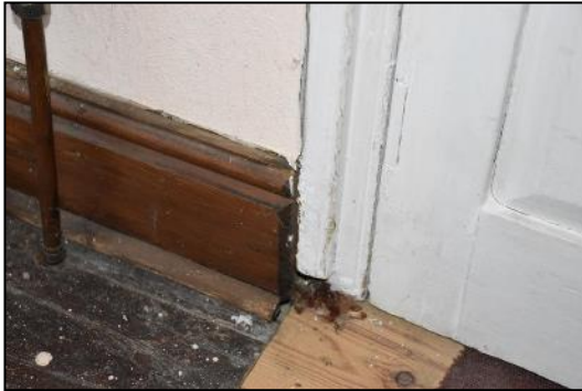
DP 151 Detail of the modern skirting in FF07 (Range 3), taken from the north-west
