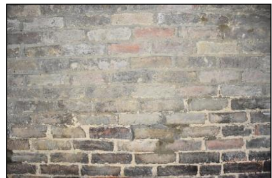
DP 54 Brickwork on the west side of the throughway (Range 2), taken from the east
