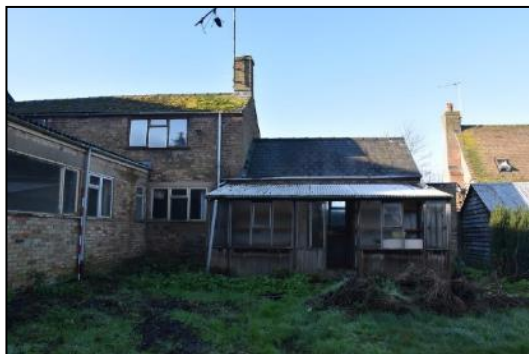
DP 41 East side of Ranges 3 and 4 with modern conservatory at low level, taken from the east
