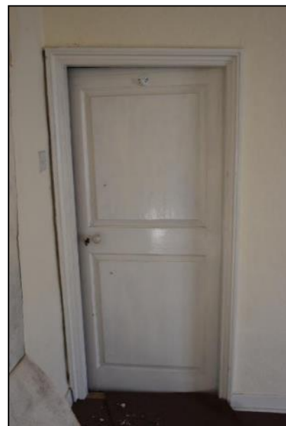
DP 138 Two-panel door in the north-east corner of FF01 (Range 1), taken from the west
