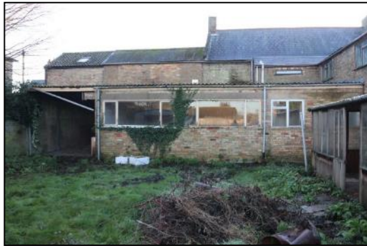
DP 43 North elevation of Ranges 1 and 2 (first floor) with Range 6 at low level, taken from the north
