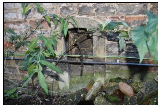
DP 36 West elevation (Range 3) showing position of former boot scraper adjoining the blocked doorway, taken from the west
