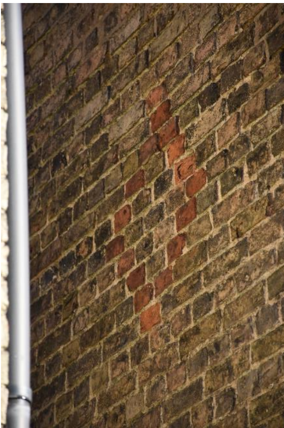
Plate 5 West elevation (Range 1) showing decorative diamond picked out in red brick, taken from the south-west (DP 29)
