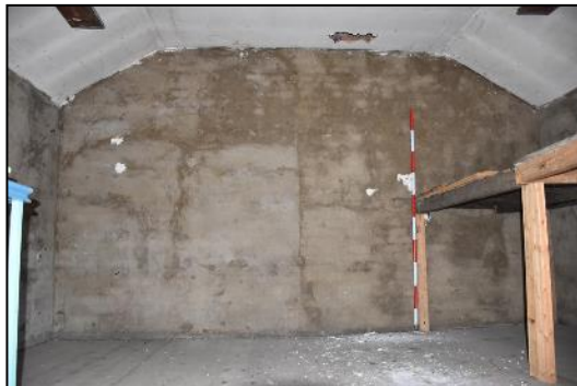
DP 105 East end of FF06 (Range 2) with possible outline of former aperture, taken from the west
