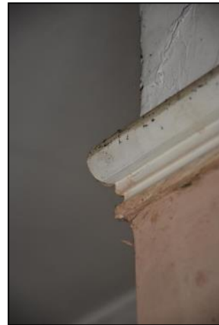
DP 116 Detail of the picture rail in FF04 (Range 1), taken from the south-west
