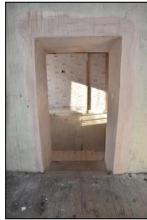
DP 110 Doorway punched through the chimney stack between FF04 and FF06 (Ranges 1 and 2), taken from the east
