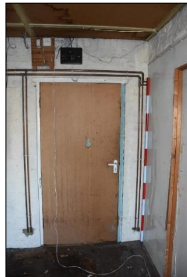
DP 96 South end of GF06 (Range 6) showing modern doorway inserted into the rear wall of Range 1, taken from the north
