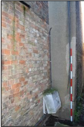
DP 31 Junction between Range 1 and 3 (north-east side) showing area of disturbed brickwork, taken from the north
