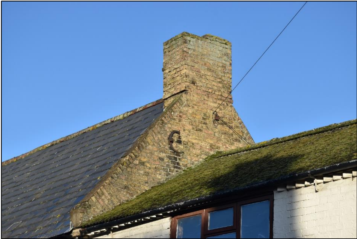
Plate 4 East gable-end of Range 1 showing tumbled-in brickwork and iron tie-plate, taken from the south-east (DP 8)
