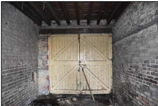
DP 51 Double doors on the south side of the throughway (Range 2), taken from the north
