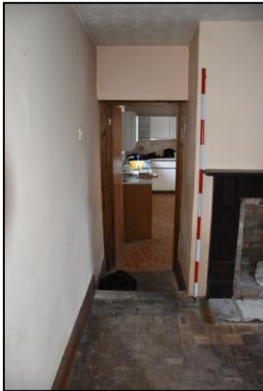
DP 85 North-west corner of GF04 (Range 3) inserted to give access to GF05 (Range 4), taken from the south
