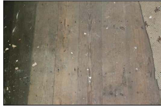
DP 128 Detail of the floorboards in FF02 (Range 1), taken from the east
