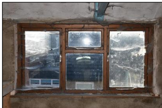
DP 107 Window on the south wall of FF06 (Range 2), taken from the north
