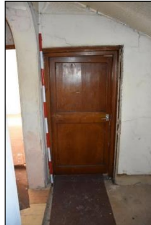
DP 146 Two-panel door on the west side of FF05 (Range 5), taken from the east
