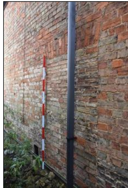
Plate 8 West elevation (Range 3) showing blocked doorway in the centre, taken from the south-west (DP 9)
