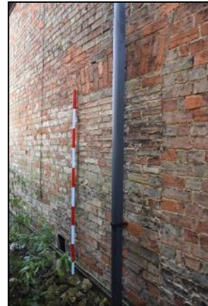
DP 34 West elevation (Range 3) showing blocked doorway in the centre, taken from the south-west
