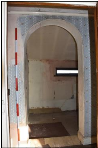
DP 123 Corridor FF03 (Range 1) showing aperture to Range 5, taken from the south
