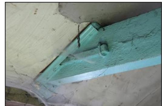
DP 108 Detail of a tie-beam in FF06 (Range 2) showing iron strapping, taken from the west
