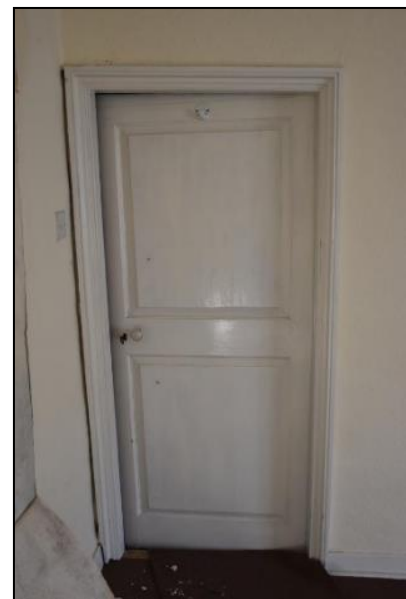
Plate 12 Two-panel door in the north-east corner of FF01 (Range 1), taken from the west (DP 138)
