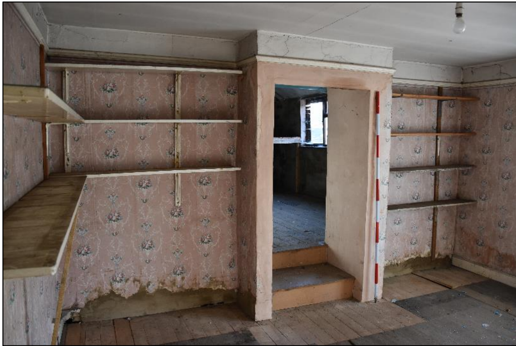
Plate 14 East side of FF04 (Range 1) showing doorway punched through the chimney stack into the adjoining range, taken from the west (DP 111)
