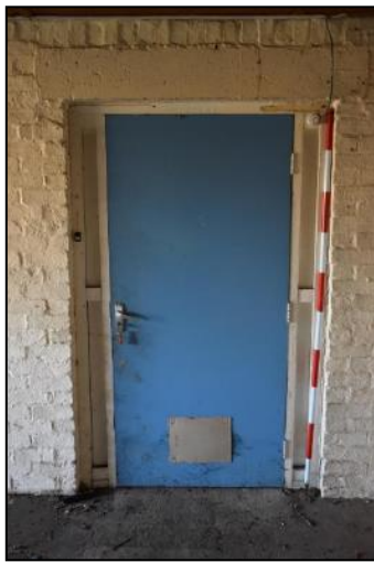
DP 99 East wall of GF07 (Range 6) showing doorway to the throughway, taken from the west
