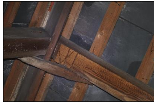
DP 134 Rafter in the roof structure (Range 1) showing possible Baltic timber mark, taken from the south-east
