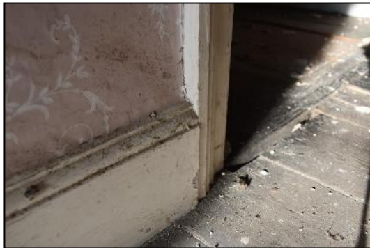
DP 117 Detail of the skirting board in FF04 (Range 1), taken from the south-east
