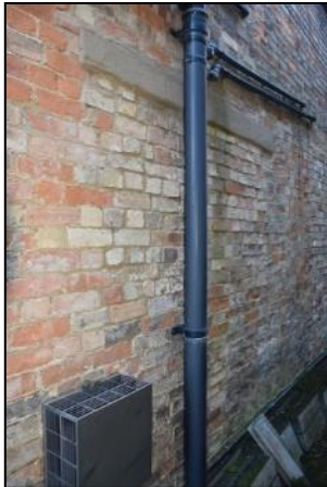
DP 33 West elevation (Range 3) showing blocked doorway in the centre, taken from the north-west
