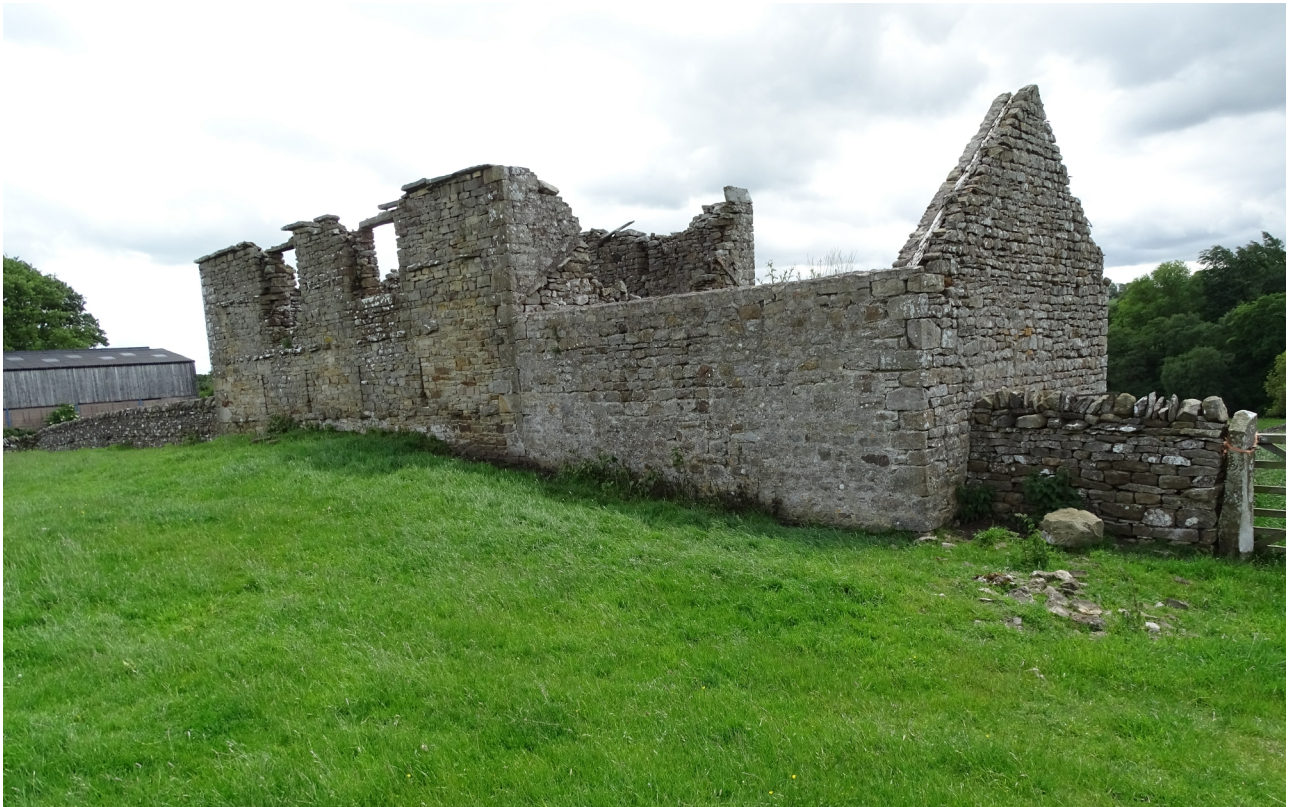
Plate 7. The northern elevation from the northwest with the extension in the foreground (frame GVB19001)
