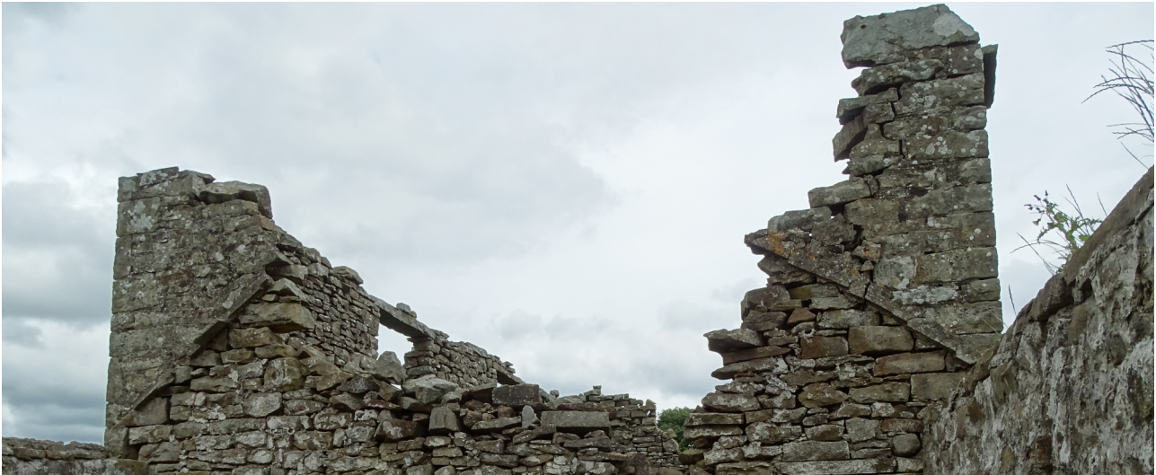
Plate 8. The remains of the original barn western gable end, obscured by the roofline from the extension (frame GVB19017)
