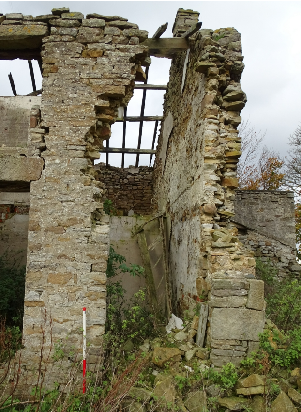
Plate 7. The collapse and door jamb (detail) (frame WCW006).
