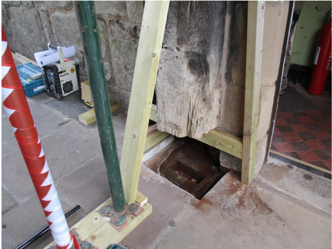
Plate 3: The Jamb after removal of its base and excavation of loose material.
