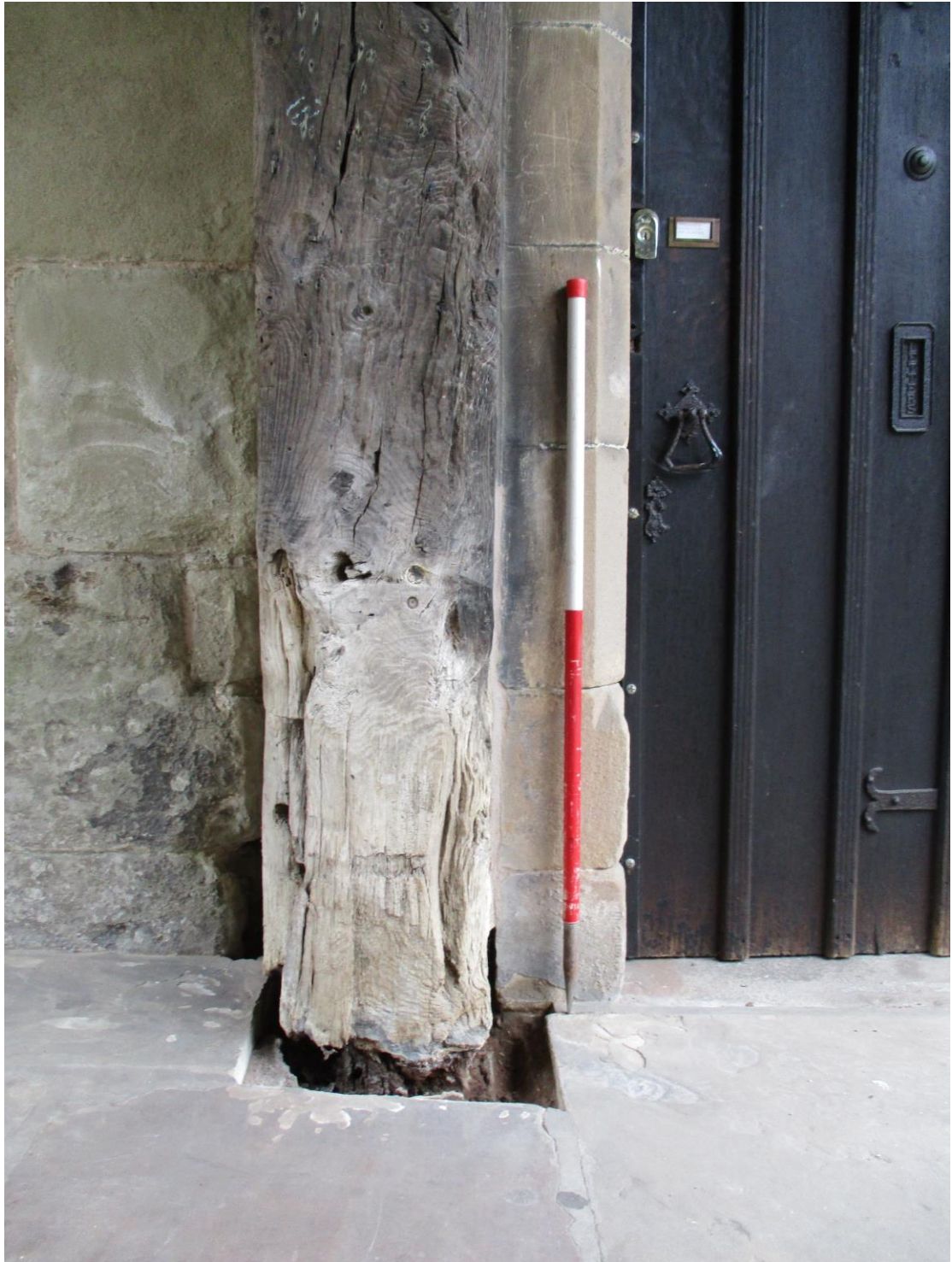
Plate 1: Timber jamb looking east, showing the extent of the damage and rot.
