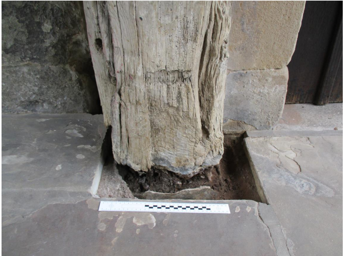
Plate 2: Detail showing splintering and abrasion to the jamb.
