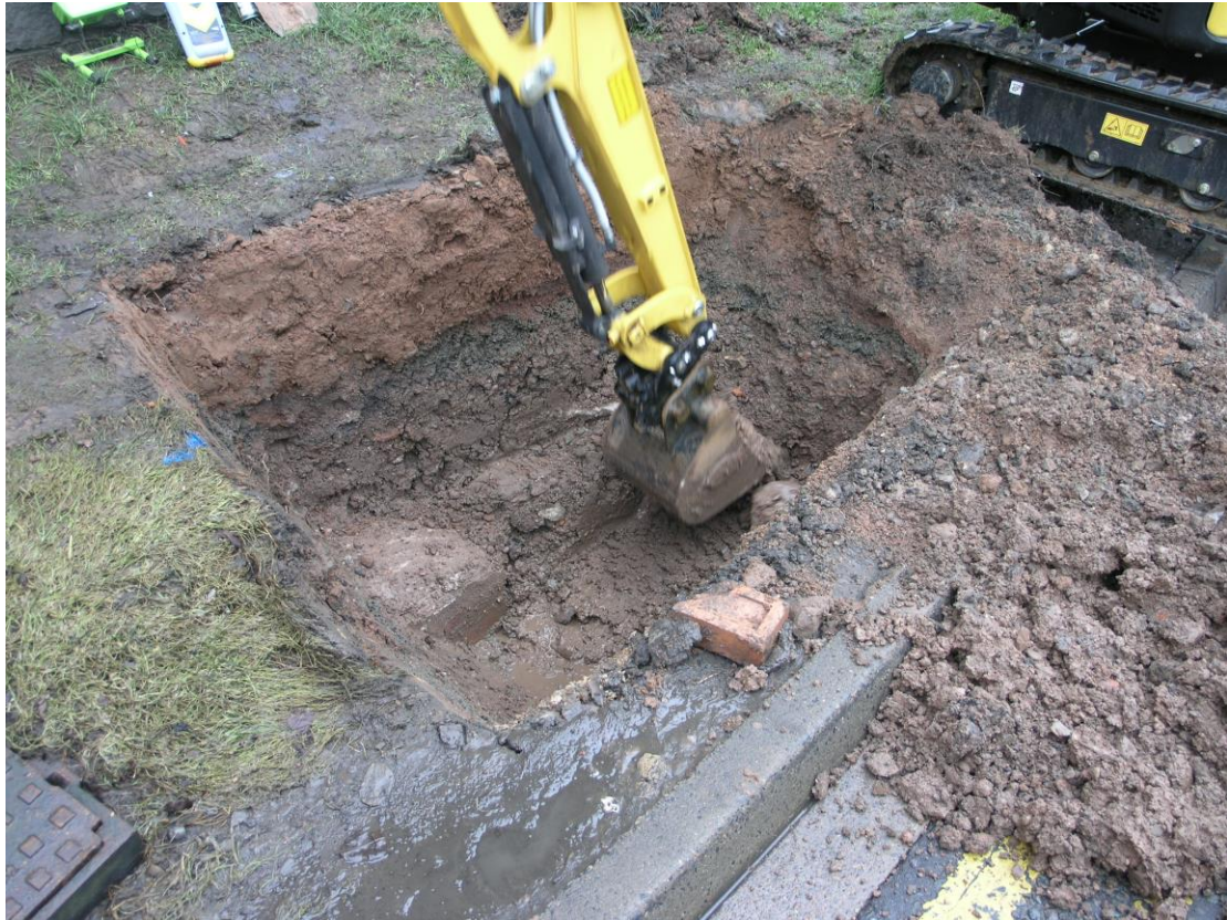
Plate 2: Trench during excavation clearly showing a top deposit of red sand associated with the construction of the wall.
