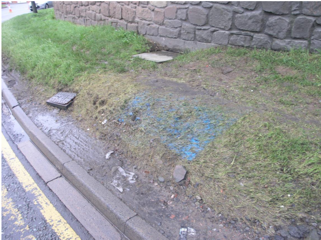
Plate 1: Location of pipe leak (blue marker paint) within the verge and in relation to other services.
