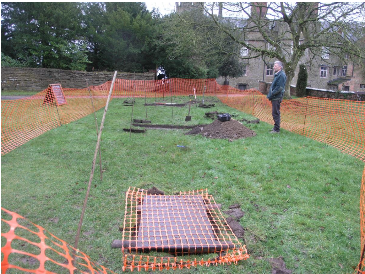
Plate 3: Line of trench / path looking south showing the drain inspection lid in the foreground.
