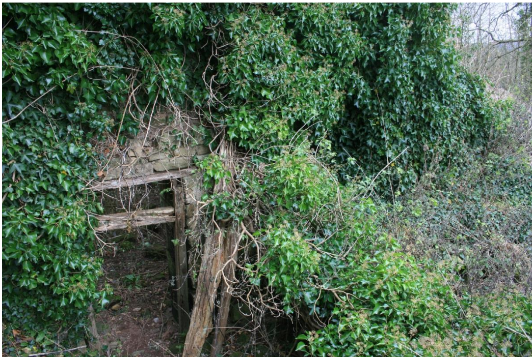
The east wall (interior), looking east over current doorway; the darker green ivy, top right, conceals a 17 th -century fireplace, condition unknown
