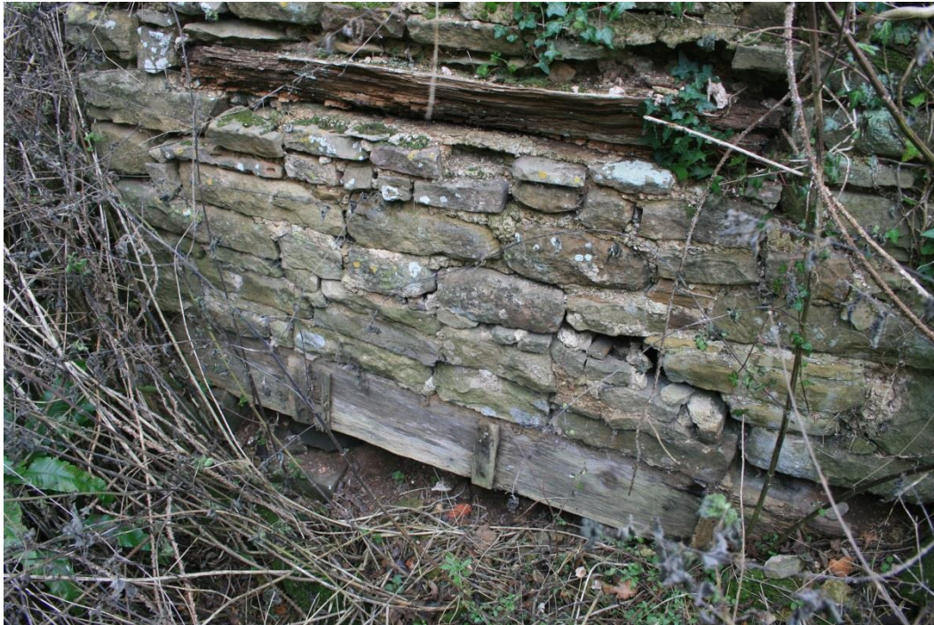
South gable wall interior: fireplace opening at base of stack. Note condition of masonry
