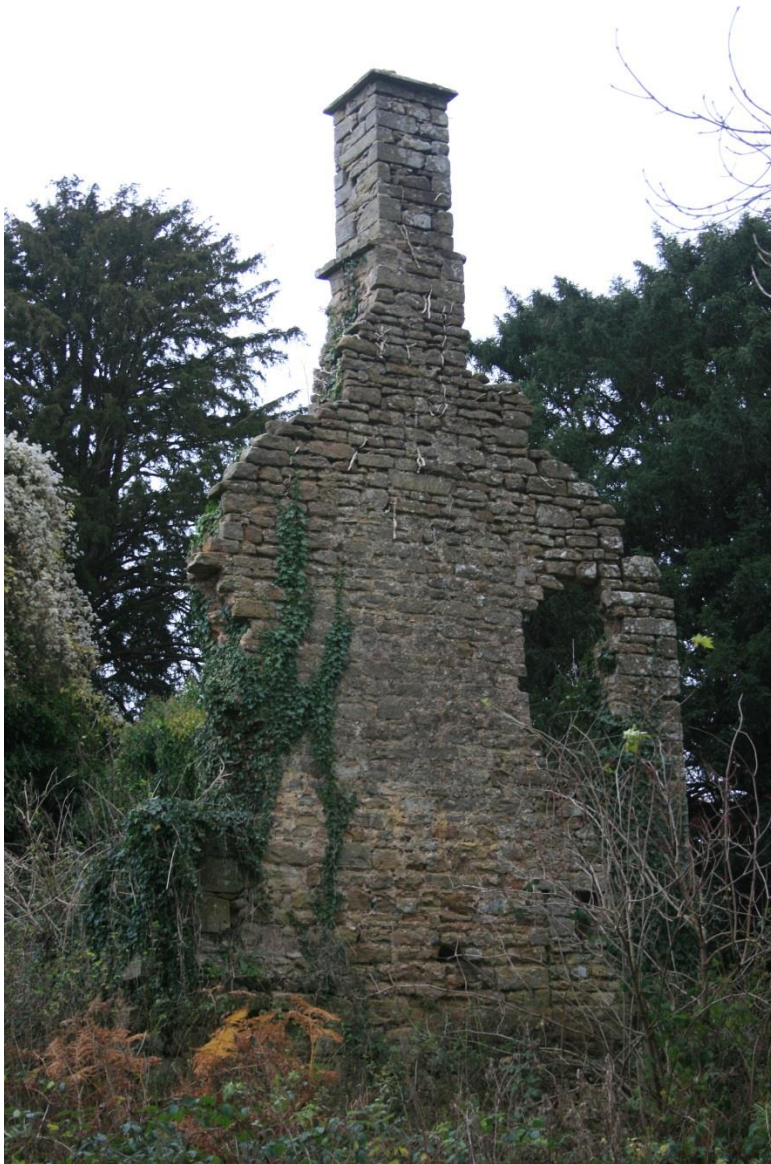
The south gable wall (external). Note state of masonry above opening, upper right
