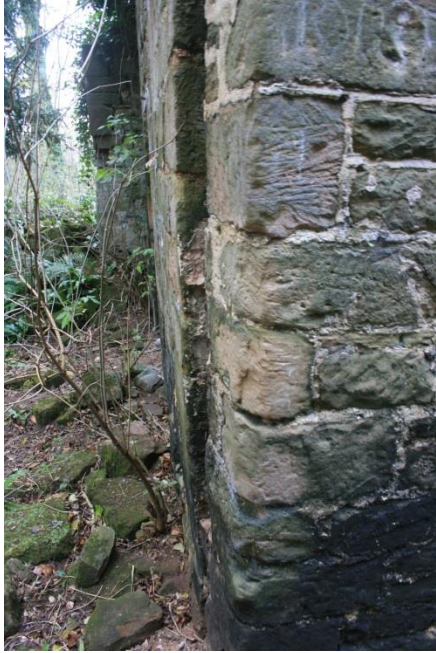
The north east corner, looking south. The long east wall is moving outwards and separating from the gable end wall at the straight butt joint
