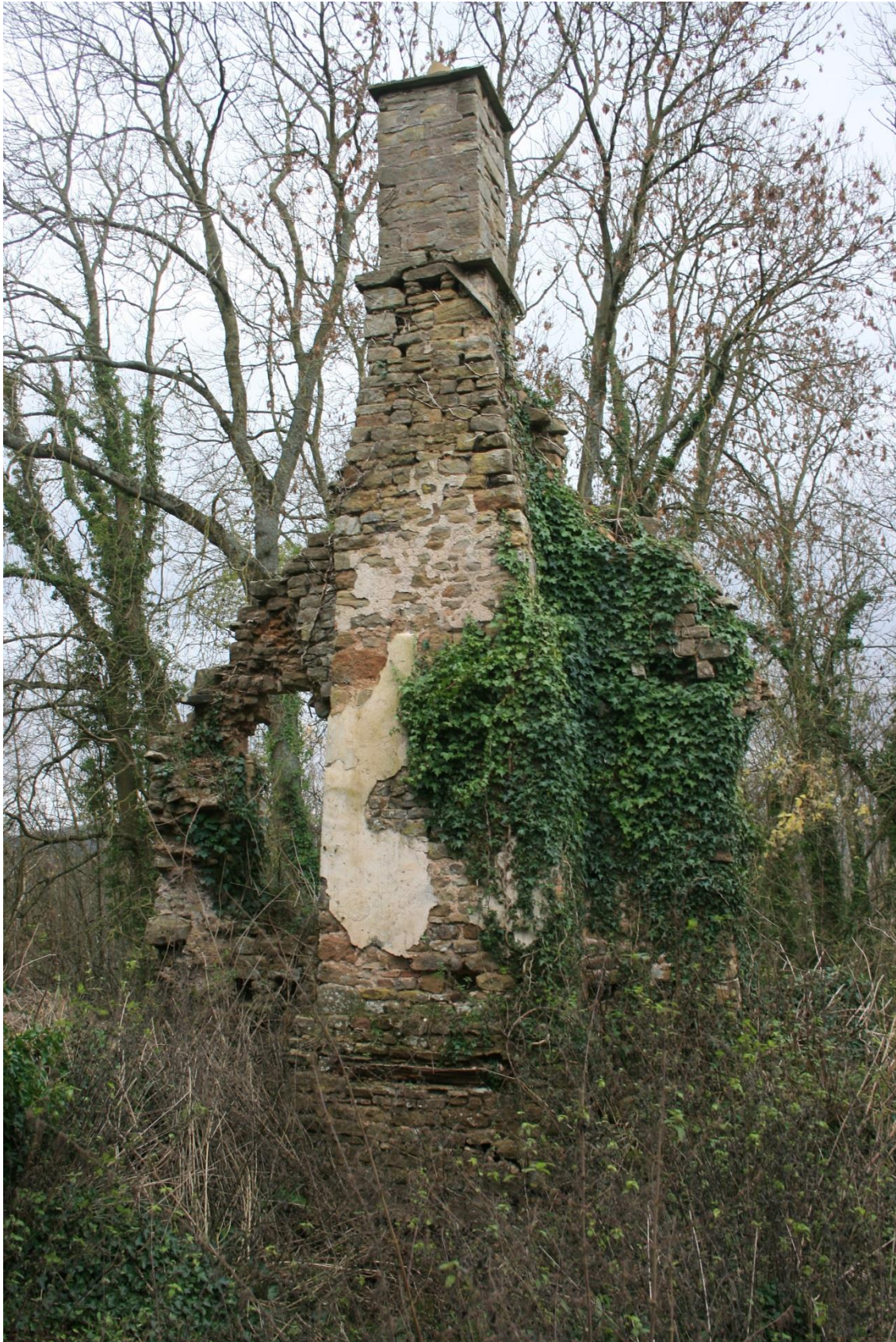
South gable wall interior. Note condition of masonry, particularly above the opening top left. Also note steepness of roof pitch and joist holes for roof and upper floor timbers
