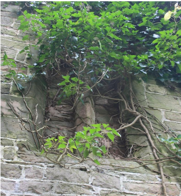
The north gable end wall (exterior) showing the medieval window (blocked) in the apex. Note strip pointing
