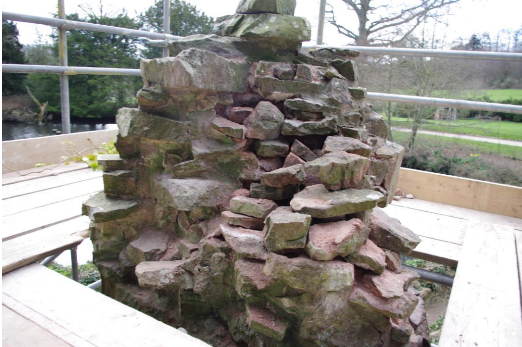
Plate 6: View of the top of the gatehouse tower as seen from the northeast.
