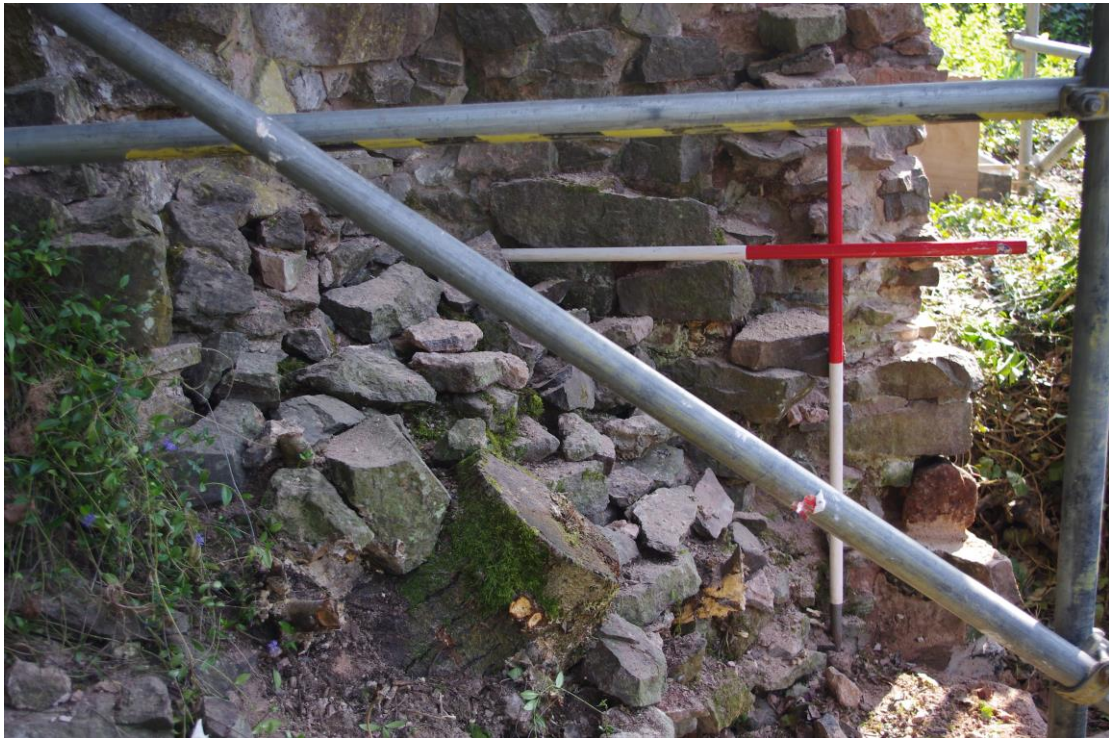
Plate 14: View of the gatehouse tower core work from the northwest, before Consolidation.
