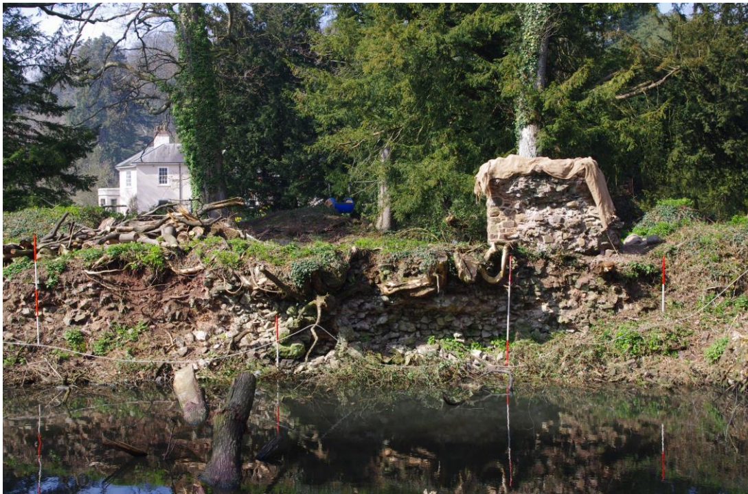
Plate 32: View of the Stair tower after initial clearance as seen from the east.
