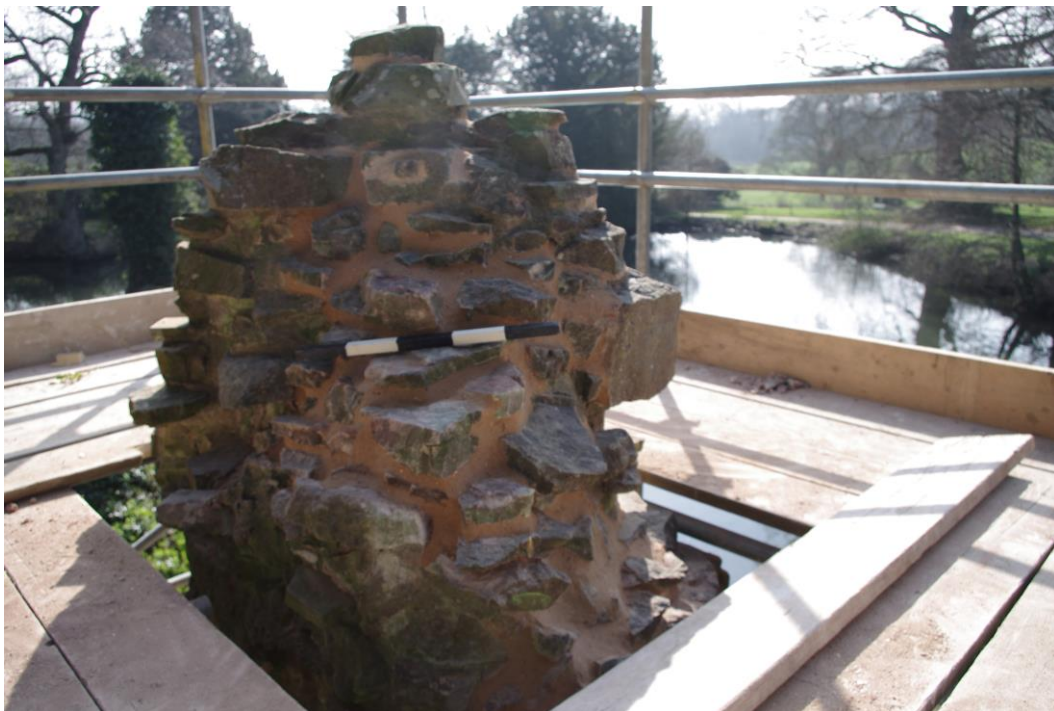
Plate 7: View of the top of the gatehouse tower from the northeast after re-pointing.
