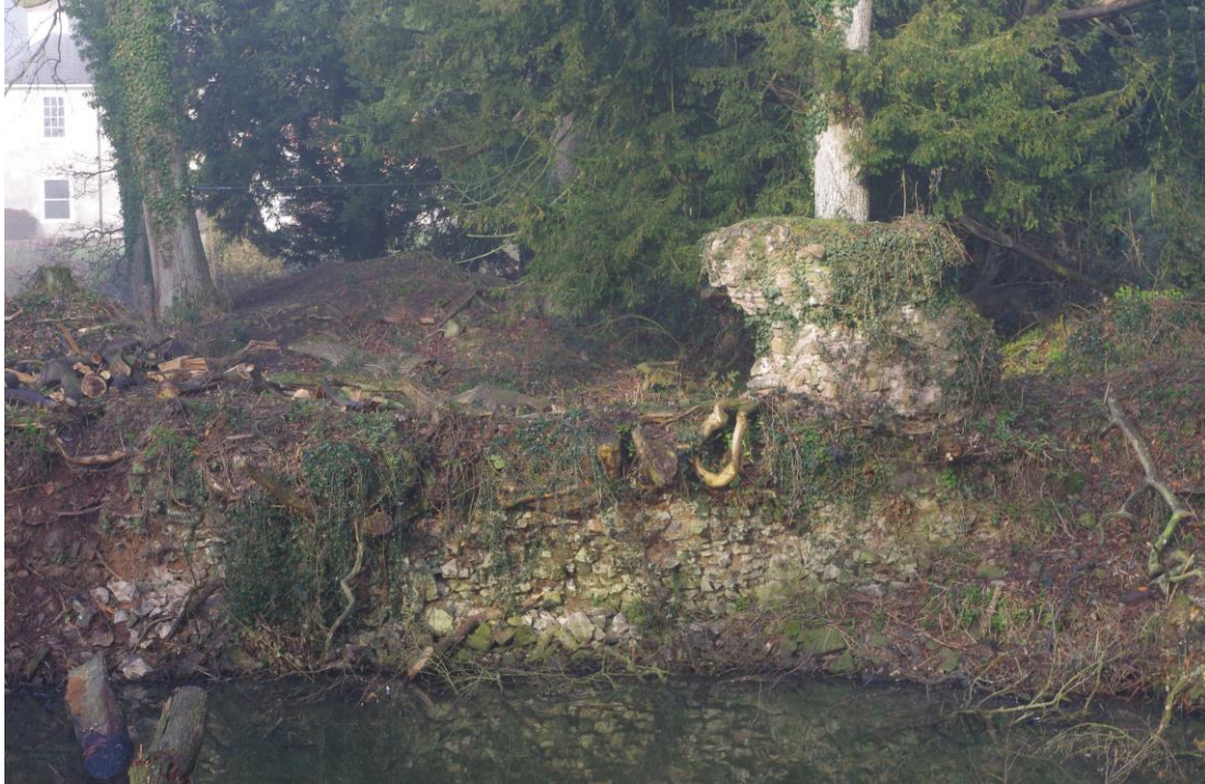
Plate 31: View of the Stair Tower and the eroding curtain wall as viewed from the east before work began.
