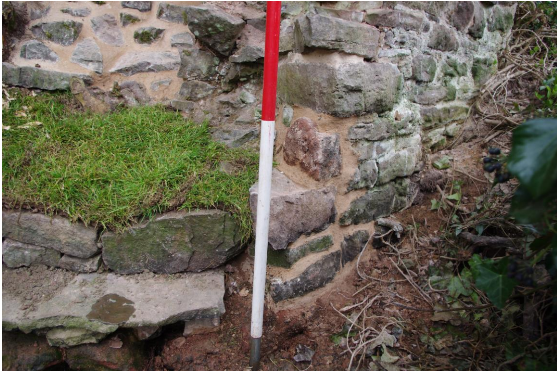
Plate 4: Re-pointed section at the base of the Gatehouse tower as seen from the west.
