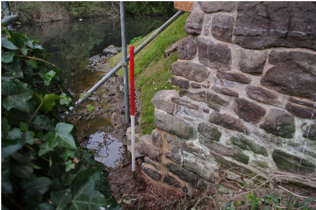
Plate 5: Re-pointed section at the base of the gatehouse as seen from the South.
