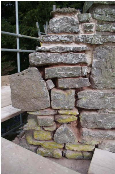
Plate 8: Upper portion of the raked out section above the moulding as viewed from the southwest.
