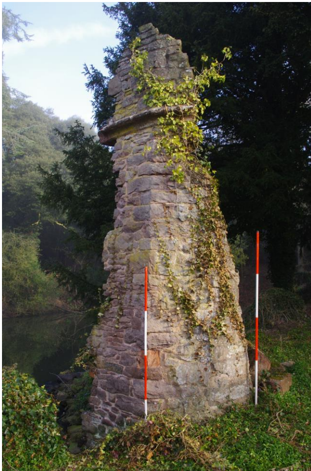
Plate 3: The gatehouse tower as seen from the southeast. Continued erosion of the earth around the base is clearly visible (bottom left).
