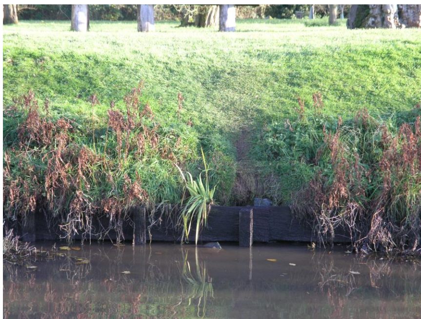
Plate 7: Timber revetting showing under-cutting and scaring due to water-fowl.
