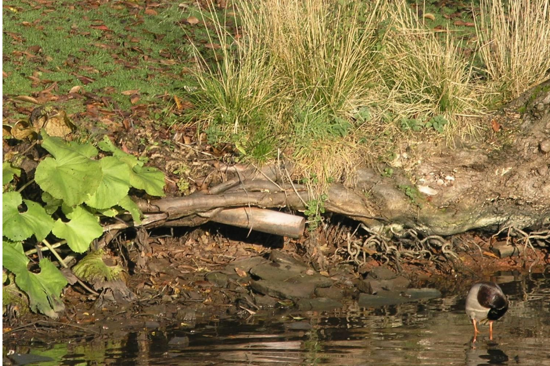
Plate 1: Plastic pipe laid in 1993 showing amount of erosion and undercutting over the last 20 years.
