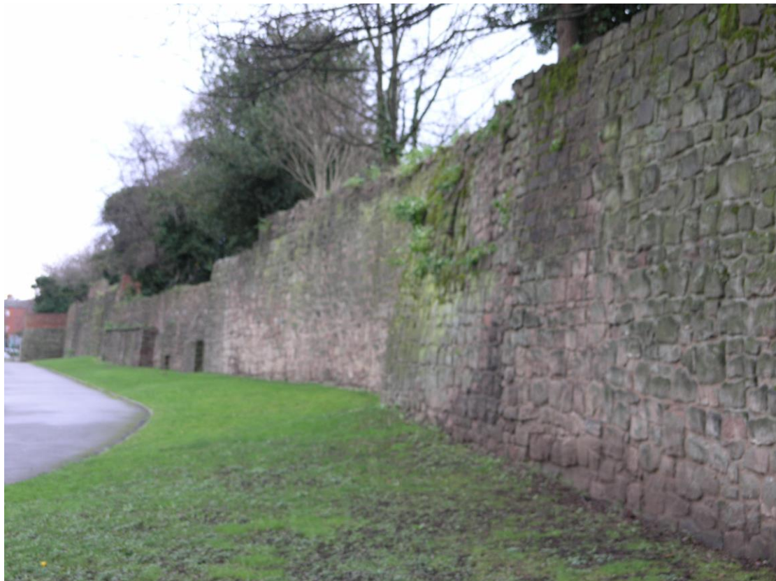
The same view in 2008. Apart from the absence of the brickwork features seen above, the extent of the 1968-9 reconstruction work is not obvious
