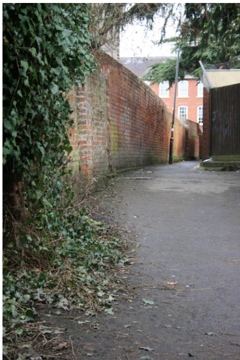
Levels dropping into the infilled ditch of the Bishop's Meadow Row Ditch to the north of Drybridge House at the rear of the St Martin's Street plots
