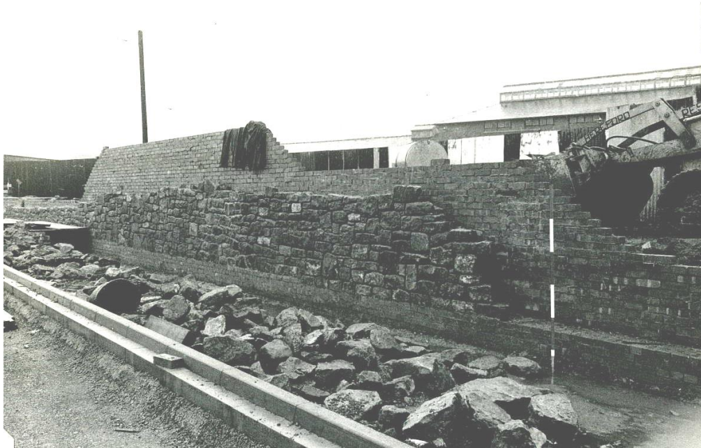
The first replacement wall under construction in October 1968, looking north-east across the site of the 1968 Brewery site excavation trench
