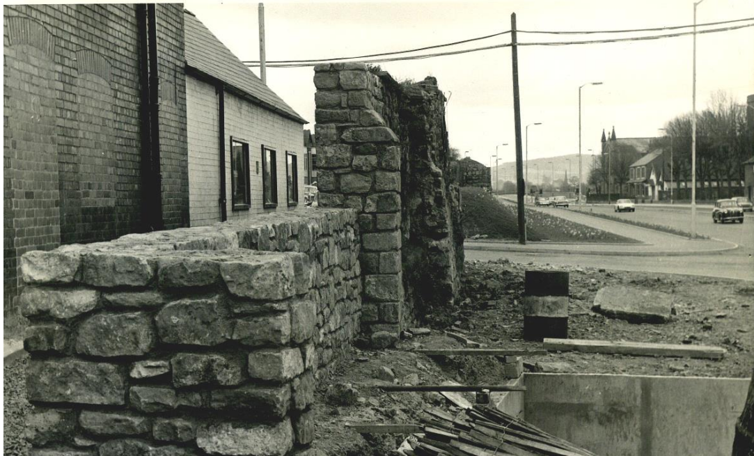
The north end of the Gunners Lane wall in April 1969 after reconstruction. Other photographs show the stones of the buttress (mid-foreground) numbered for dismantling (Contract photographs file, Hereford City Council)
