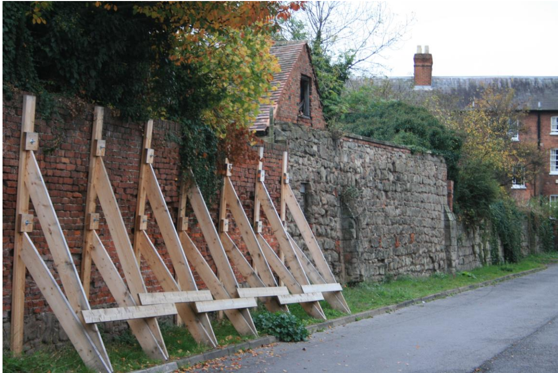
The failed brickwork stretch of wall immediately north of the Black Lion plot, prior to repairs
