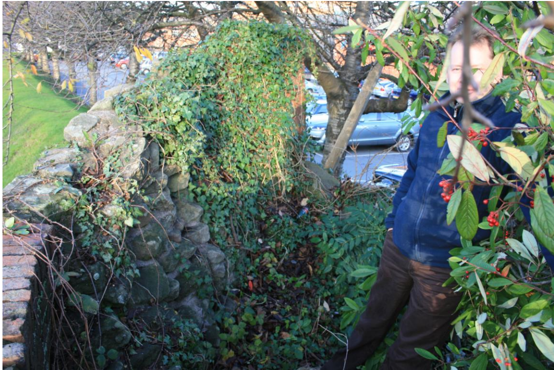
Bastion 4 interior, looking north at rampart-top level. The figure in the foreground is parting the undergrowth to allow a clearer view
