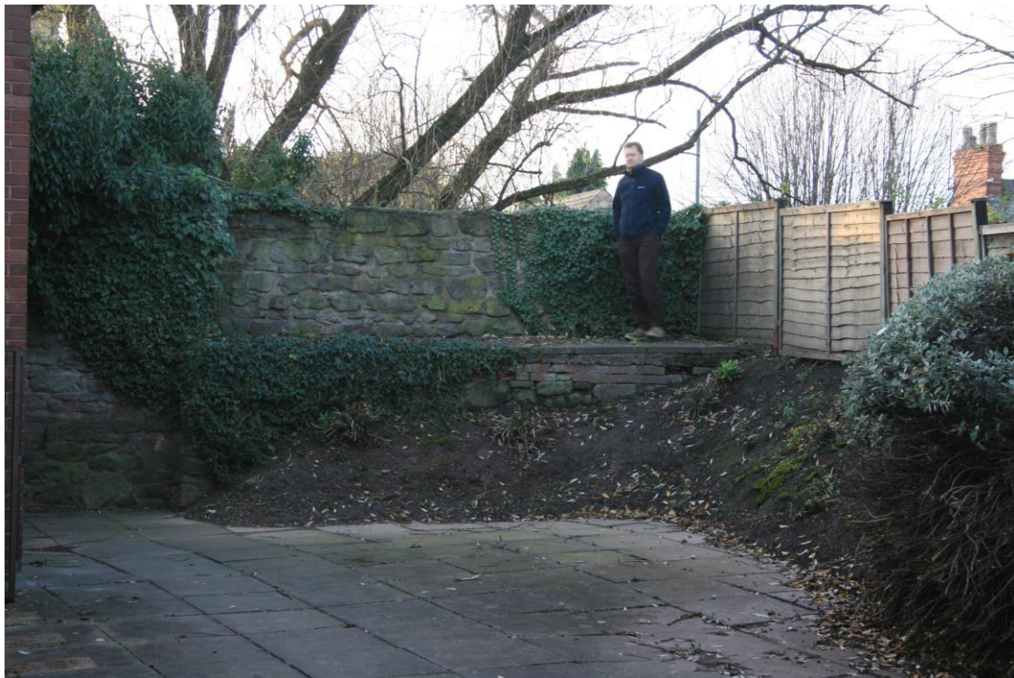
Interior at rampart level behind offices/houses on St Nicholas Street. This is the area of the collapsed section north of the sub-station, seen above in 1968
