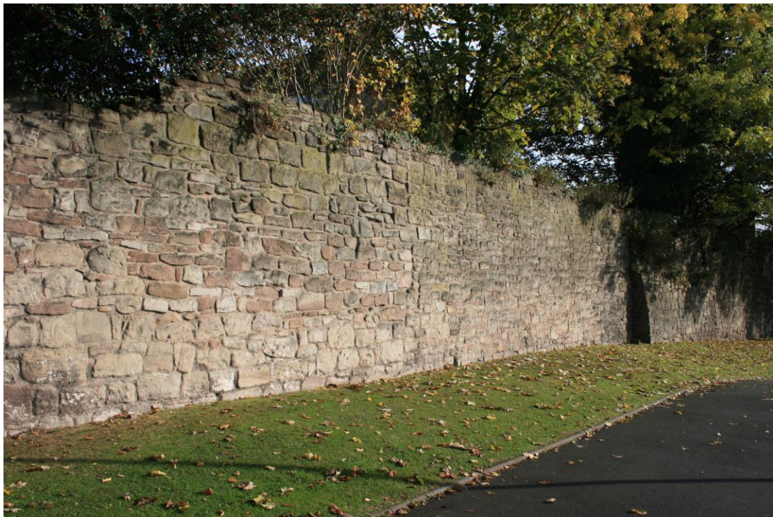
Different builds in the masonry of section 3 on the exterior face of the Berrington Street Job Centre stretch
