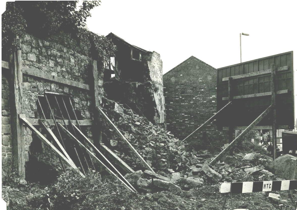
The south end of section 3 looking south. Photograph of September 1968 showing collapses immediately north of the electricity sub-station (Hereford City Council contract photographs file)
