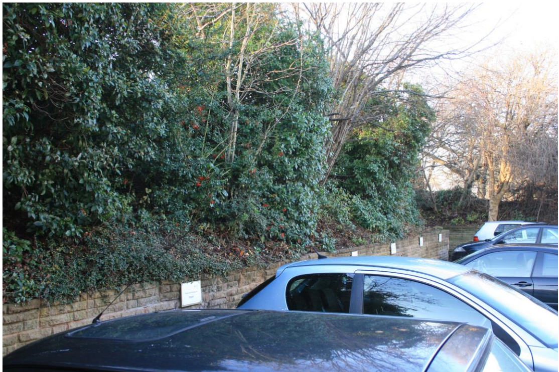
Interior face of the rampart on the Kemble Housing Association plot, looking north towards Bastion 4. The wall parapet is concealed by the dense undergrowth
