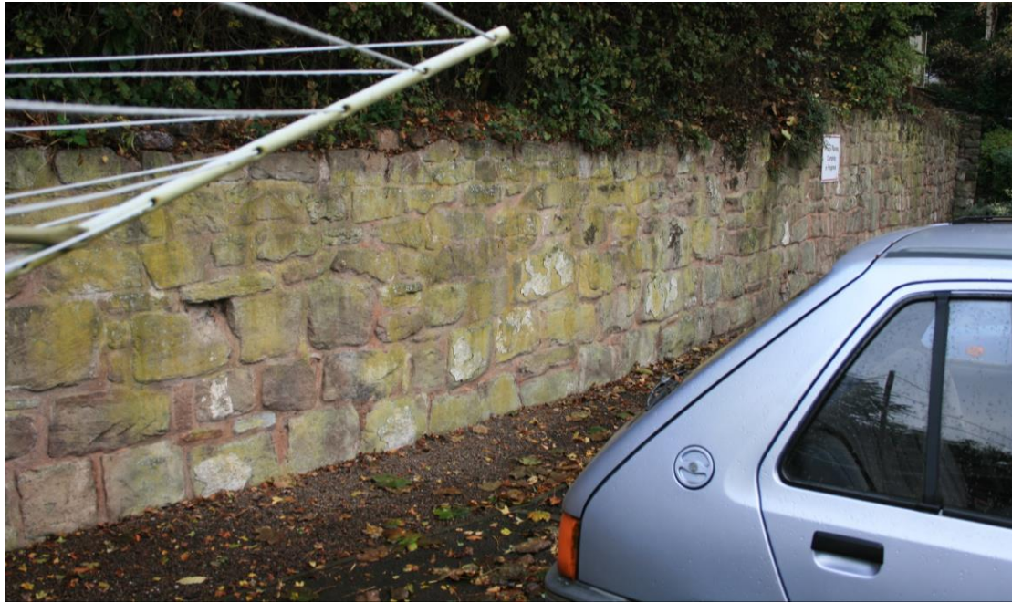
The wall, retaining the higher ground of the pre-Conquest ramparts, to the south of the Cantilupe Street excavation site
