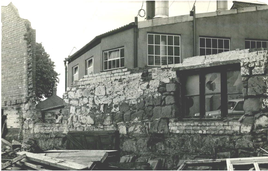
A stretch of the Wall Street wall, with the characteristics of primary city wall masonry, newly exposed by the demolition of buildings on the south side of New Market Street in August 1968 (City Council contract photographs file).
