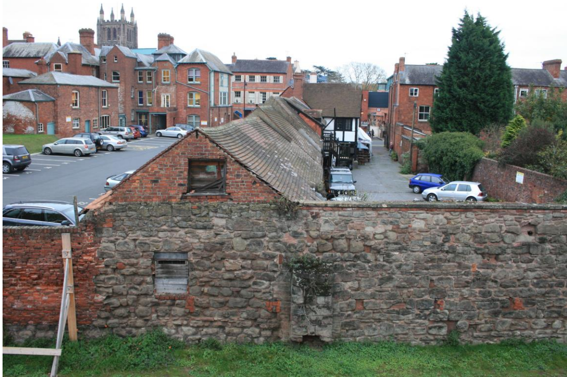
The section 1 wall at the rear of the Black Lion pub on Bridge Street
