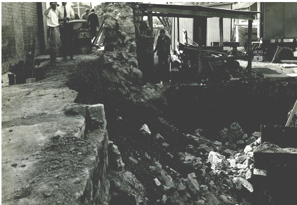
The north end of the Gunners Lane wall in 1968 following the collapse of masonry into the underpass excavations alongside (Contract photographs file, Hereford City Council)
