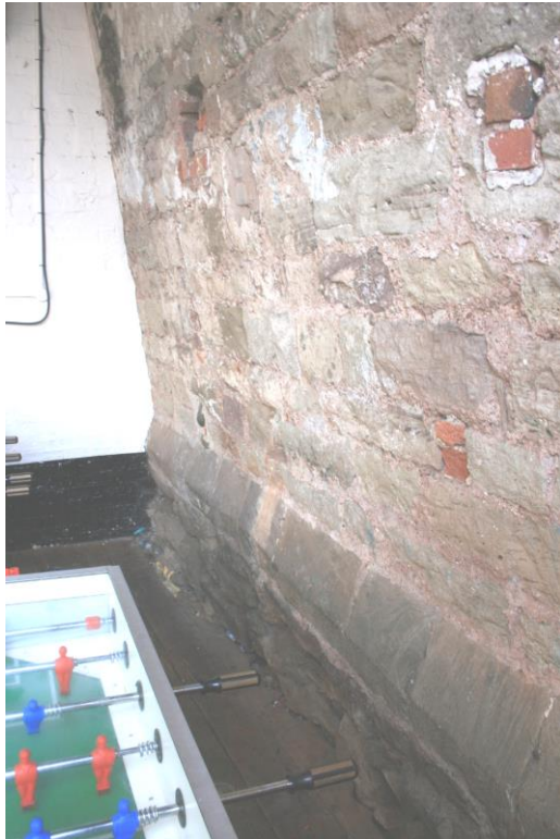
Detail of the wall in the Barrels, showing the extreme outward lean and the chamfered ashlar plinth with foundation courses below
