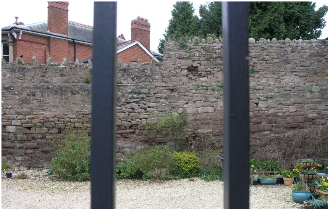
The wall in the garden of 14 Mill Street. The offset ledge marks the transition from the retaining wall to the garden wall on top. The condition of the wall in terms of missing and eroded stones, voids and lack of pointing is evident
