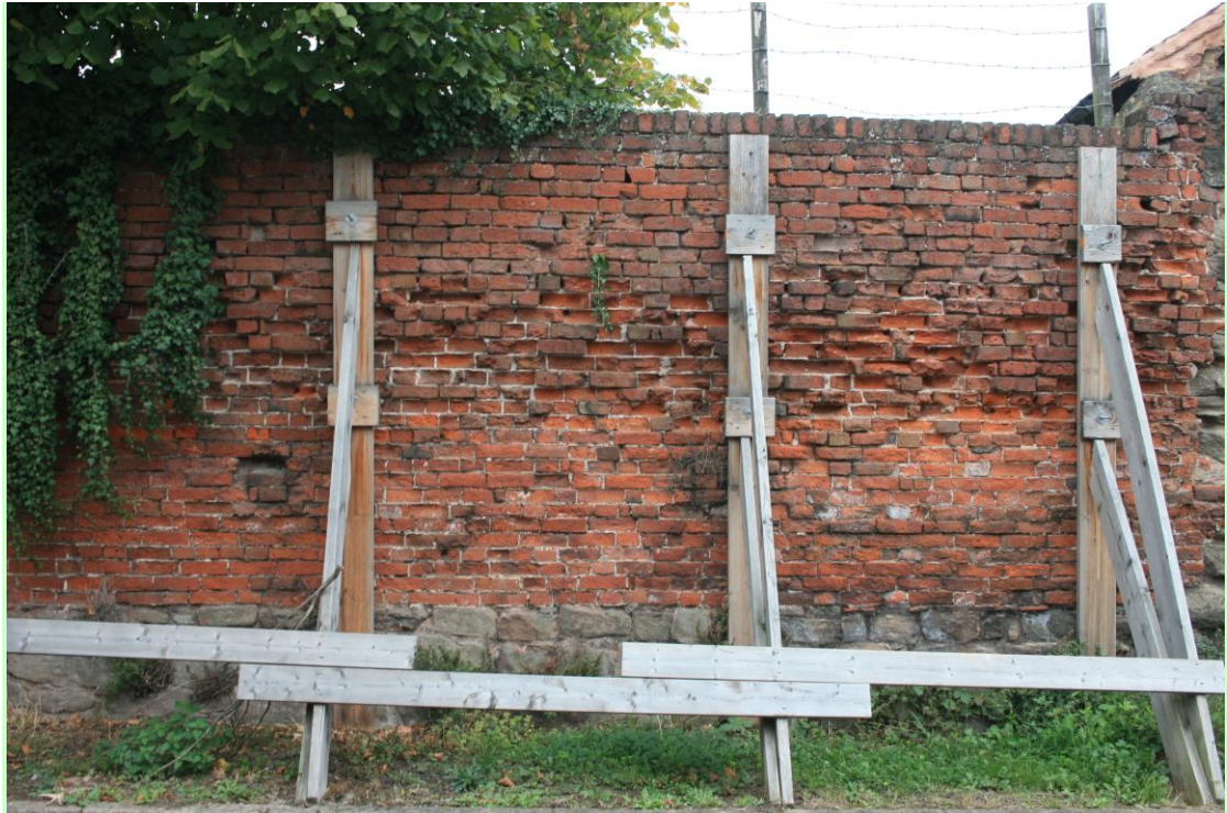
Plate 2: The central stretch of the propped brickwork with the city wall fabric reduced to two or three courses. The weathering of the brickwork approximately mid-height is particularly noticeable here
