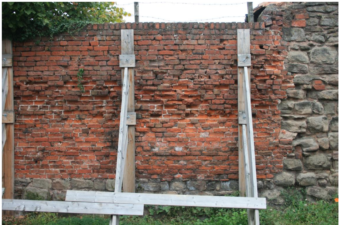
Plate 3: The southern end of the propped section showing its junction with the Black Lion outbuilding. Trench 2 lies behind the brickwork here
