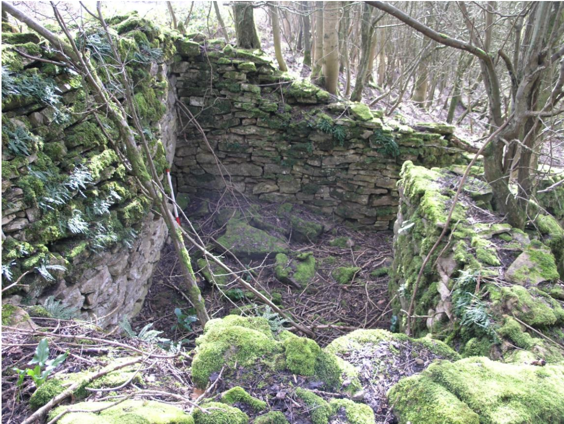
Plate 2: The Hermitage looking east showing the bowing north wall and angle of pent roof.
