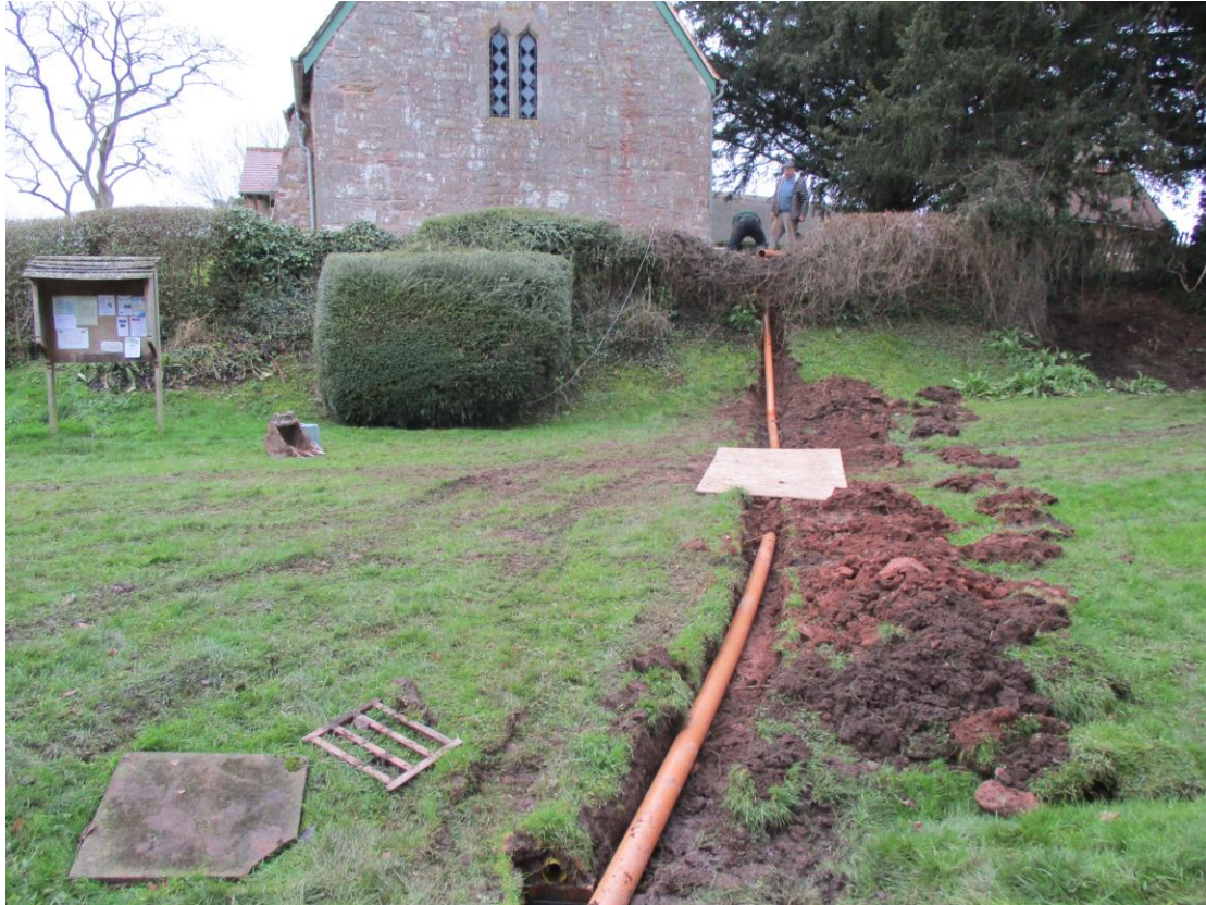
Plate 6: Drainage run from the north east corner of the church looking west from the junction into the existing drain. The old pipes from the old drain are visible at the bottom centre of the photograph.
