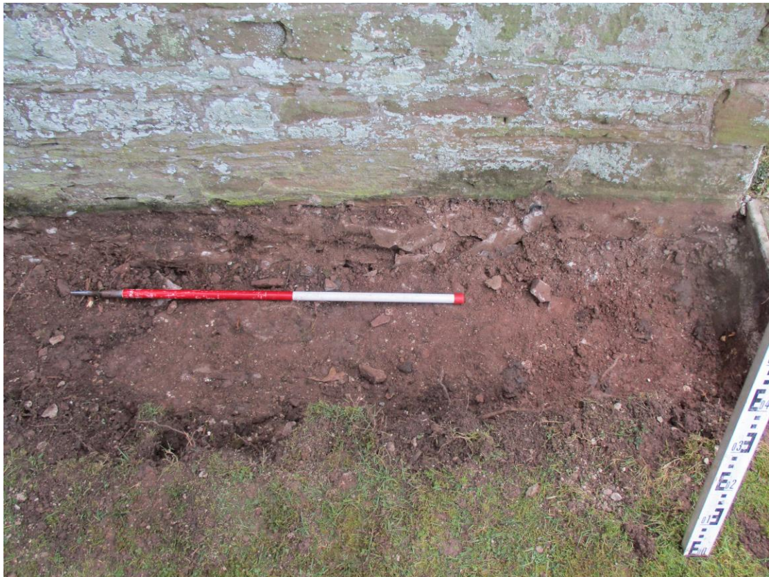
Plate 3: Detail of disturbed ground at the base of the drainage run.
