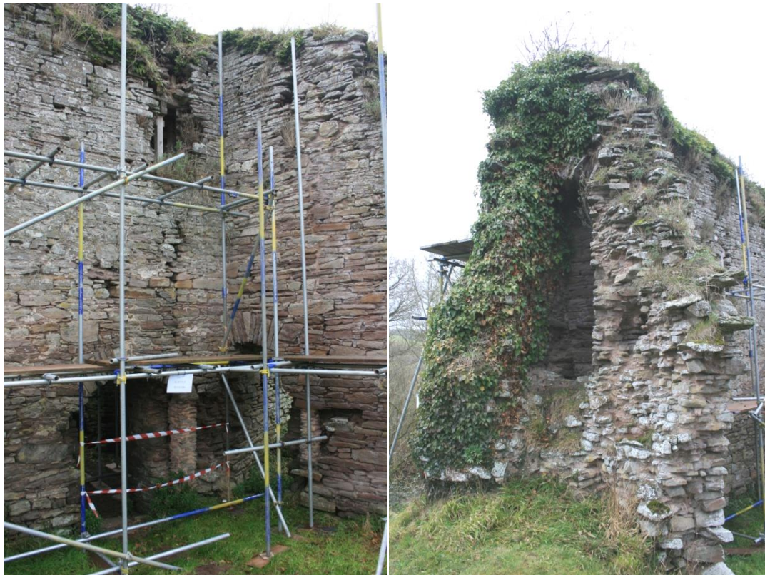
(4) Above left: junction of the curtain wall with hall south wall. (5) Above right: stub-end of wall with garderobe chamber off former SW tower
