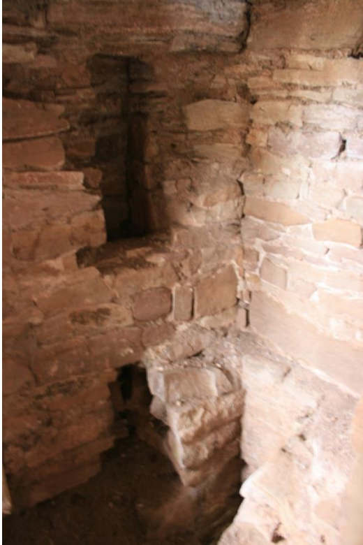
(9) Garderobe chamber in W wall, first-floor level. Looking SW at bench and opening of main chute (bottom right) with holes knocked through the south wall at two levels into incomplete garderobe chute behind
