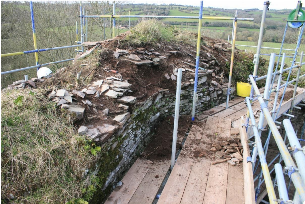
(17) West wall top, looking north, early stages of 'gardening' – removal of vegetation, root-mat, soil and displaced/loose stone
