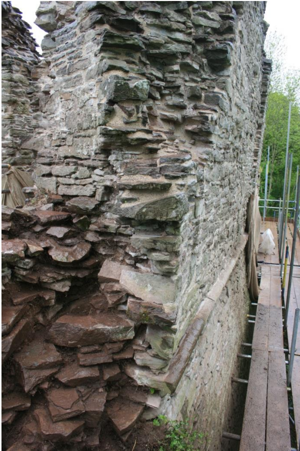
(39) North wall of the hall, external, looking west from damaged area at NE corner of chamber to east of the hall. Note string course slabs are integral to wall fabric
