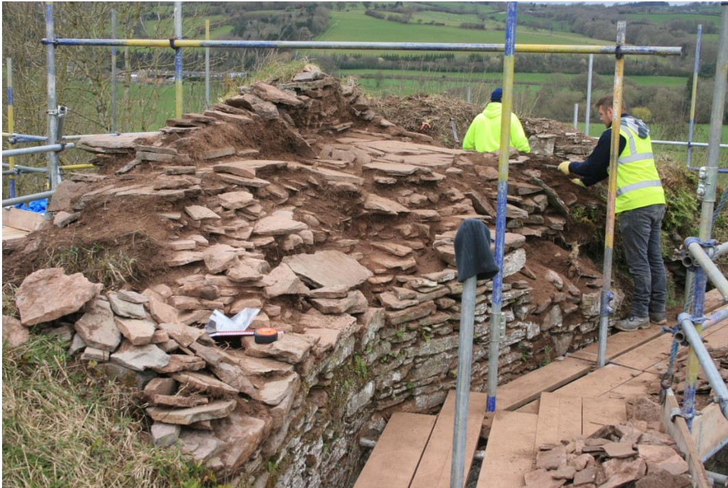
(19) West wall top looking north. The wall-walk and parapet as first revealed
