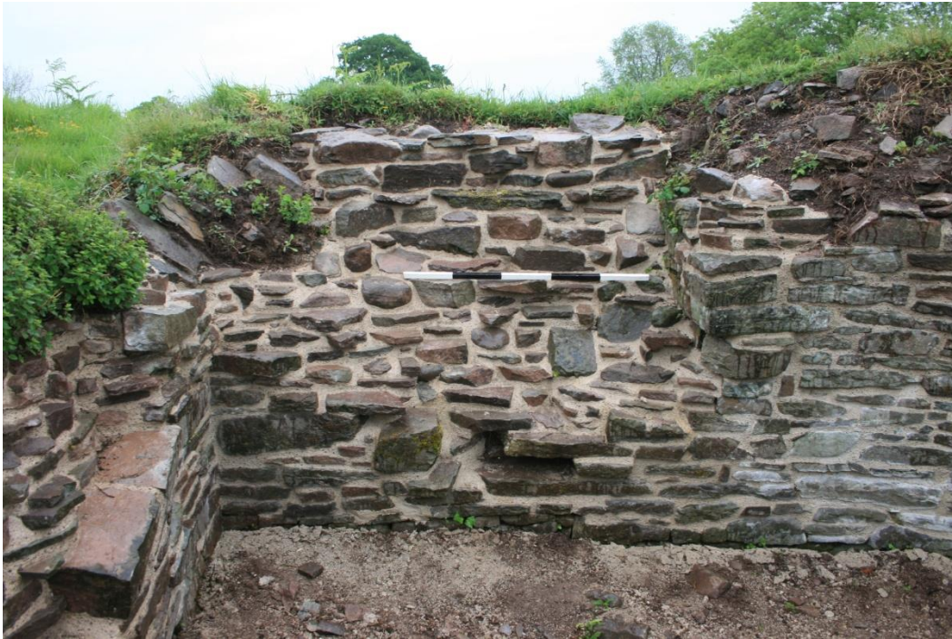
(62) North-east wall and window embrasure of SE tower at end of consolidation process, compare (59)
