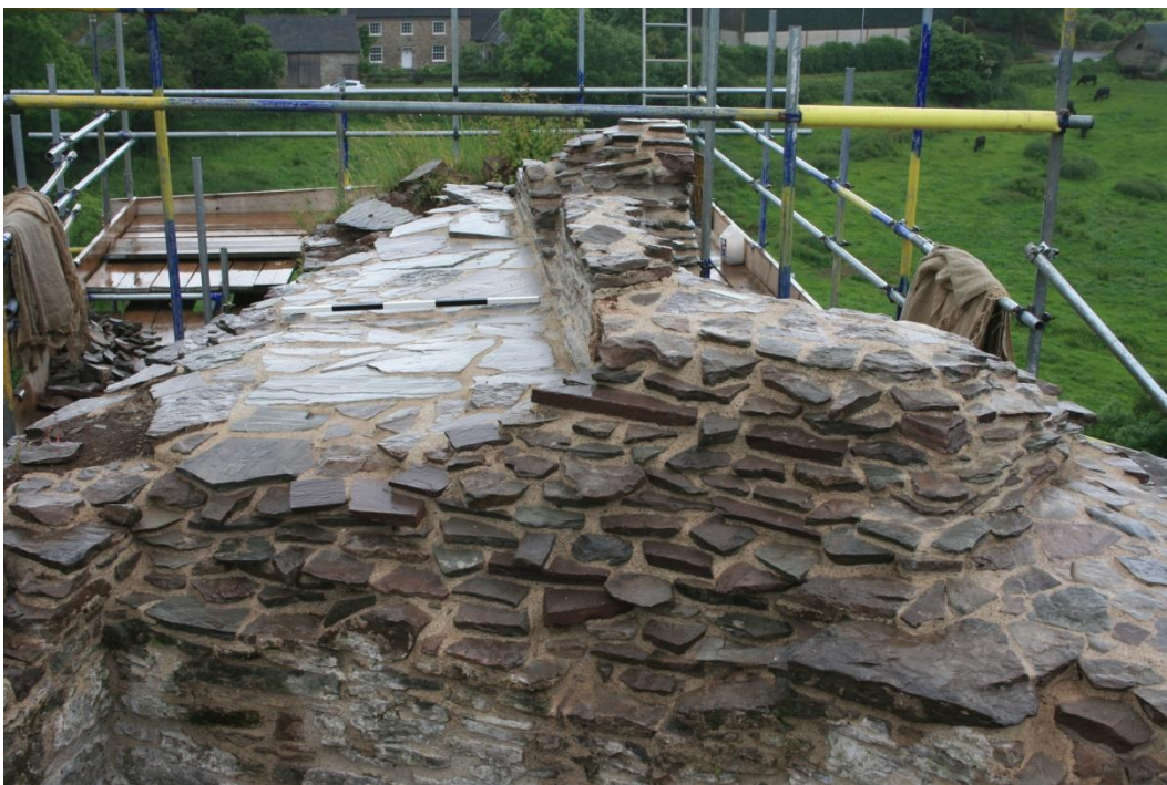
(25) West curtain wall looking south from NW tower, post-repair, as consolidated prior to soft capping
