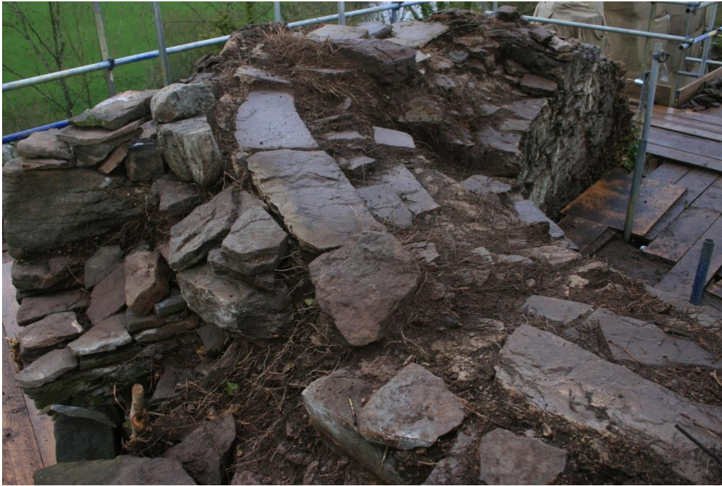
(29) NW tower wall top, NW quadrant wall walk slabs with parapet wall base course (left), as first exposed
