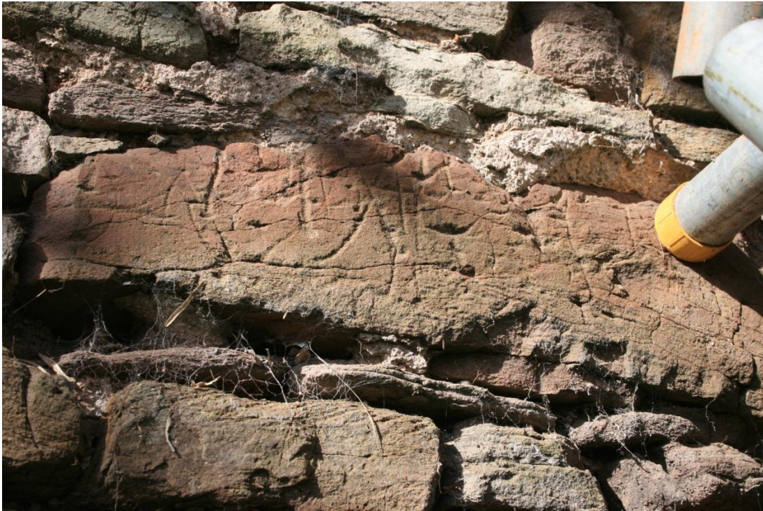
(6) West curtain wall: scratched/inscribed stone over doorway to NW tower
