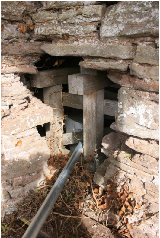
(16) West elevation: hole at first-floor level at the junction of the NW tower and main west wall face, showing propping within garderobe passage
