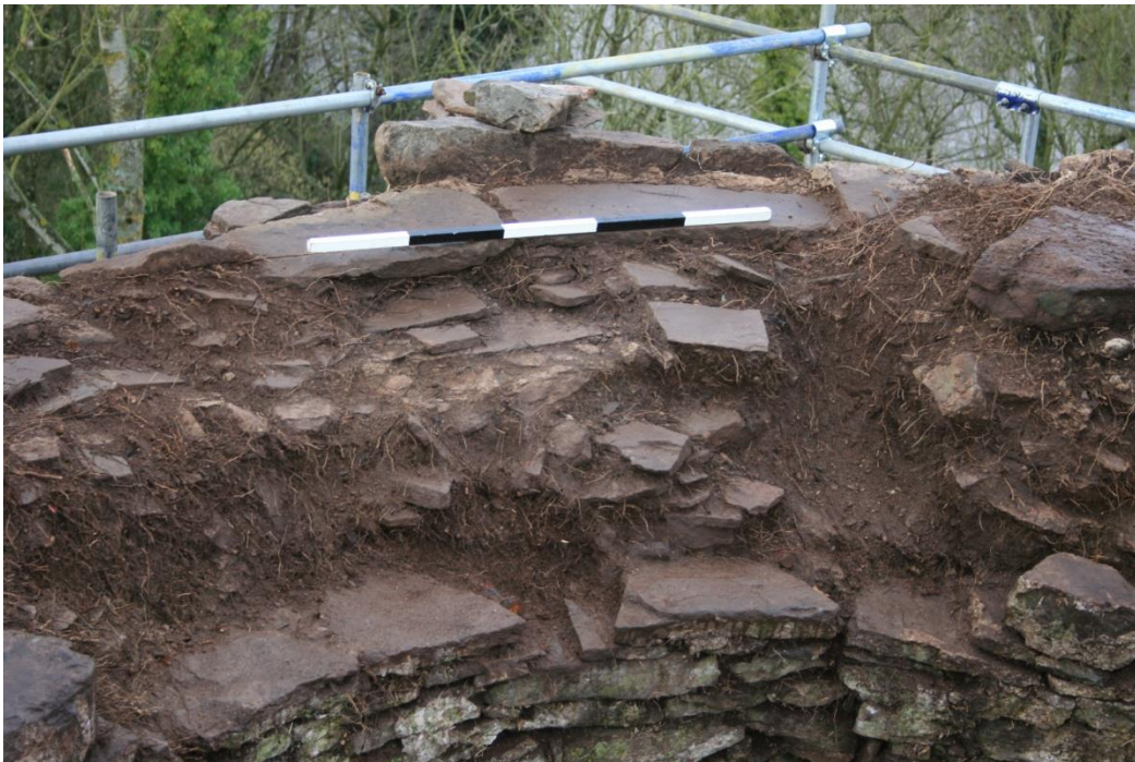
(28) NW tower wall top, NW quadrant wall walk slabs with parapet wall base course as first exposed (root mat still largely in place, foreground and right)
