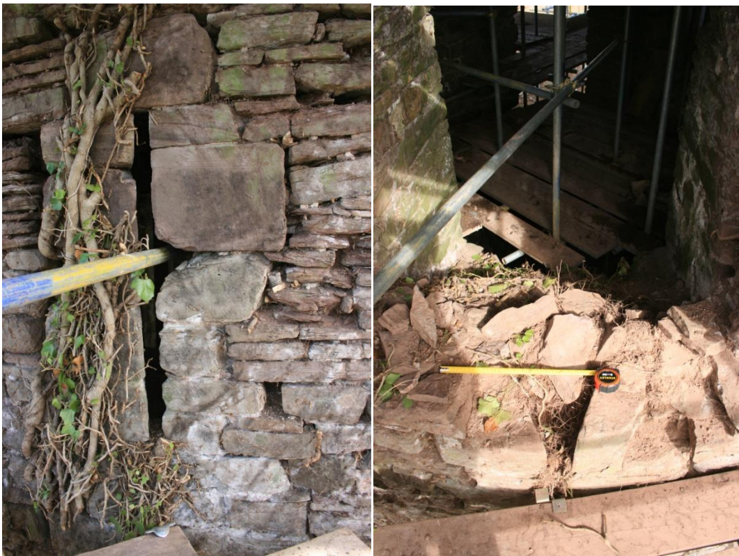
(12) Left: NW tower, first floor, loop window facing NW; (13) Right: first-floor loop window embrasure facing SW with surviving lower loop reveals
