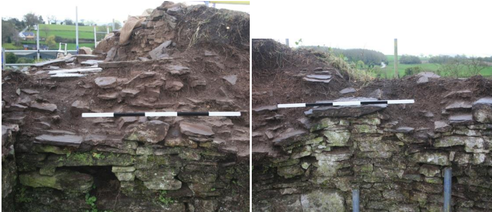
(26) NW tower wall top in final stages of gardening, S and SW sides
