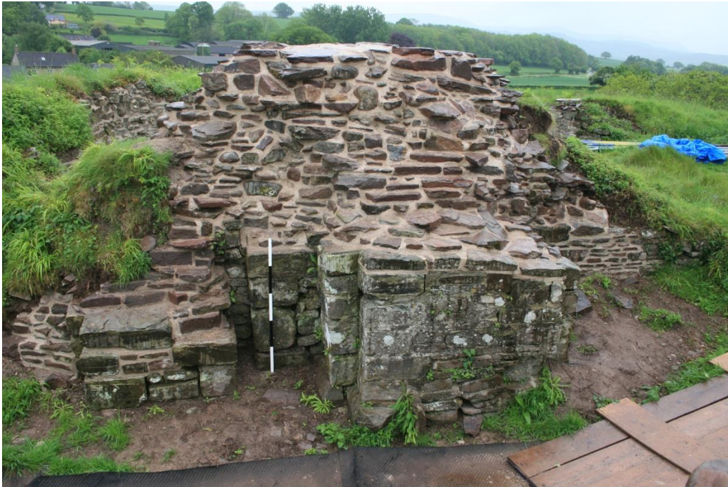
(53) Gatehouse passage, south side post-repair, portcullis slot to left of 1m scale
