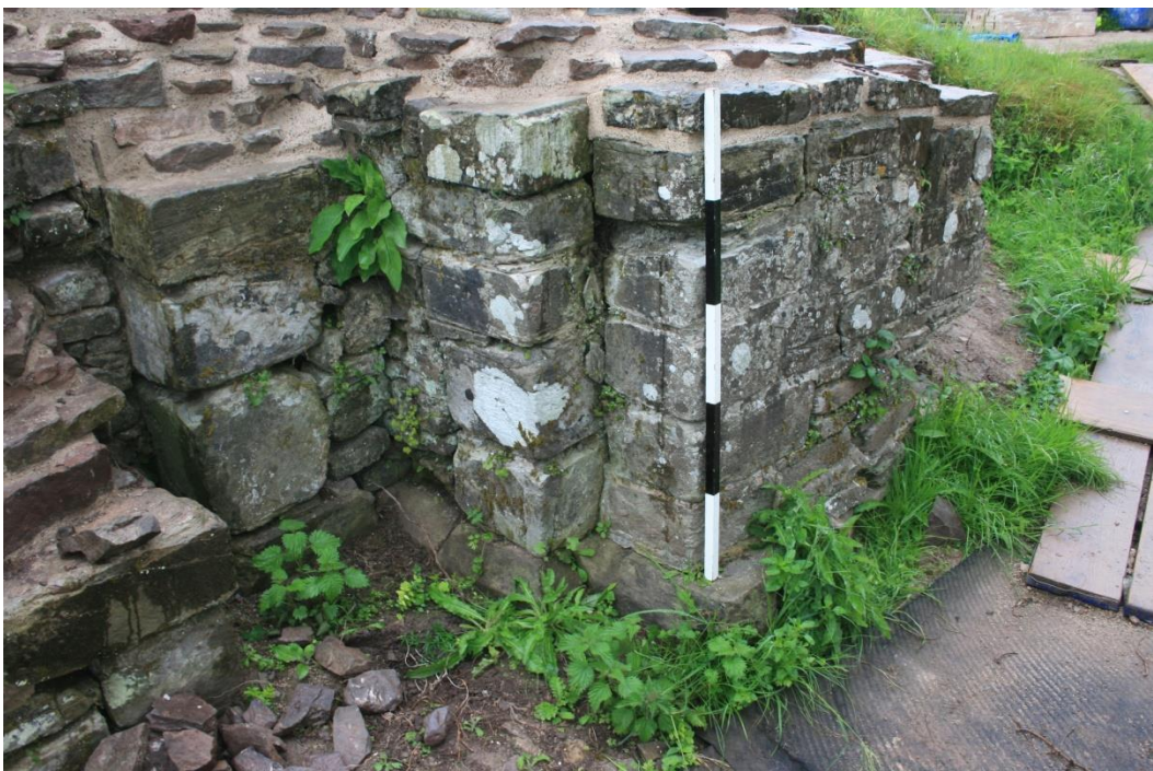
(54) Gatehouse passage, south side, inner arch detail, portcullis slot to left, post-repair
