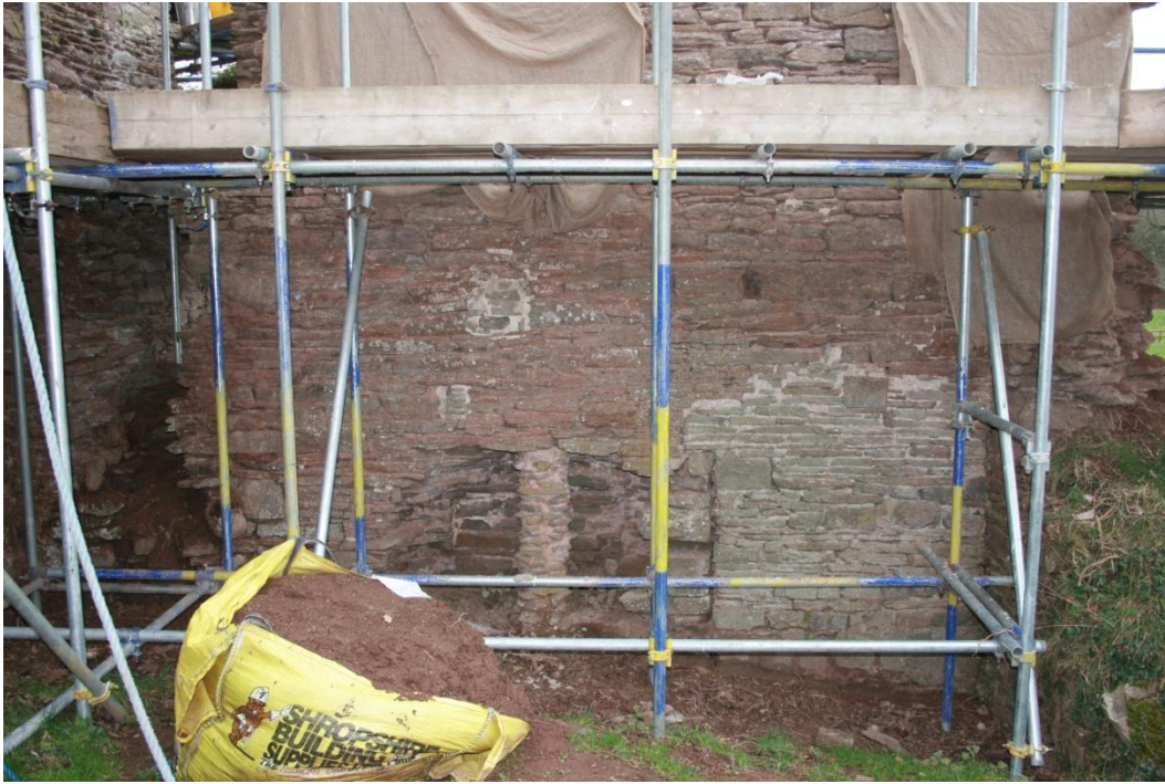
(41) E end wall of hall, internal, pre-repair showing propping in niche and blocked opening to its right
