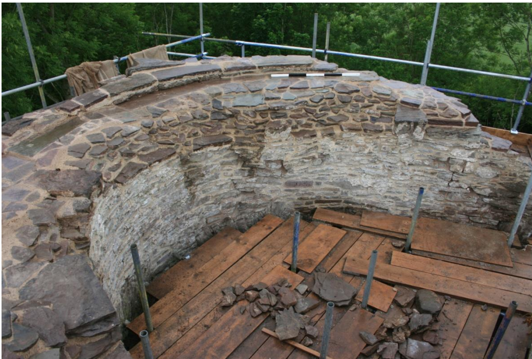
(30) The NW tower wall top, NW quadrant, after consolidation and prior to soft capping. The 1m scale lies on core-work slabs below the wall-walk slabs; very little survives of the parapet wall beyond
