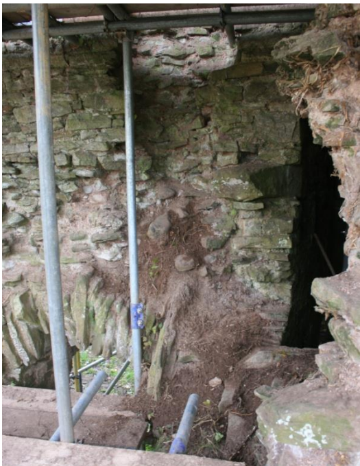
(35) S wall of hall: passage vault voussoirs (lower left) and doorway into tower (right)
